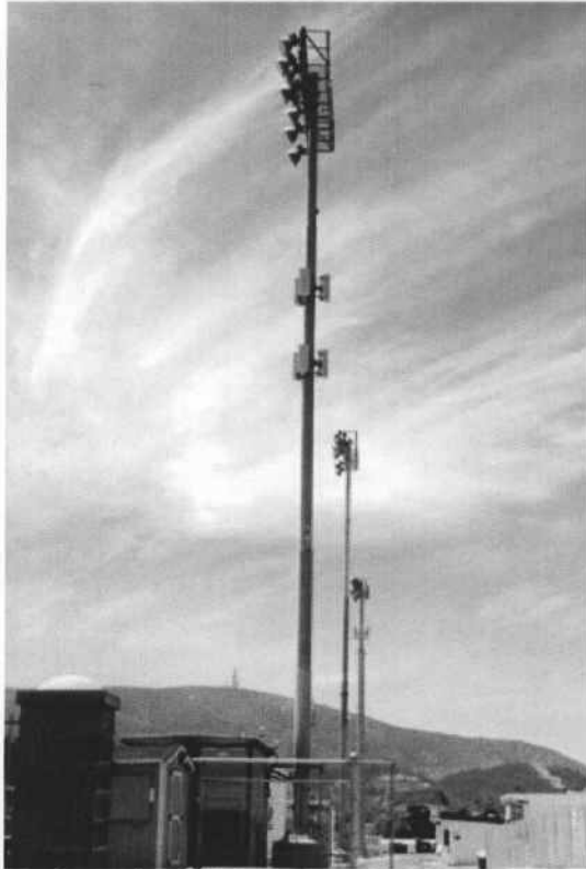
Co-location with a Stadium light
