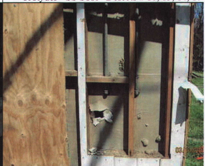
R Ryder - SS STR - Defects # 10, 12, 13, 14, 1
