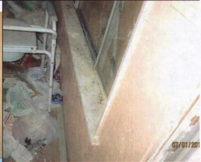
M Sanders 070110 - broken windows and water damage
