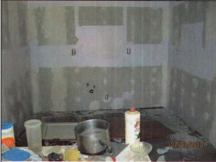
M Sanders 070110 - missing kitchen sink and lighting fixture
