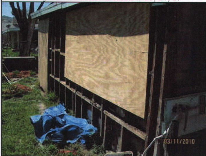
R Ryder - SS STR - Defects # 10, 13, 14, 17
