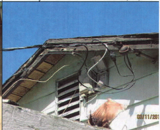
R Ryder - SS STR - Defects # 6, 14, 17
