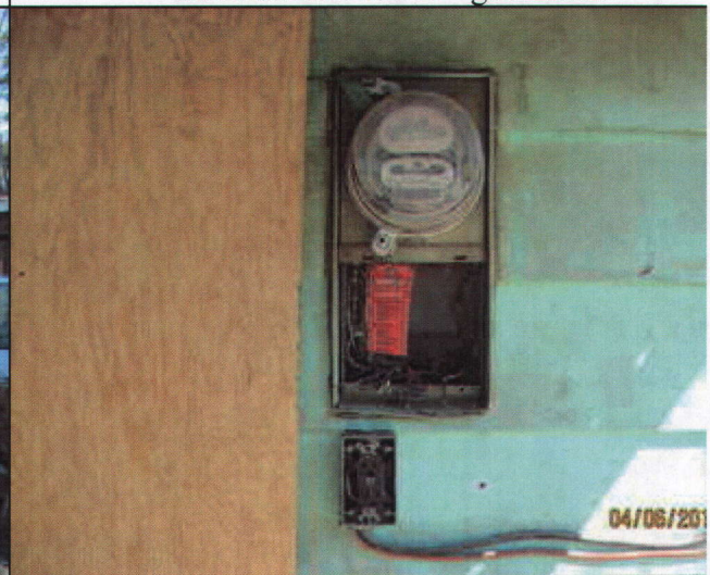
M Sanders 040610 - sub standard electrical pan
