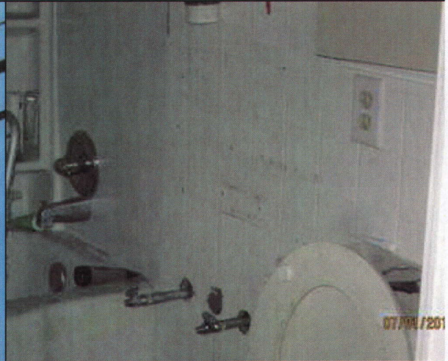
M Sanders 070110 - missing bathroom sink
