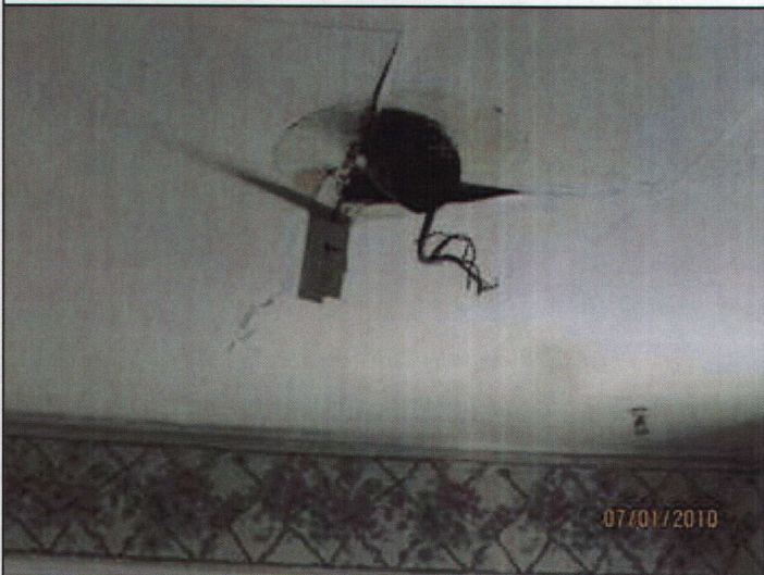
M Sanders 070110 - missing lighting fixture and exposed electrical wiring
