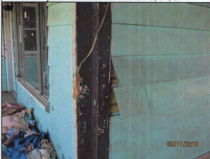
R Ryder - SS STR - Defects # 10, 14, 17
