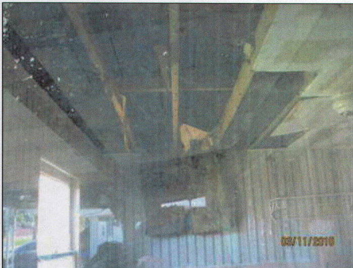
R Ryder - SS STR - Defects # 11, 12, 14, 17
