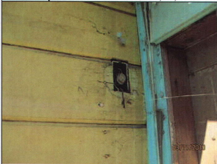
R Ryder - SS STR - Defects # 6, 14, 17
