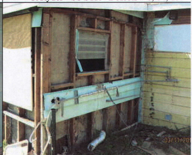
R Ryder - SS STR - Defects # 10, 13, 14, 17
