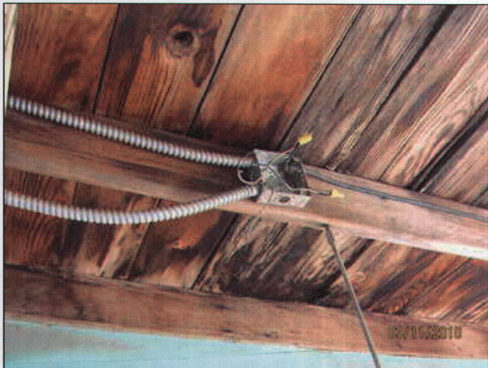
R Ryder - SS STR - Defects # 6, 14, 17
