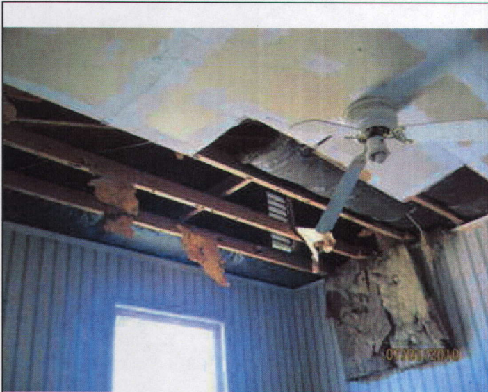
M Sanders 070110 - missing ceiling
