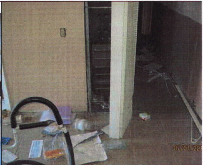
M Sanders 070110 - heater, thermostat missing from wall
