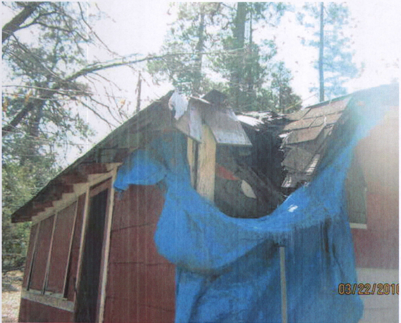
CForrey / Defect #10, 11, 12 Open, damaged roof and walls - 03/22/2010
