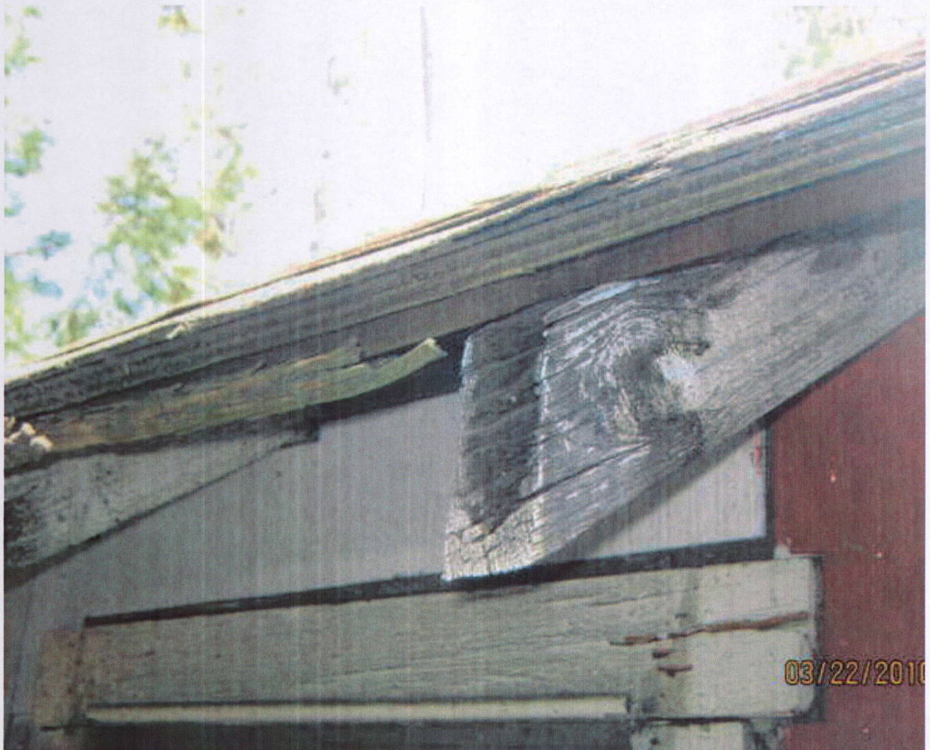
CForrey / Defect #14, no mainenance, eaves deteriorated - 03/22/2010
