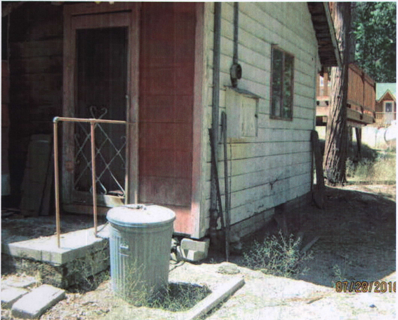
CForrey / Foundation has not been repaired - 07/28/2010
