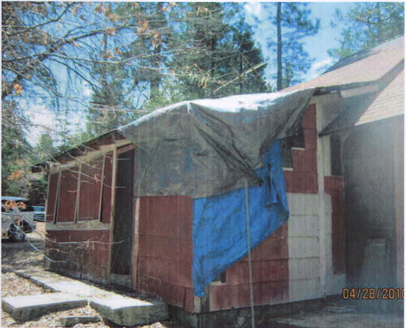
CForrey / Tarp over damaged area - 04/28/2010
