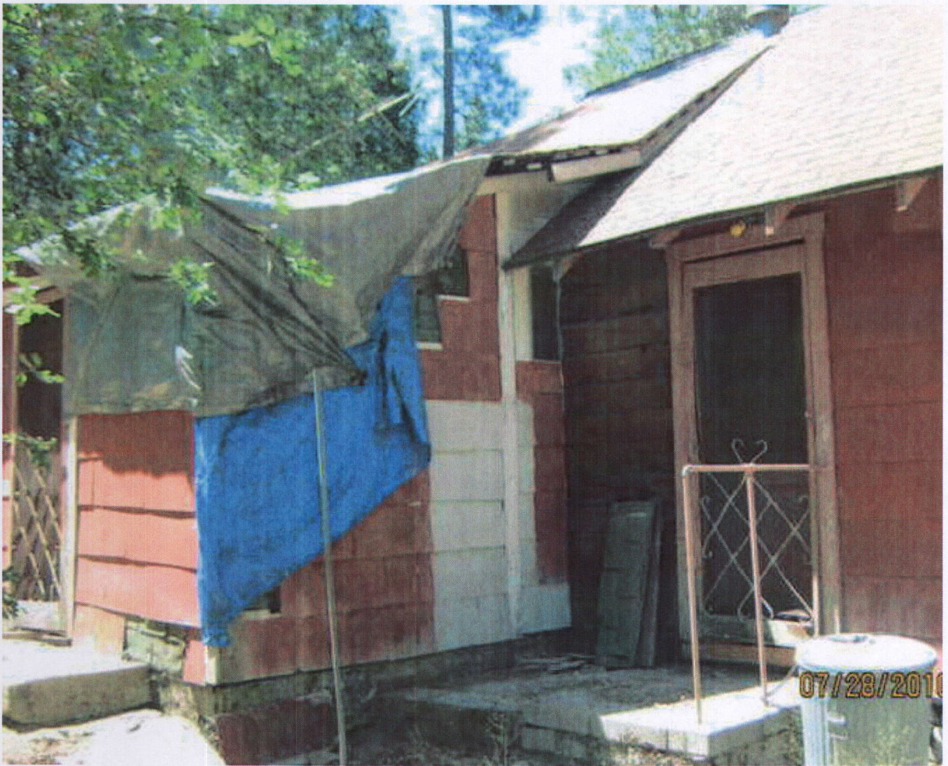
CForrey / Structure is still in substandard condition - 07/28/2010
