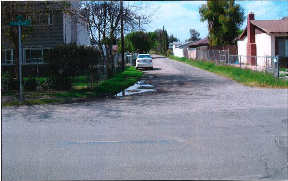
Figure 10. Norco MDP Lateral N-1D and Norco - Spirit Knoll Court Storm Drain. Intersection of Rose Court and Temescal Avenue, Rose Court looking west.
