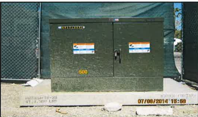
Figure 11. July 08, 2014: New Transformer for Existing Jail
