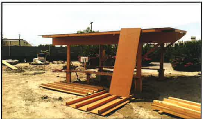
Figure 12. August 01, 2014: 115 Degree Weather requires Shade, Water and Misters for the MBC Construction Crew
