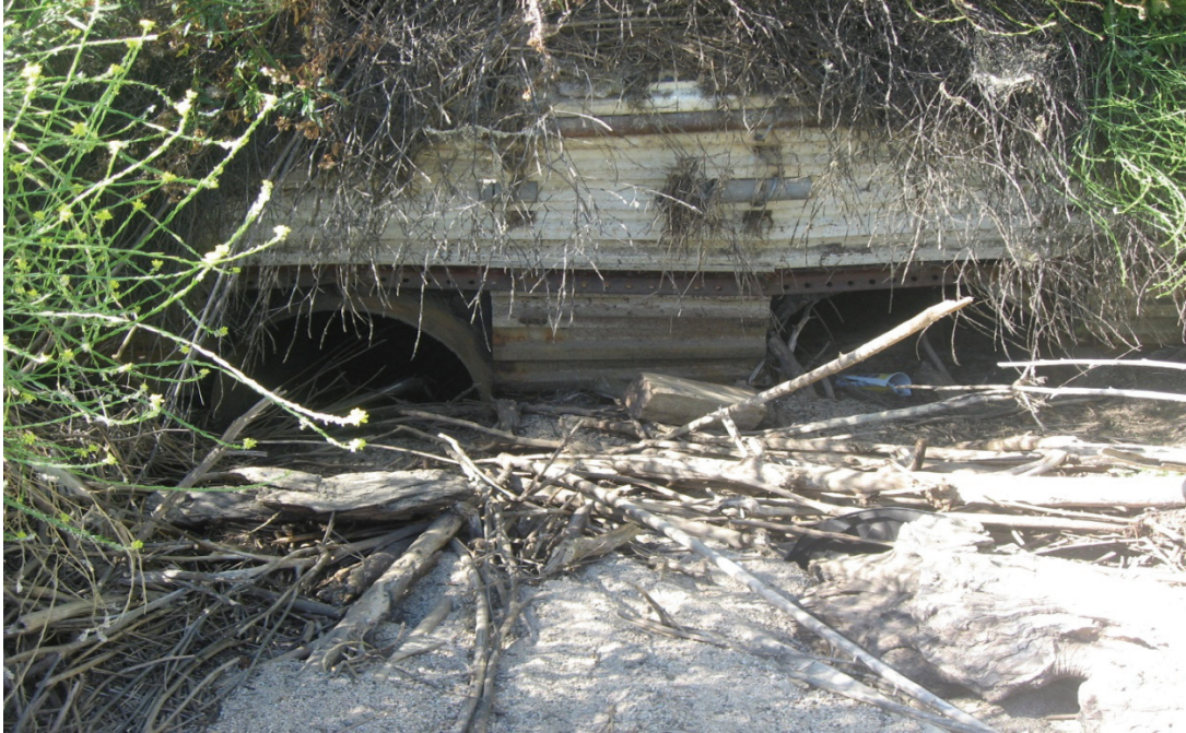
Photograph 11: Double culvert under dirt driveway that conveys flow to French Valley Creek downstream – facing south
