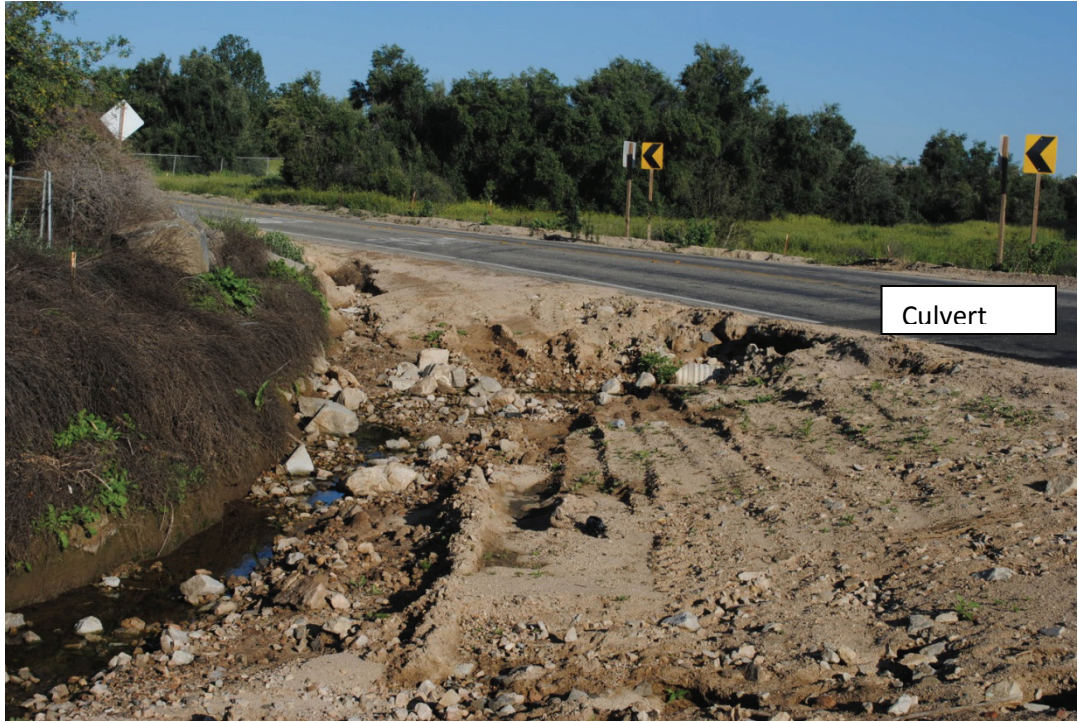
Photograph 9: Culvert Under Los Alamos Road – facing northwest looking at Los Alamos Road
