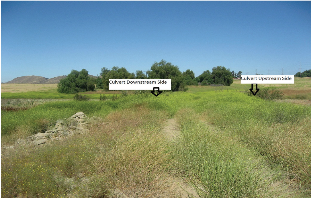
Photograph 12: Dirt driveway that contains the double culvert which conveys flows to French Valley Creek downstream – facing west
