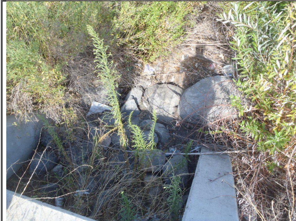
Photo 44 Date: 08-20-2013 Feature: Drainage 9 Direction: East Description: Downstream view of Drainage 9 from a culvert outlet beneath Whitewood Road.
