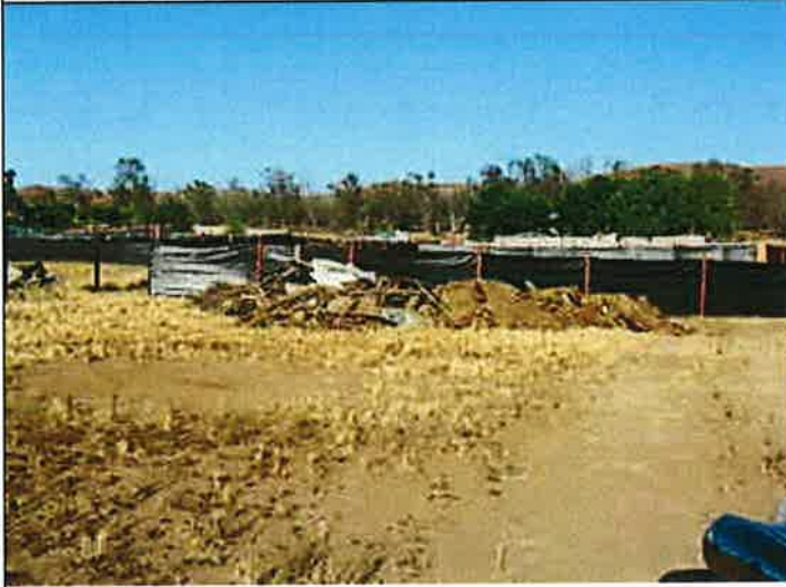
Accumulated rubbish remains-JMorris 4/17/15
