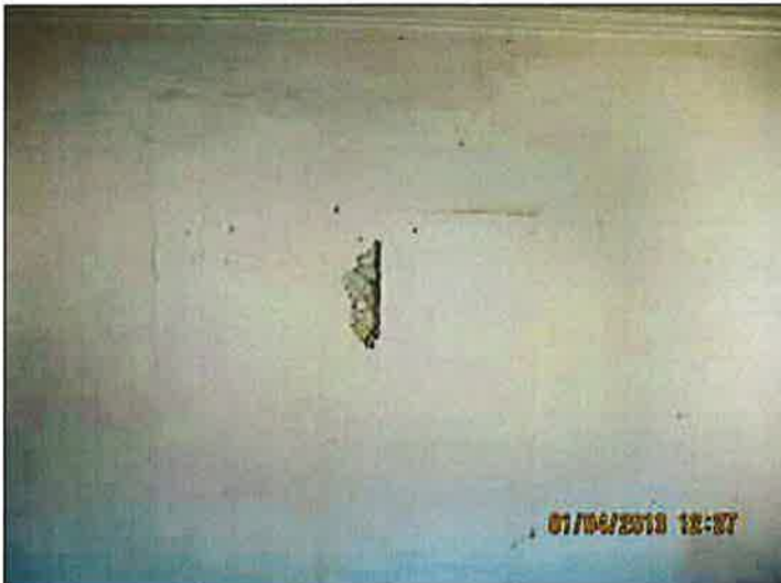
Damaged Wall 1/4/13 J. Cole
