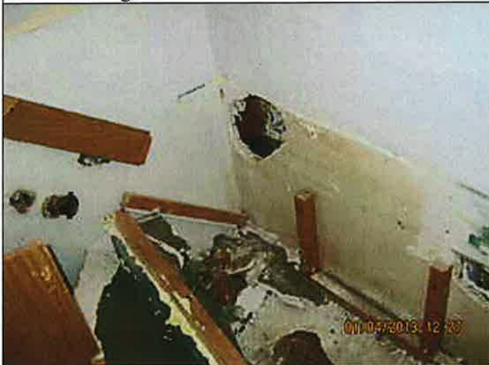
Damaged Wall 1/4/13 J. Cole
