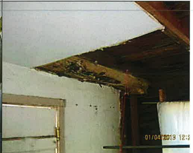
Damaged Ceiling 1/4/13 J. Cole
