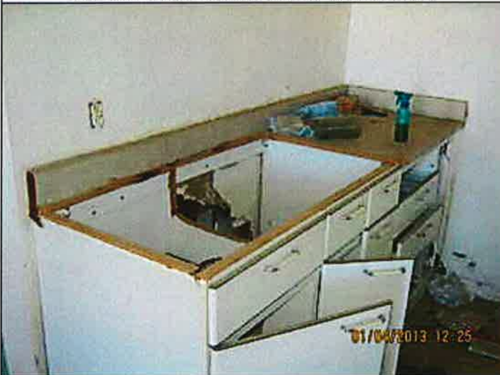
Missing Kitchen Sink 1/4/13 J. Cole
