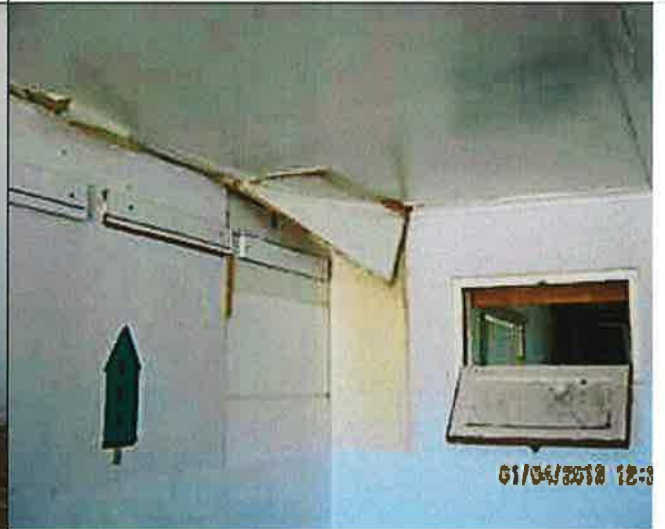
Damaged Ceiling 1/4/13 J. Cole
