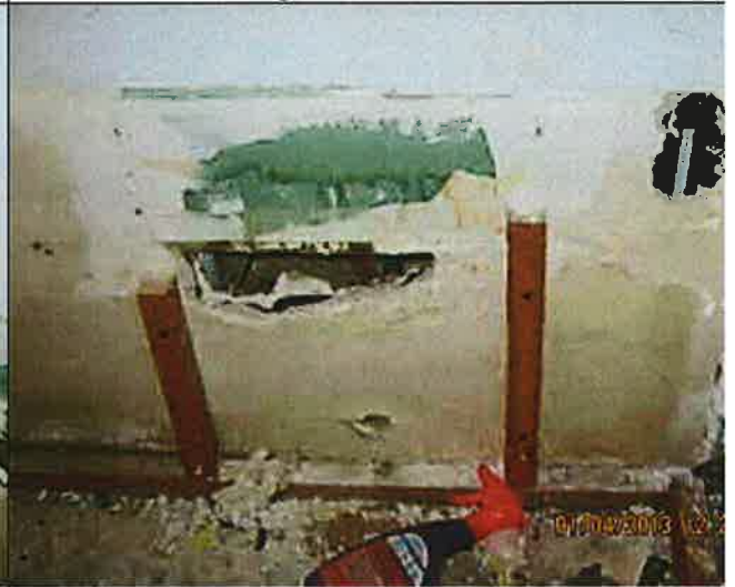
Damaged Wall 1/4/13 J. Cole
