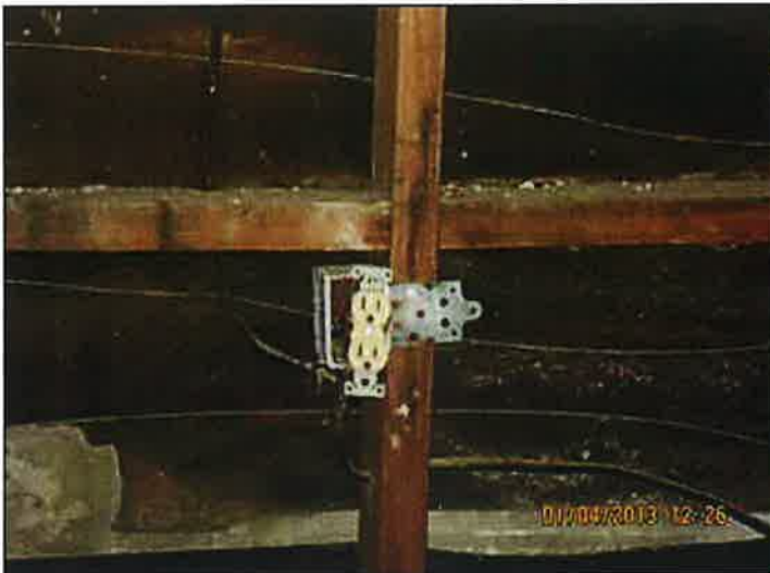
Damaged Wall/Outlet 1/4/13 J. Cole
