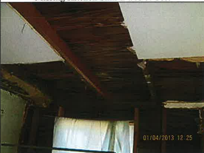
Damaged Ceiling 1/4/13 J. Cole
