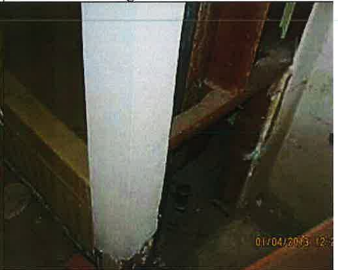
Damaged Wall 1/4/13 J. Cole
