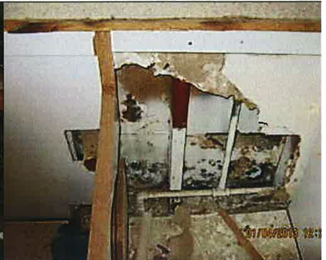
Damaged Wall 1/4/13 J. Cole
