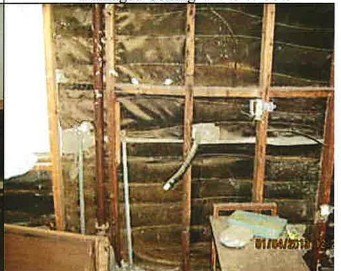
Damaged Wall/Pipes 1/4/13 J. Cole
