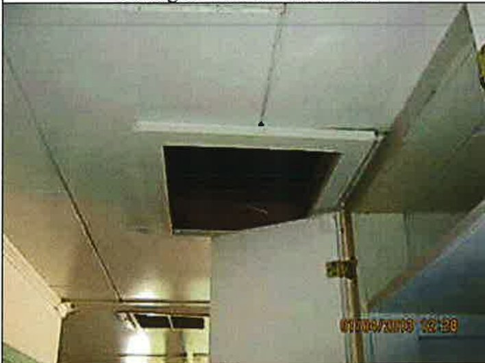
Damaged Ceiling 1/4/13 J. Cole
