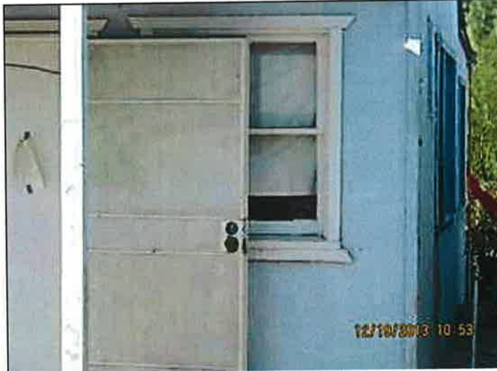
Substandard Structure 12/19/13 J. Cole
