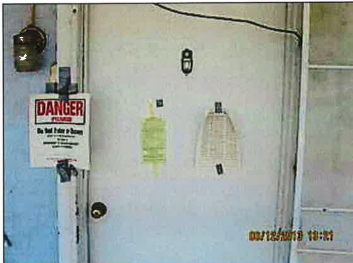
Substandard Structure 6/12/13 J. Cole
