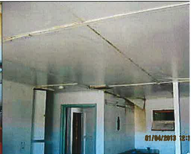
Damaged Ceiling 1/4/13 J. Cole
