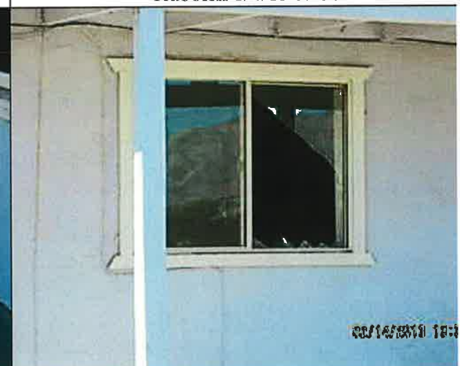
Substandard Structure 2/13/13 J. Cole
