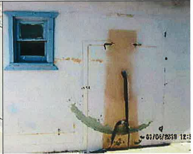
Missing Hot Water Heater 1/4/13 J. Cole
