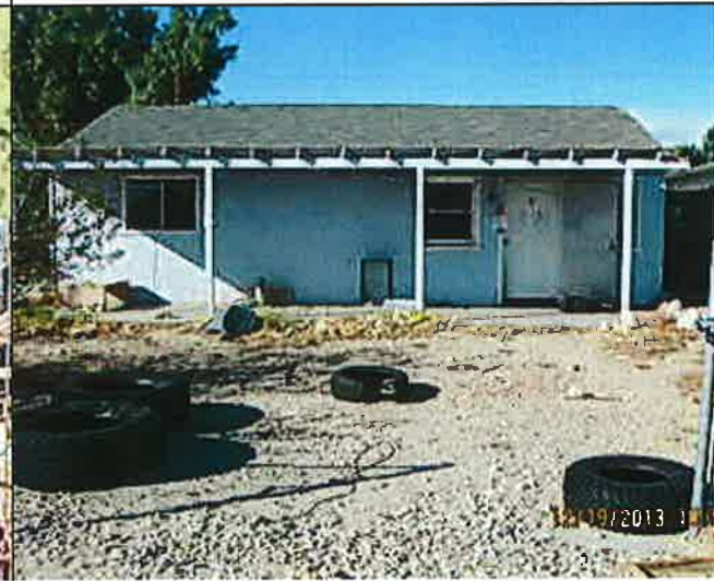
Substandard Structure 12/19/13 J. Cole
