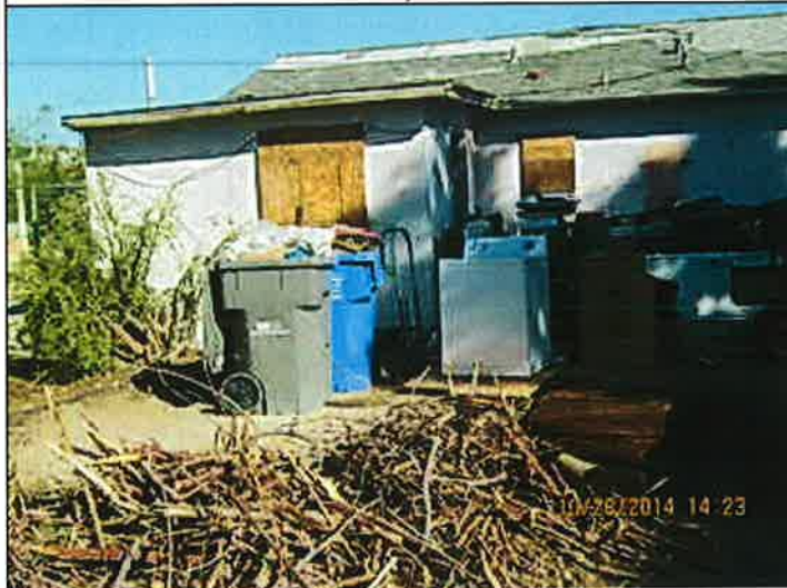
E. Torres; rear of substandard structure and rubbish
