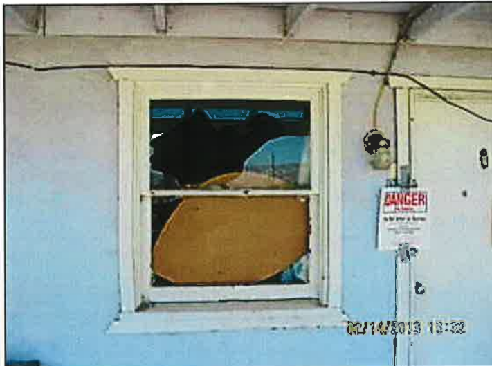
Substandard Structure 2/13/13 J. Cole
