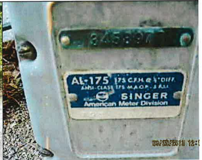
Gas Meter 3/29/13 J. Cole
