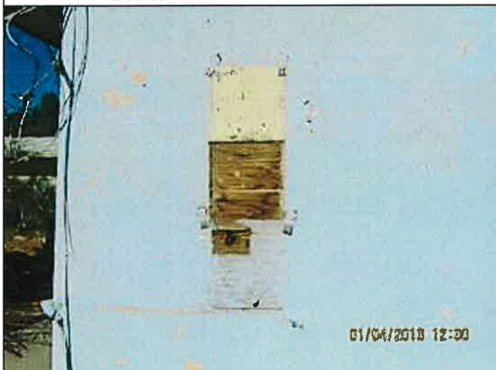
Missing Electric Meter and Box 1/4/13 J. Cole
