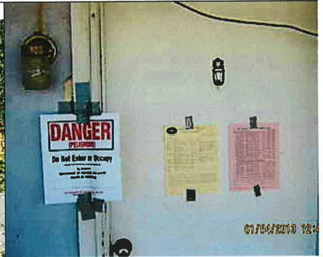
Notice of Violation, Notice of Defects, Danger/Not Enter Sign 1/4/13 J. Cole
