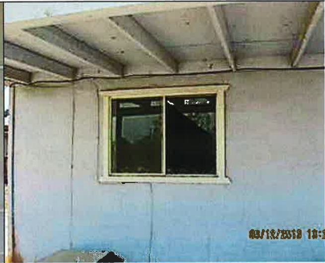
Substandard Structure 6/12/13 J. Cole
