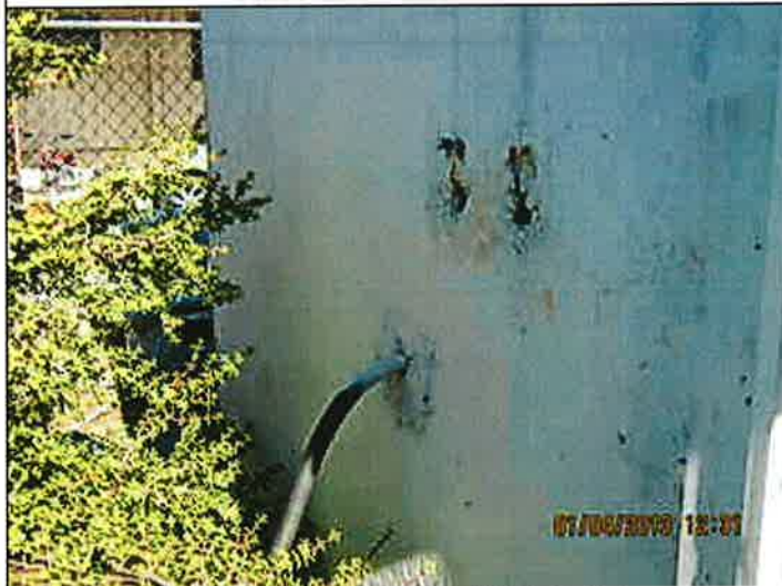
Damage Wall/Pipes 1/4/13 J. Cole
