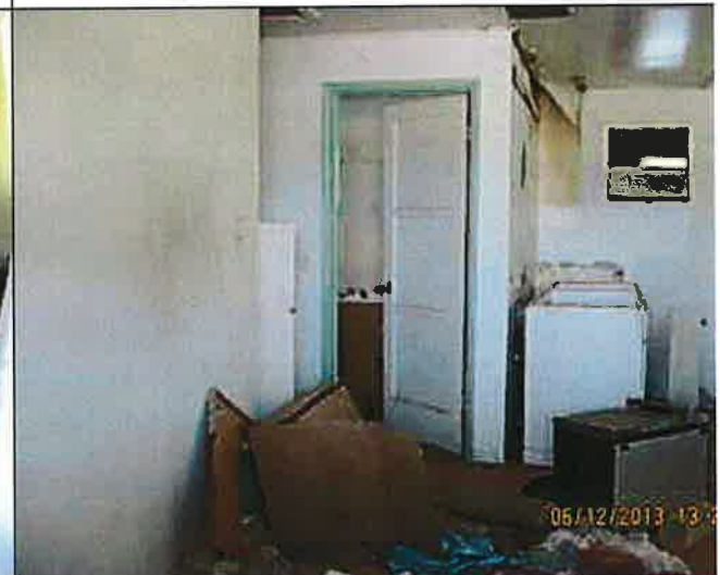
Substandard Structure 6/12/13 J. Cole
