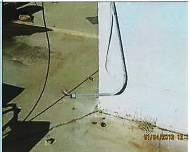
Missing Electric Meter and Box 1/4/13 J. Cole
