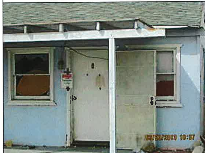
Broken Windows 3/20/13 J. Cole
