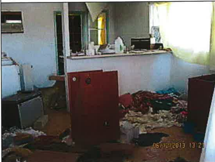
Substandard Structure 6/12/13 J. Cole
