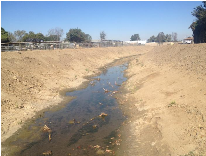
Location 17: Facing northeast, upstream. Standing water is from inlet conveying nuisance flows.
