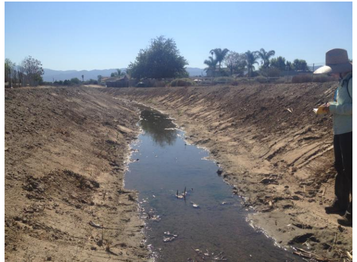
Location 17: Facing southwest, downstream. Evidence of recent maintenance activities (scrape marks along channel slopes)
