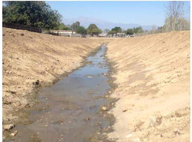
Location 18: Facing north, upstream. Water appears to be from inlet conveying nuisance flows.
