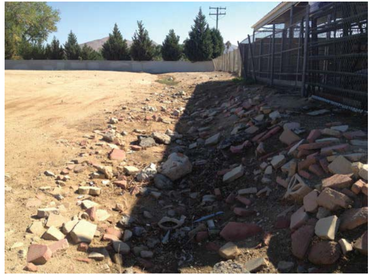
Location 13: Swale, facing east. Earthen ditch created apparently to drain nuisance flow into the channel. Broken bricks and concrete have been placed in the channel presumably to reduce erosion.
