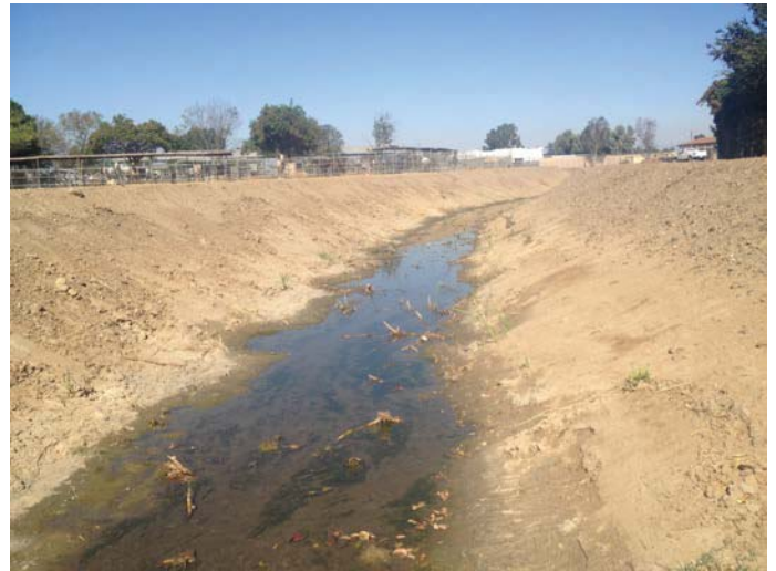
Location 20: Facing northeast, upstream. Bed 9ft. Bank 26ft. Standing water is from nuisance flows.
