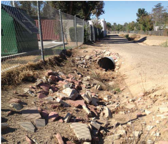
Location 13: Swale, facing west. Earthen ditch created apparently to drain nuisance flow into the channel. RCP crosses under access road and outlets into channel.
