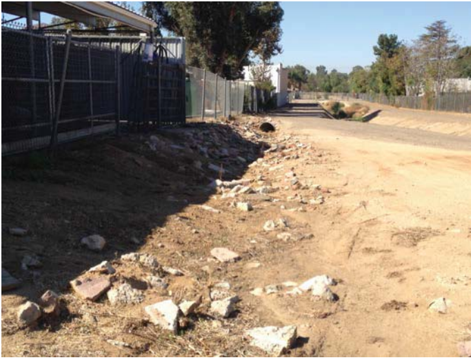
Location 12: Swale facing west, downstream. Earthen ditch for nuisance flows. Broken bricks and concrete have been placed in the ditch.
