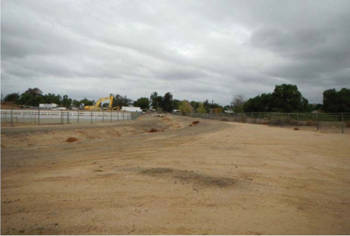
Photograph 11 - Looking north at the northeastern end of the subject property. Note the excavator on the property to the west.
