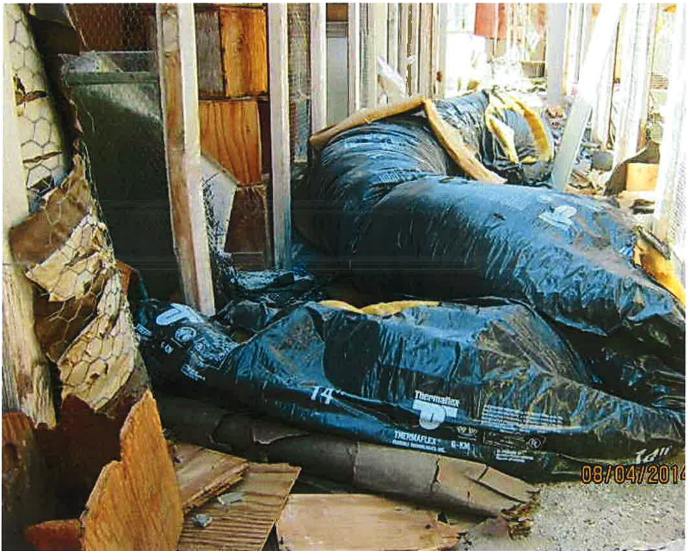
Inside str. # 4. Trash, debris and insulation present. 16 of 20. RH - 08/04/2014
