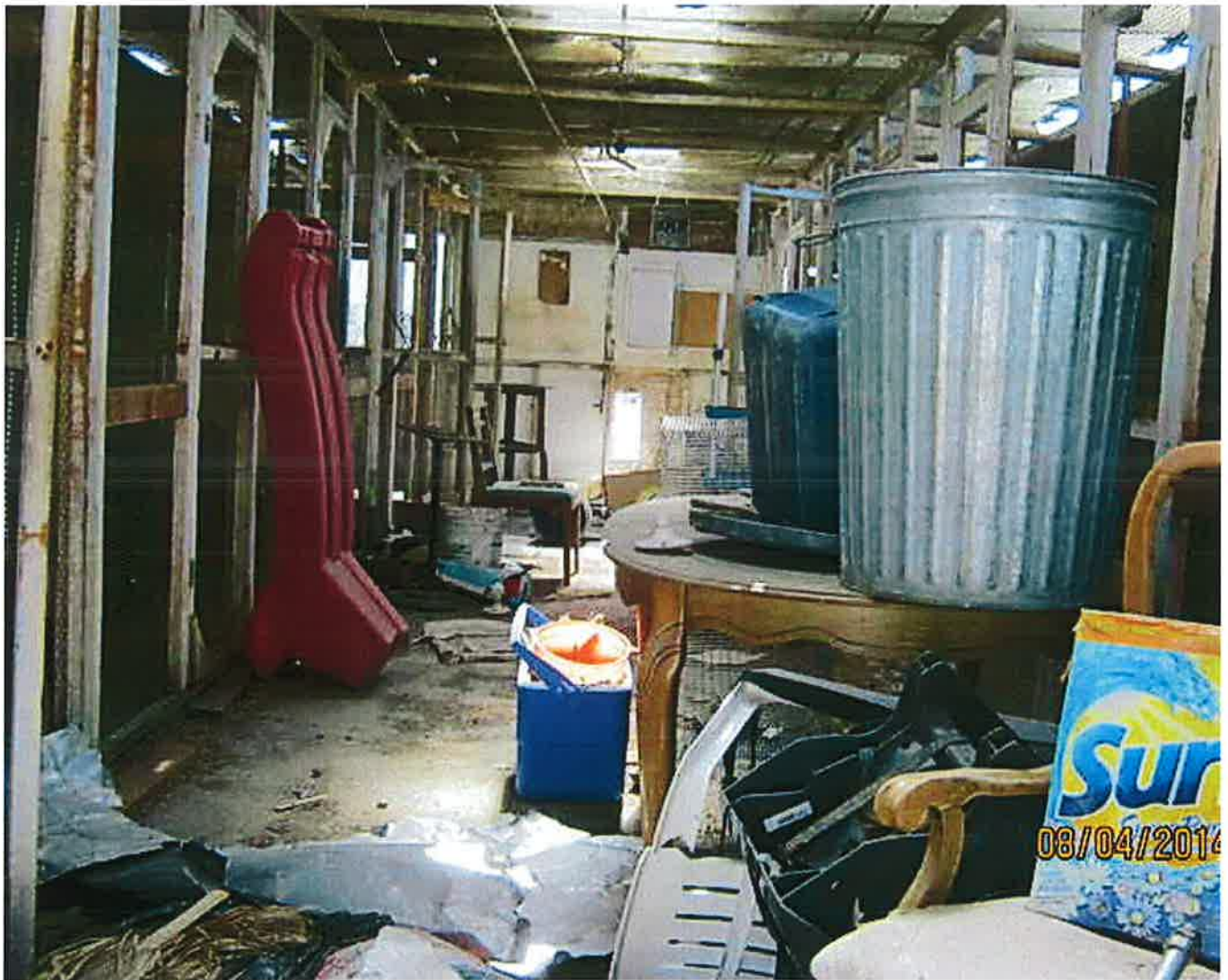
Inside str. # 3. Full of trash and debris. 12 of 20. RH - 08/04/2014
