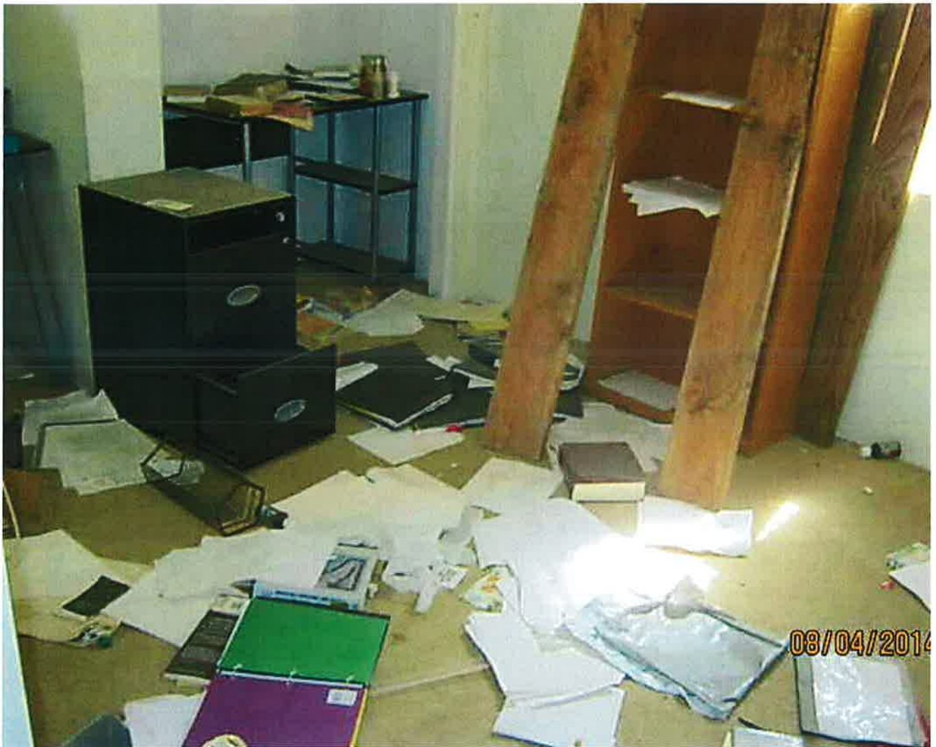
Bedroom of str. # 1. full of trash and debris. 6 of 20. RH - 08/04/2014
