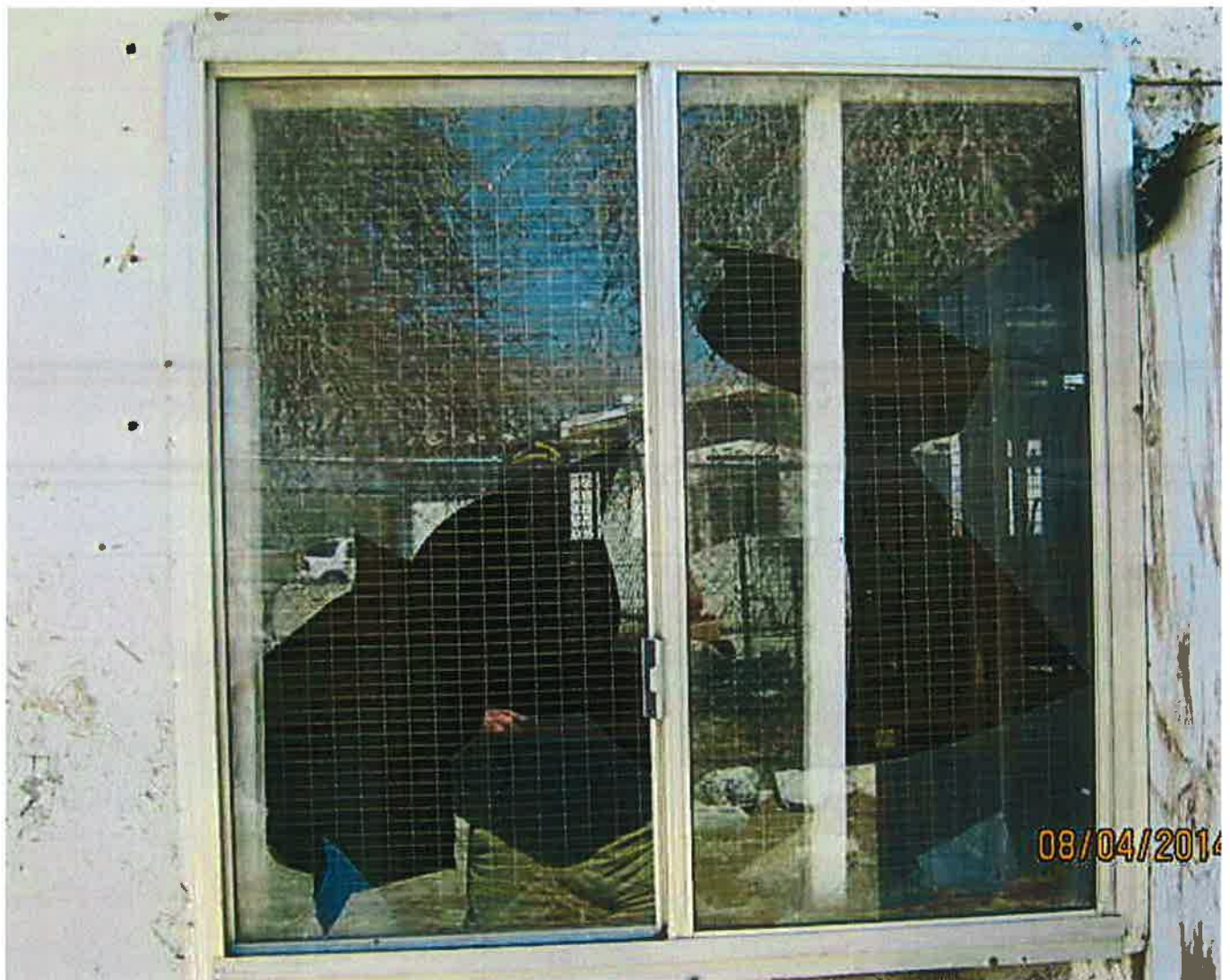
Broken window on str. # 3. 13 of 20. RH - 08/04/2014
