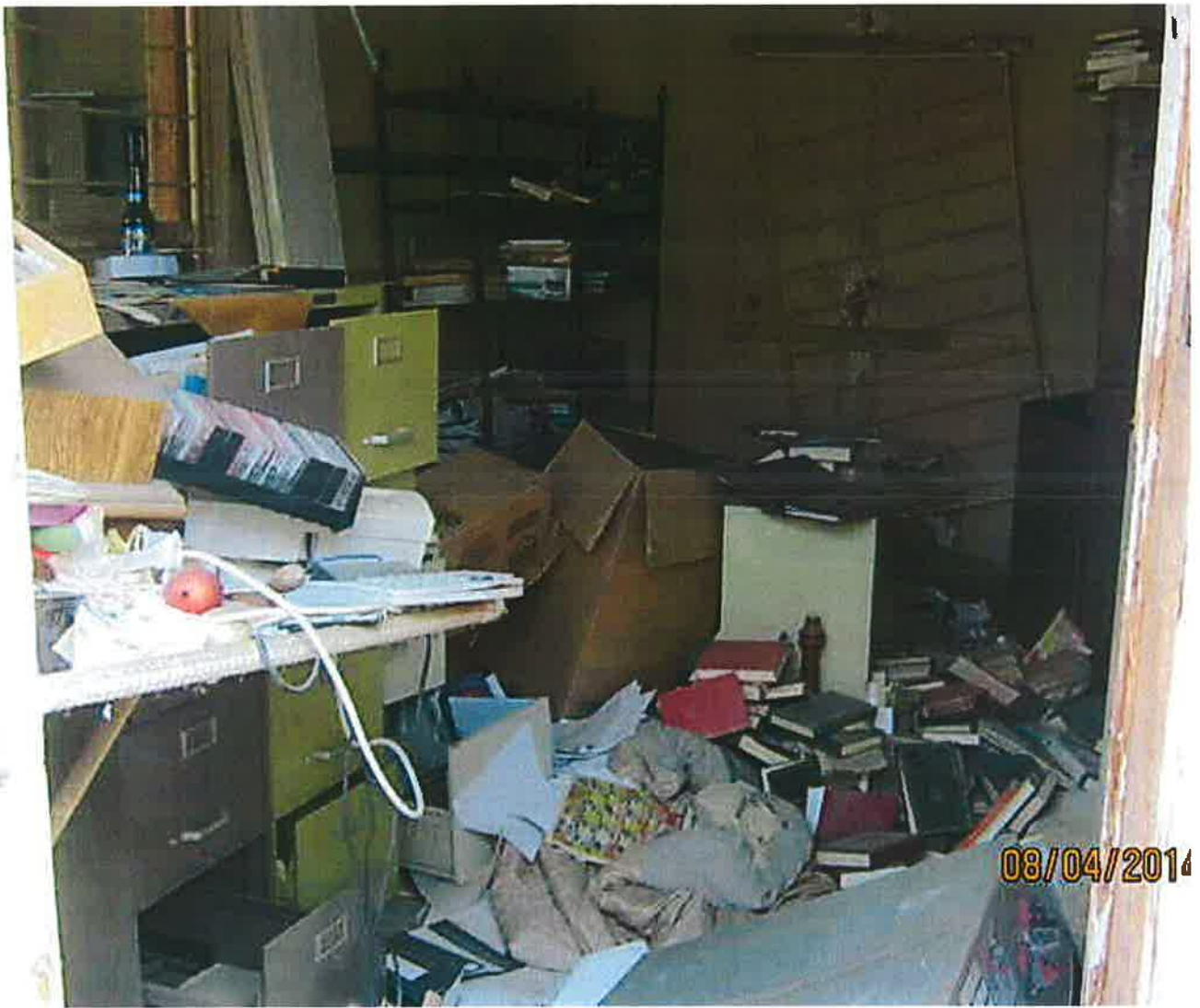
Inside room in str. # 2. trash and debris approx. 2 feet high. 9 of 20. RH - 08/04/2014
