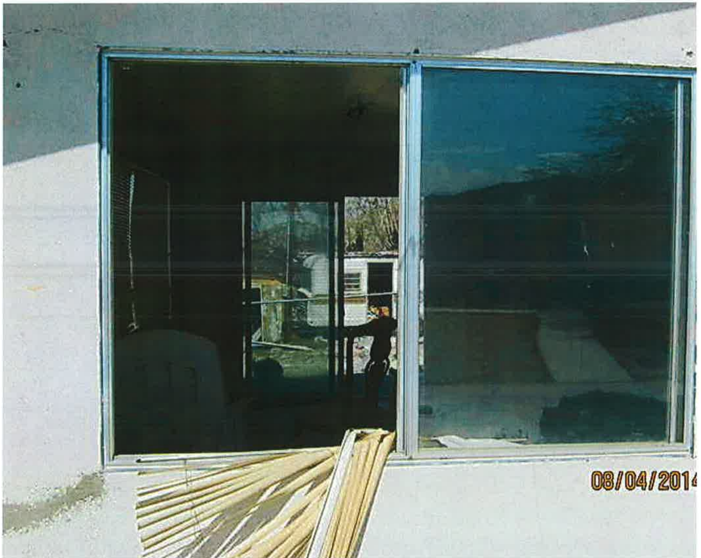
Broken window and str.# 1. 3 of 20. RH - 08/04/2014
