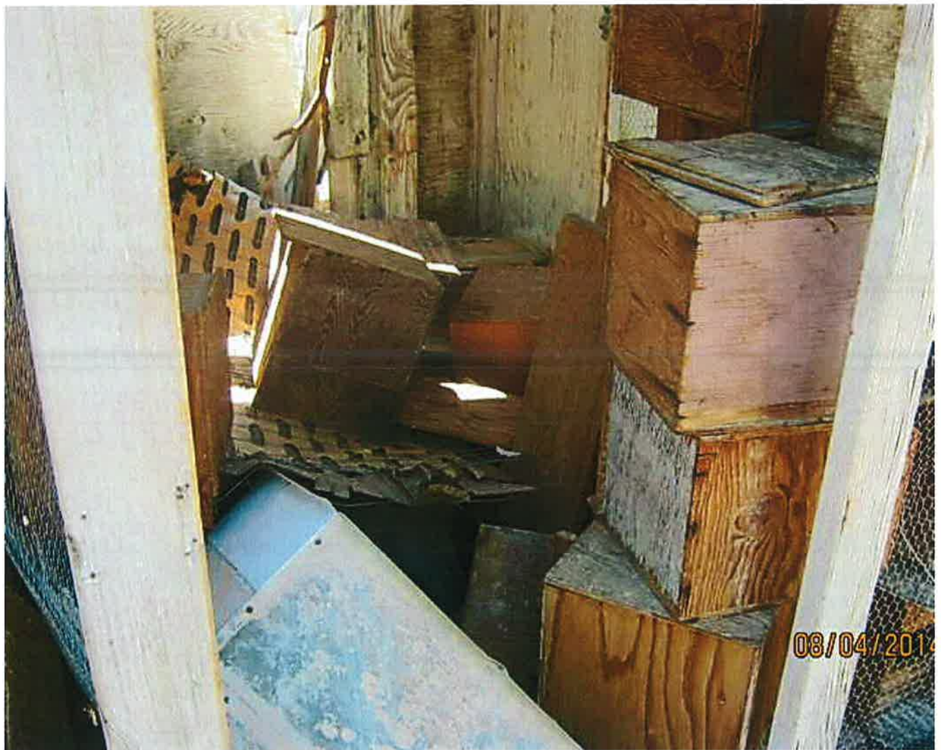
Inside str. # 4. Scrap wood throughout. 17 of 20. RH - 08/04/2014
