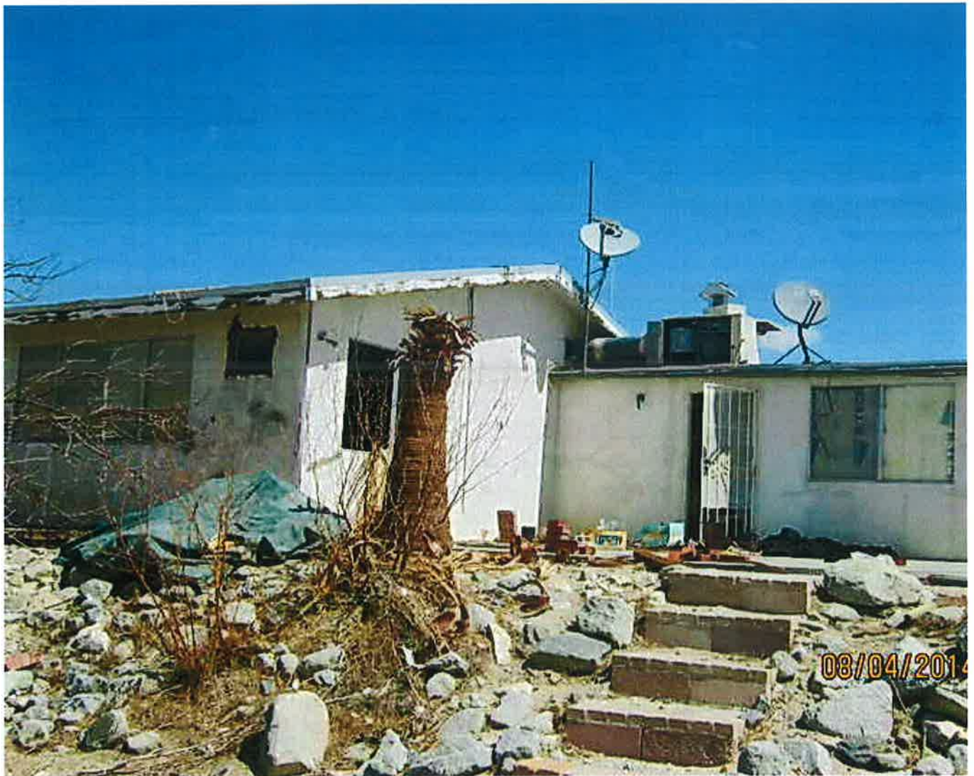
South side of structure # 1, open and unsecure, broken window. 2 of 20. RH - 08/04/2014
