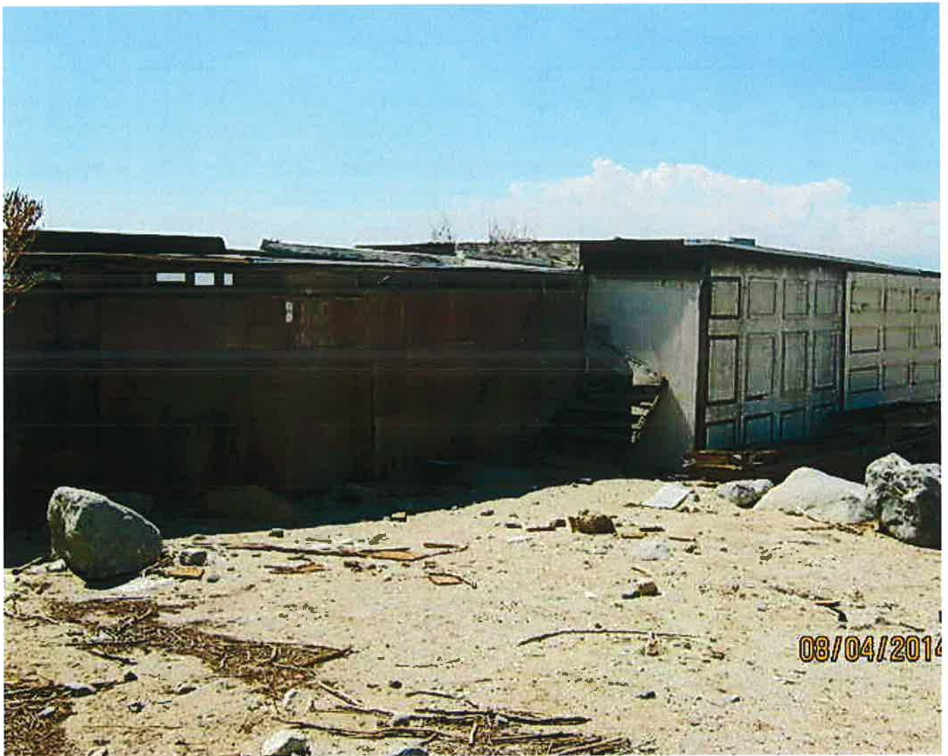
Structure # 4, built without permits & with garage doors. 14 of 20. RH - 08/04/2014
