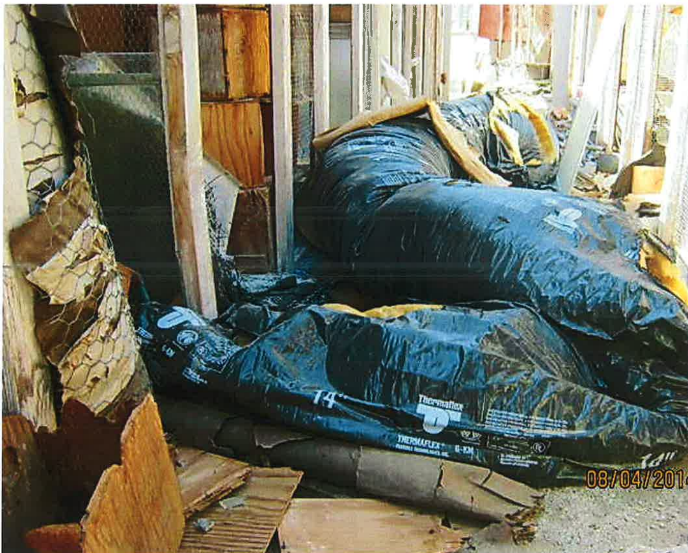
Inside str. # 4. Trash, debris and insulation present. 16 of 20. RH - 08/04/2014
