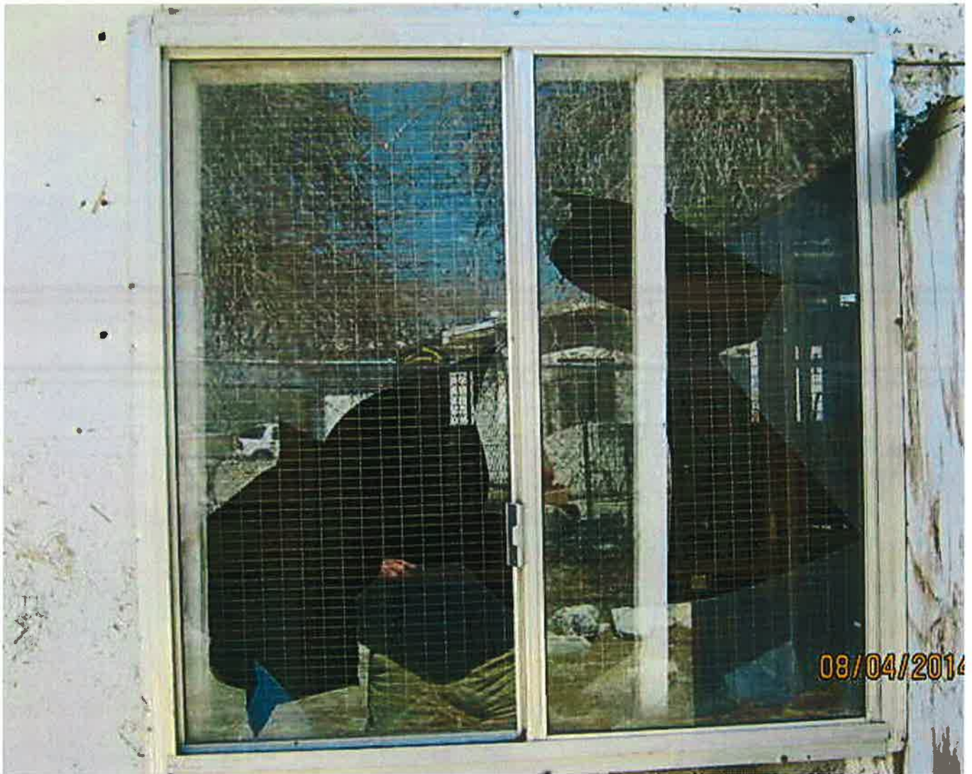
Broken window on str. # 3. 13 of 20. RH - 08/04/2014
