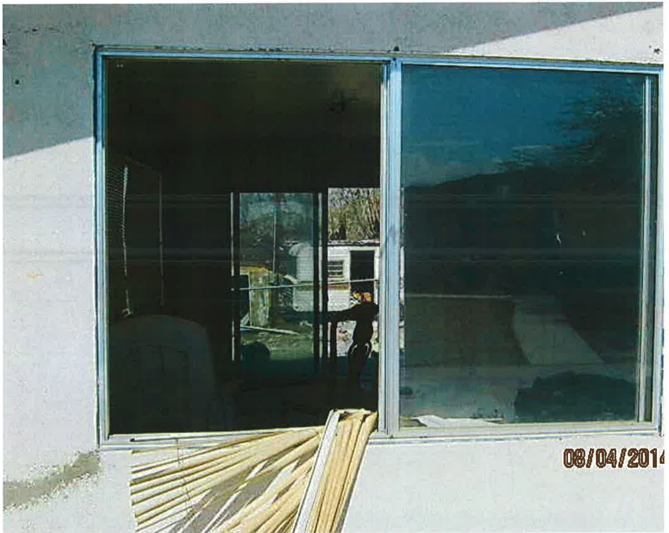
Broken window and str.# 1. 3 of 20. RH - 08/04/2014
