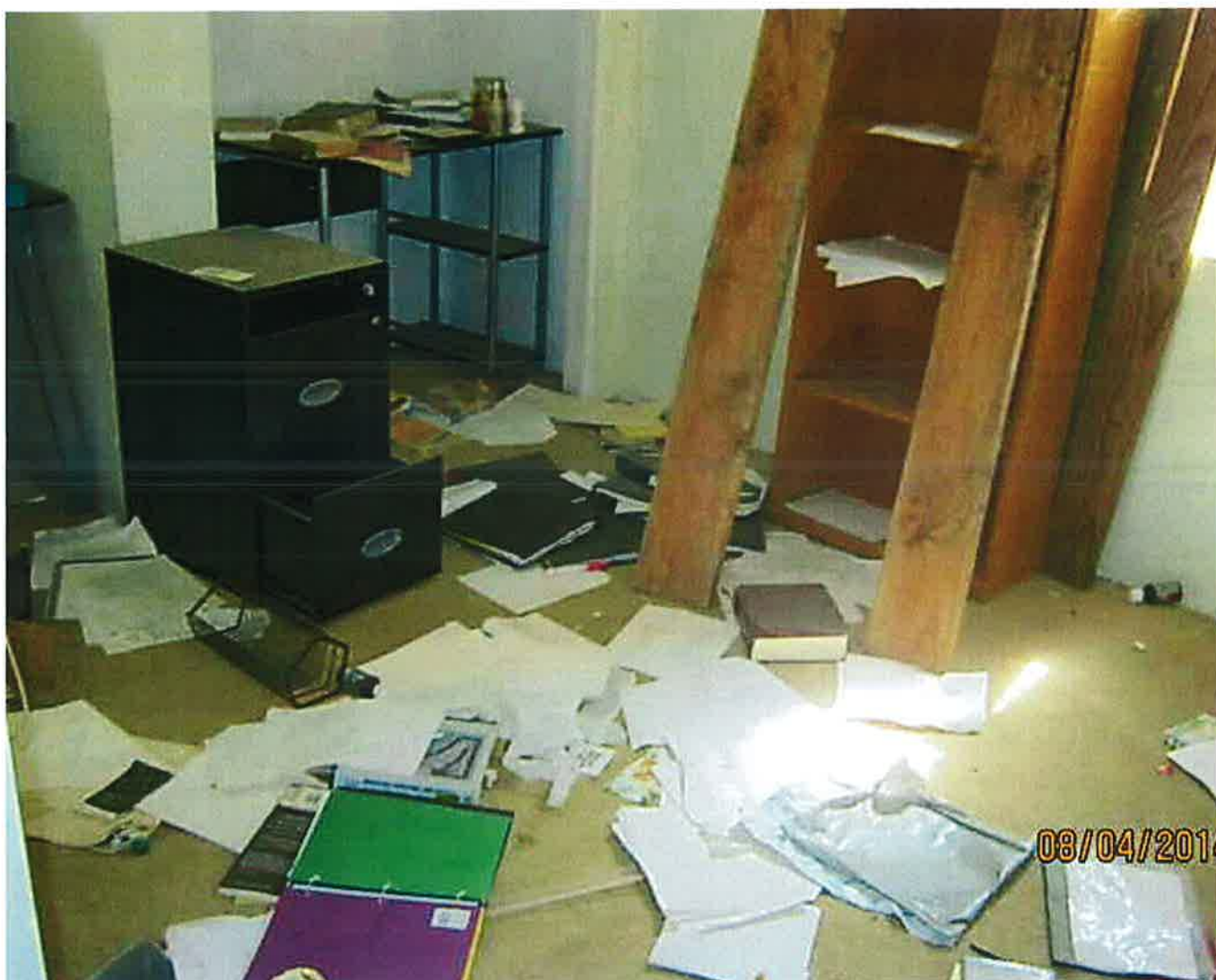
Bedroom of str. # 1. full of trash and debris. 6 of 20. RH - 08/04/2014
