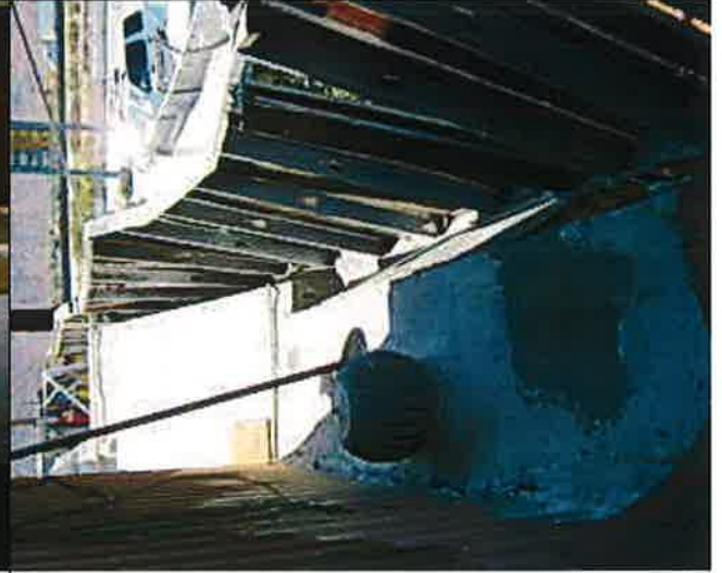
-09/26/14 - Initial Inspection SSST Verified - NC 14,17 - Pike
