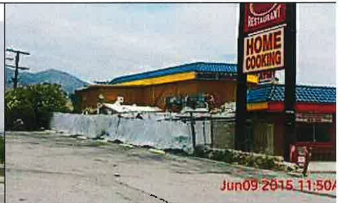
E. Torres; dilapidated and vandalized service equipment over kitchen
