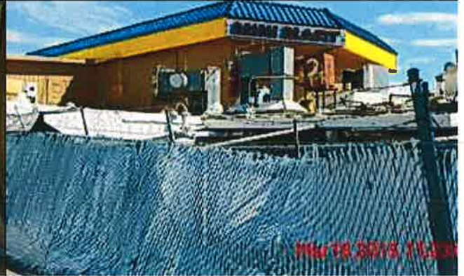
E. Torres; substandard structure continues to deteriorate
