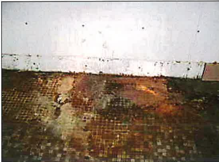
-09/26/14 - Initial Inspection SSST Verified - NOD# 12 - Pike
