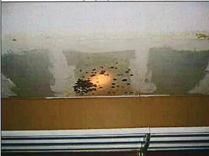
-09/26/14 - Initial Inspection SSST Verified - NOD# 11, 12, 14 - Pike
