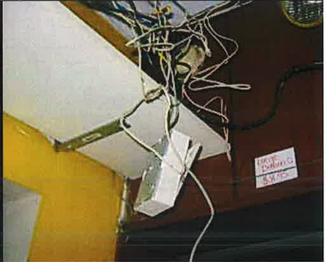
-09/26/14 - Initial Inspection SSST Verified - NC 6,14,15 - Pike
