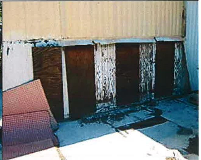
-09/26/14 - Initial Inspection SSST Verified - NC 14,17 - Pike
