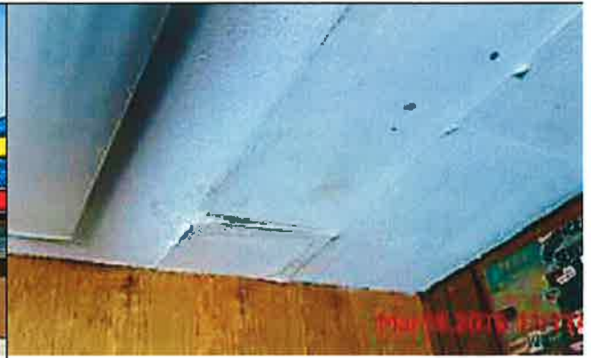
E. Torres; substandard structure continues to deteriorate
