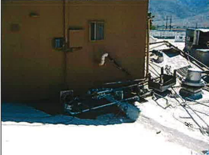
-09/26/14 - Initial Inspection SSST Verified - NOD# 14,17 - Pike
