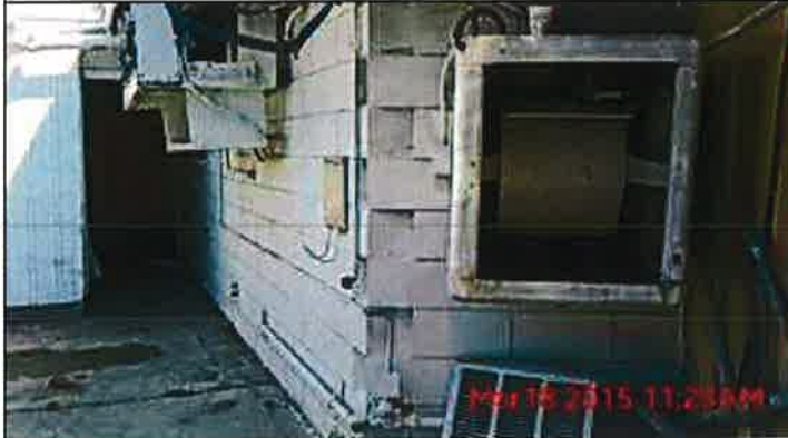
E. Torres; substandard structure continues to deteriorate
