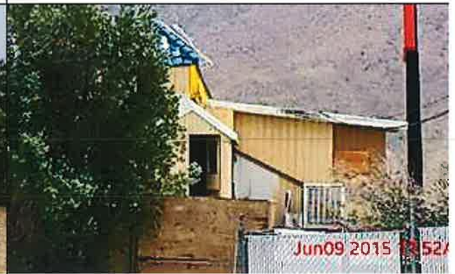
E. Torres; structure is not secure
