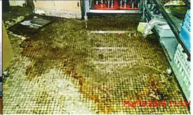
E. Torres; substandard structure continues to deteriorate
