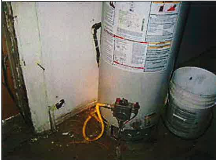
-09/26/14 - Initial Inspection SSST Verified - NOD# 1,2 - Pike
