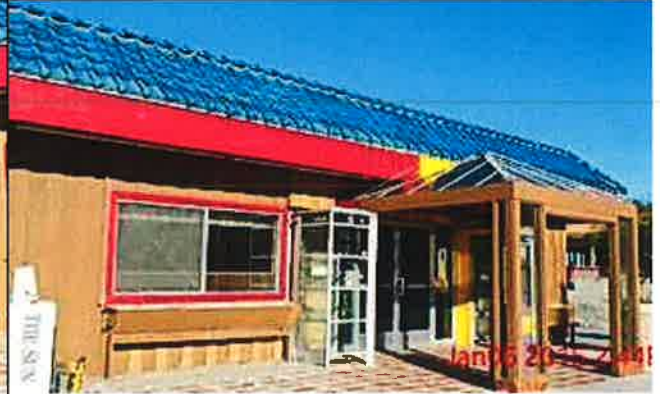
E. Torres; structure remains in substandard condition
