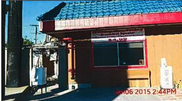
-E. Torres; structure remains in substandard condition
