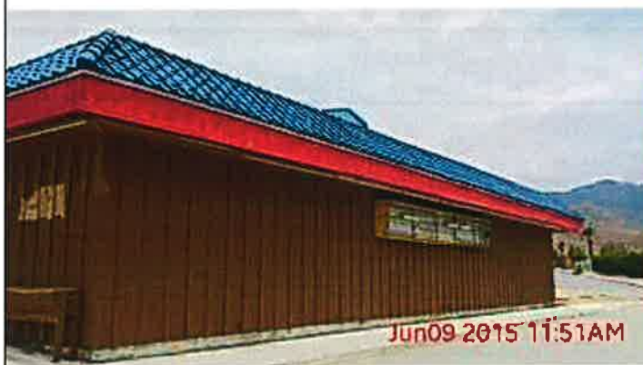
E. Torres; broken signage
