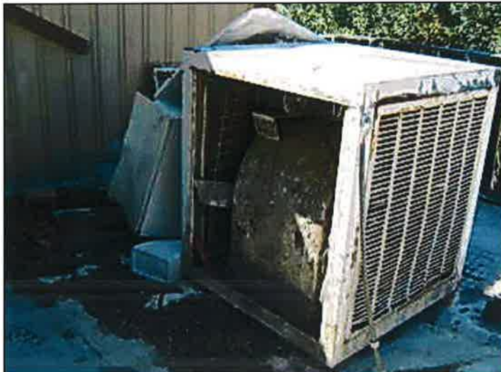
-09/26/14 - Initial Inspection SSST Verified - NOD# 14,17 - Pike
