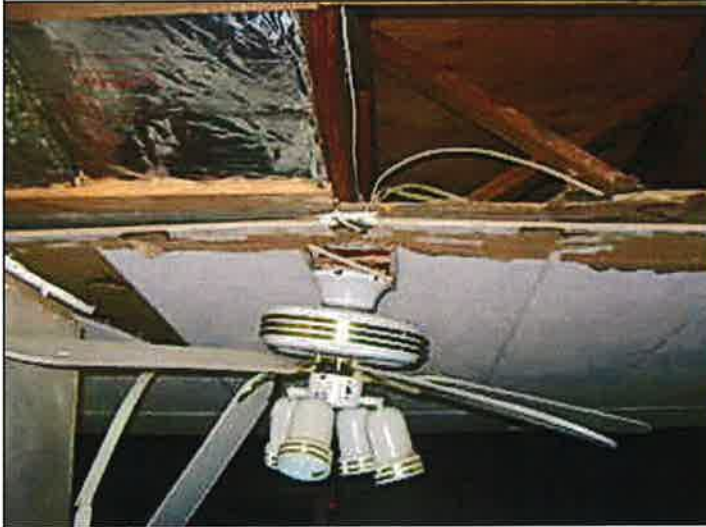
-09/26/14 - Initial Inspection SSST Verified - NOD# 11,14,15 - Pike
