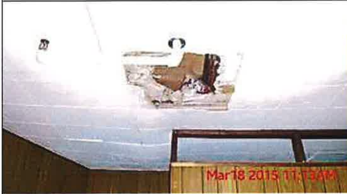
E. Torres; substandard structure continues to deteriorate
