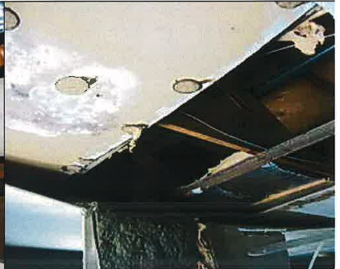
-09/26/14 - Initial Inspection SSST Verified - NC 11,14,15 - Pike
