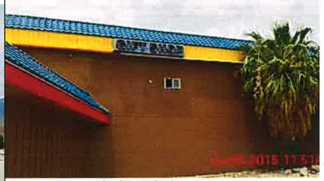
E. Torres; missing window/exposure to pests and elements
