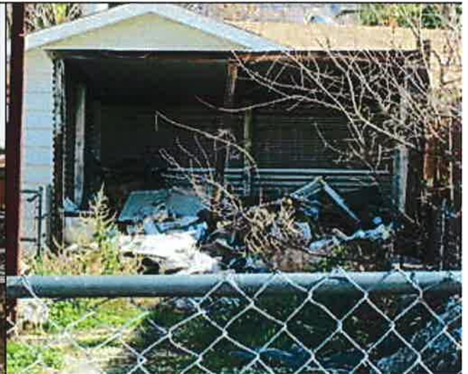
current photo - trash remains in defiance of code
