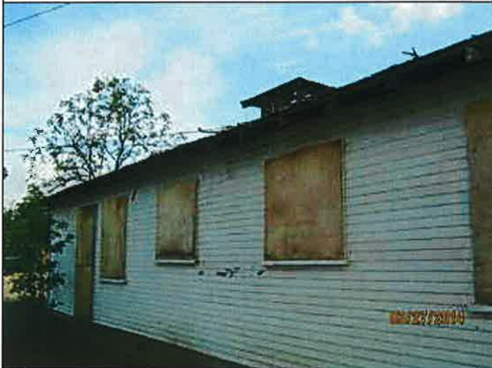
SUBSTANDARD STRUCTURE. LPADILLA
