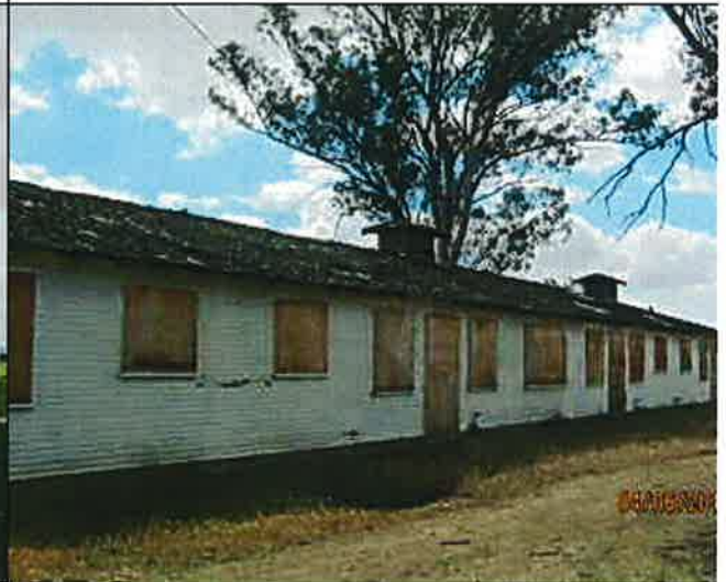
Property remains in violation. Lpadilla
