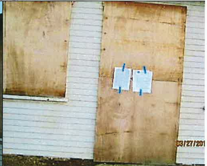
SUBSTANDARD STRUCTURE. LPADILLA
