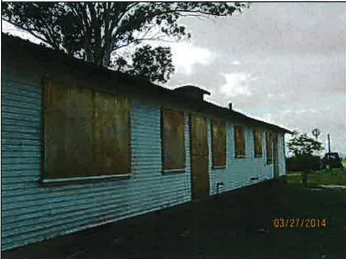
SUBSTANDARD STRUCTURE. LPADILLA
