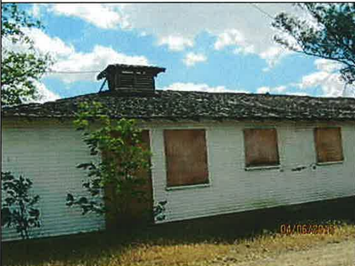
Property remains in violation. Lpadilla
