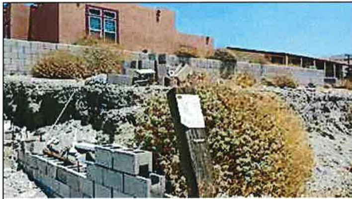
Notice of Violation 7/9/15 J. Cole
