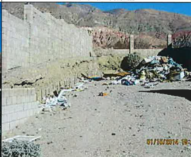
Unpermitted Grading 1/15/14 J. Cole
