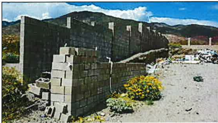
Unpermitted Grading/Cut 3/18/15 J. Cole
