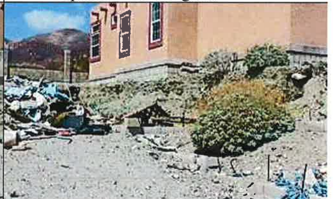
Unpermitted Grading/Cut 5/7/15 J. Cole
