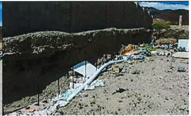
Unpermitted Grading/Cut 3/18/15 J. Cole
