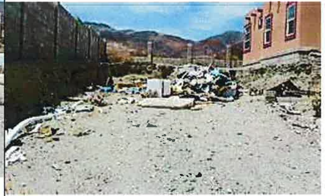
Unpermitted Grading/Cut 6/29/15 J. Cole
