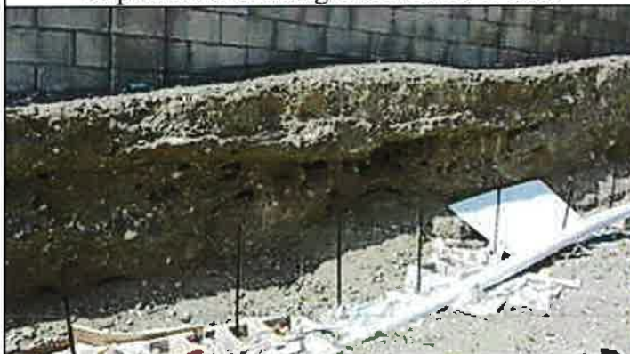
Unpermitted Grading/Cut 3/18/15 J. Cole
