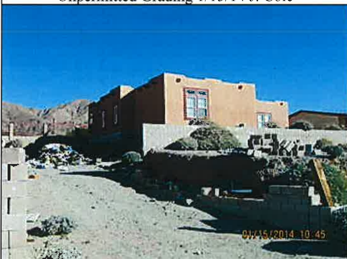
Unpermitted Grading 1/15/14 J. Cole
