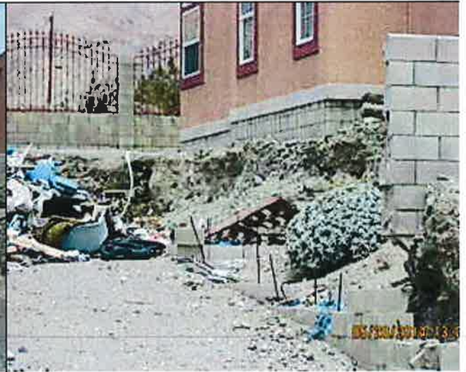
Unpermitted Grading 5/28/14 J. Cole
