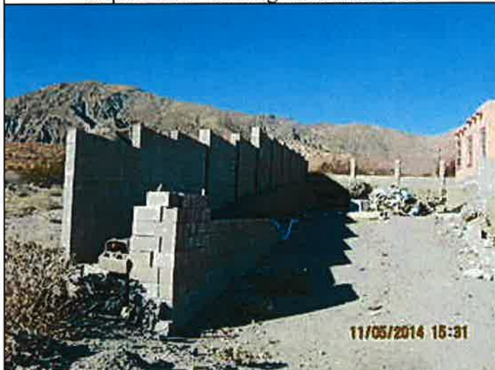
Unpermitted Grading/Cut 11/5/14 J. Cole
