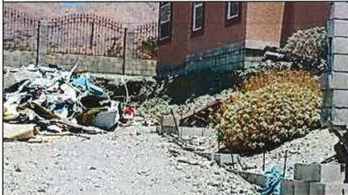
Unpermitted Grading 7/9/15 J. Cole
