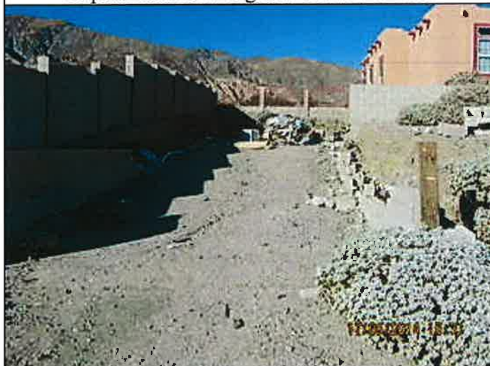
Unpermitted Grading/Cut 11/5/14 J. Cole
