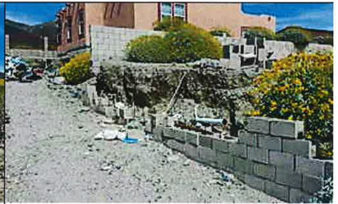
Unpermitted Grading/Cut 3/18/15 J. Cole
