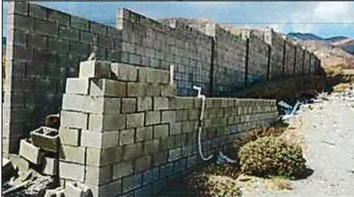
Unpermitted Grading/Cut 5/7/15 J. Cole
