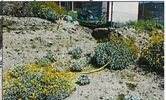
Unpermitted Grading/Cut 3/18/15 J. Cole
