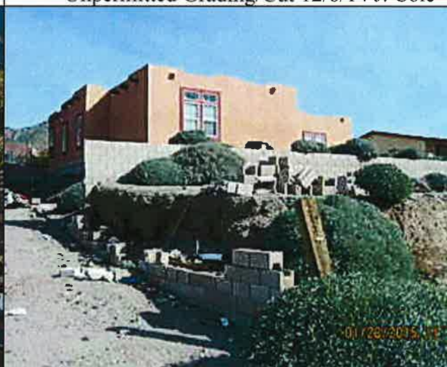
Unpermitted Grading/Cut 1/28/15 J. Cole
