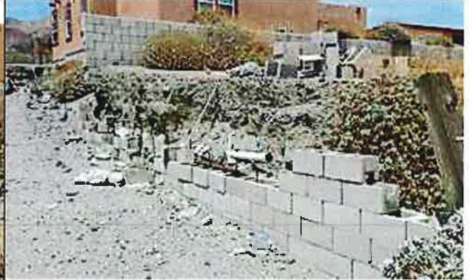
Cut Along the Front of the Property and Along the West Side of the Structure 6/29/15 J. Cole
