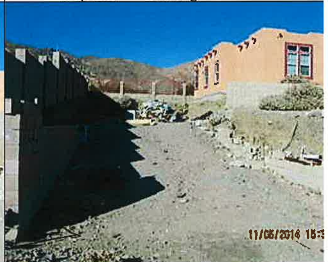
Unpermitted Grading/Cut 11/5/14 J. Cole
