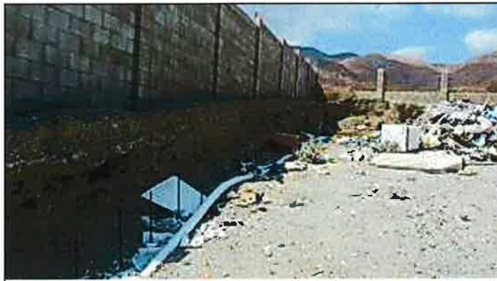
Unpermitted Grading/Cut 5/7/15 J. Cole
