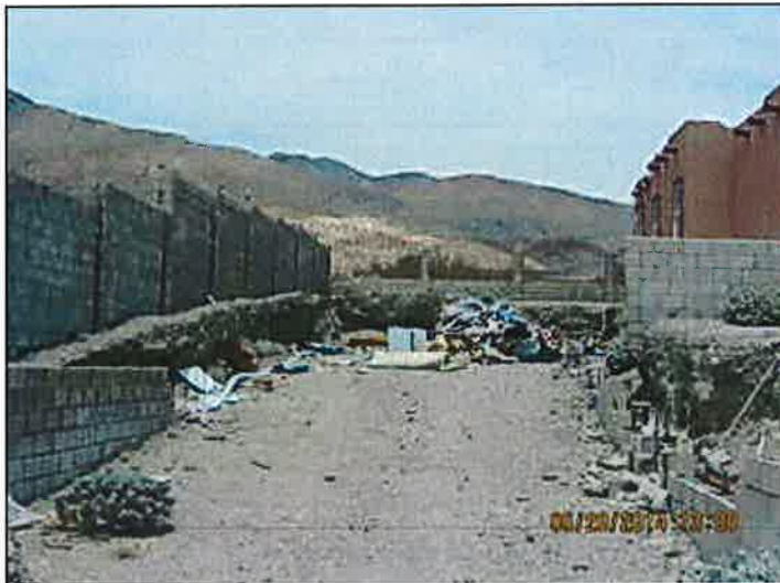
Unpermitted Grading 5/28/14 J. Cole
