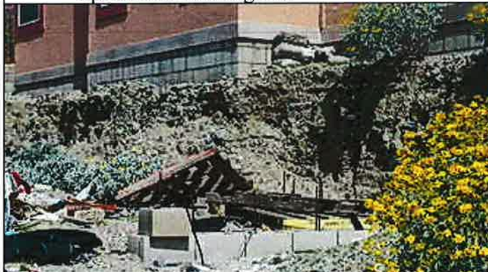
Unpermitted Grading/Cut 3/18/15 J. Cole
