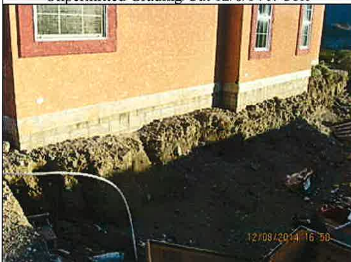
Unpermitted Grading/Cut 12/8/14 J. Cole
