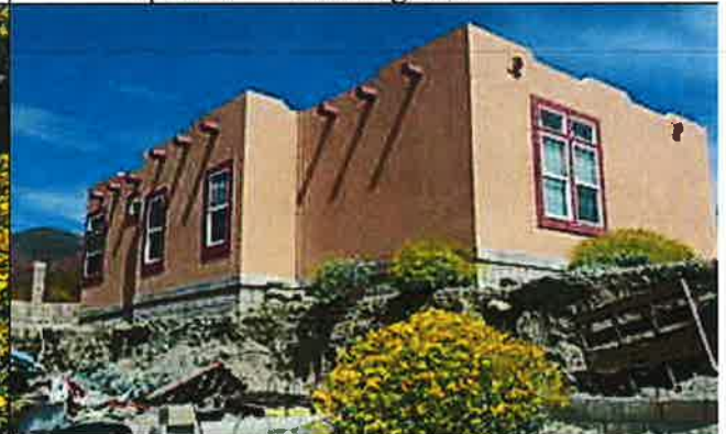
Unpermitted Grading/Cut 3/18/15 J. Cole
