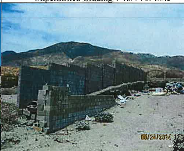
Unpermitted Grading 5/28/14 J. Cole
