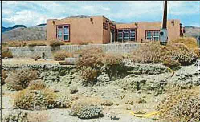
Substandard Structure 6/29/15 J. Cole
