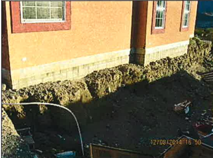
Deteriorated Foundation 12/8/14 J. Cole
