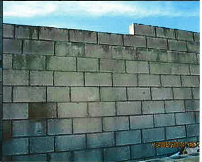
Substandard Block Wall 12/8/14 J. Cole
