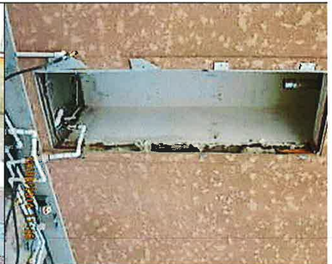
Missing Water Heater 12/8/14 J. Cole
