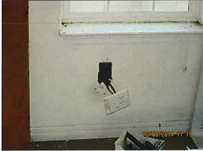
Hazardous Electrical 12/8/14 J. Cole
