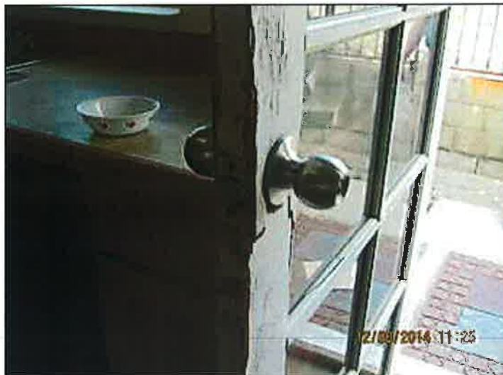
Damaged/Unsecured Rear Door 12/8/14 J. Cole
