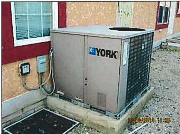
Air Conditioner Unit Intact 12/8/14 J. Cole
