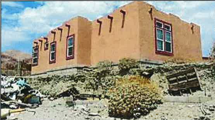
Substandard Structure 6/29/15 J. Cole
