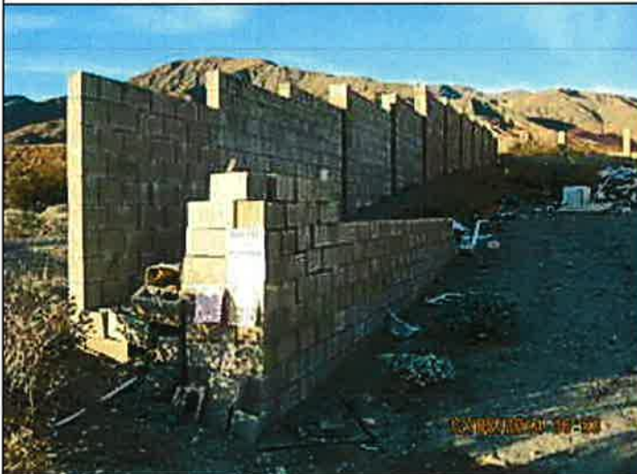
Substandard Block Wall 12/8/14 J. Cole
