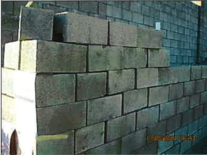
Substandard Block Wall 12/8/14 J. Cole
