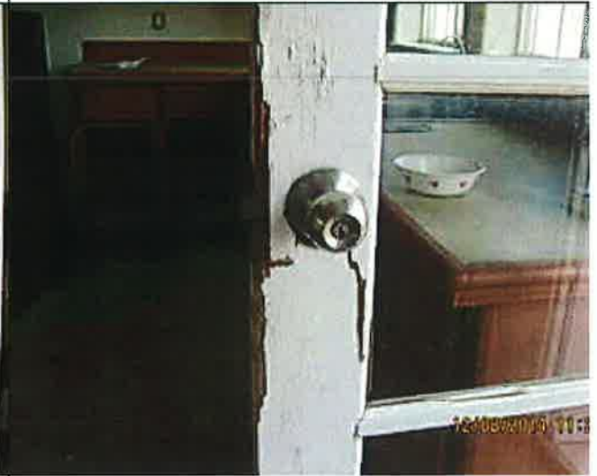
Damaged/Unsecured Rear Door 12/8/14 J. Col
