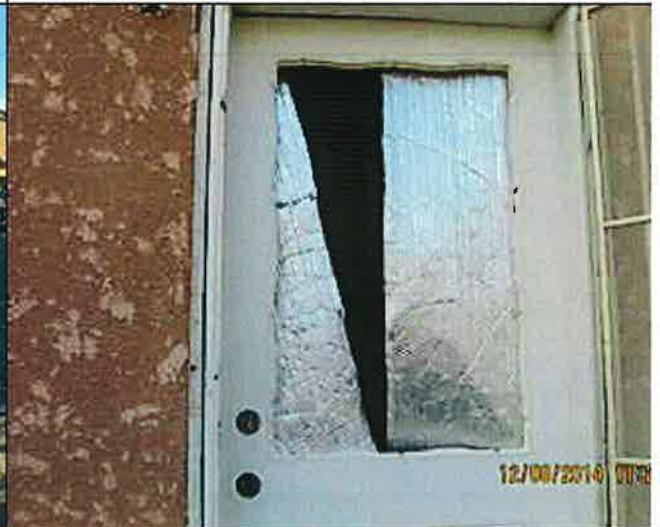
Damaged/Unsecured Rear Door 12/8/14 J. Col
