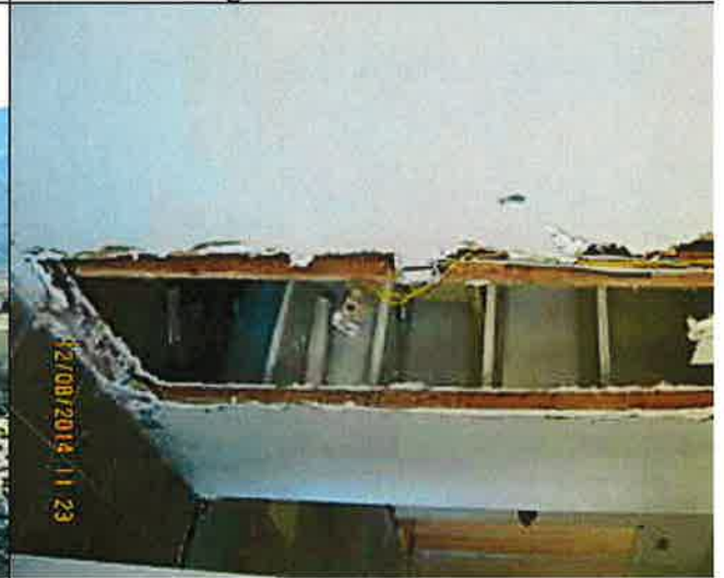
Hole in the Wall, Hazardous Electrical 12/8/14 J. Cole
