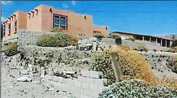
Substandard Structure 5/7/15 J. Cole
