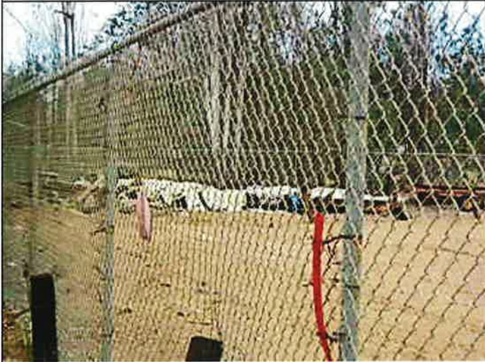
Accumulated rubbish remains-JMorris 5/6/15
