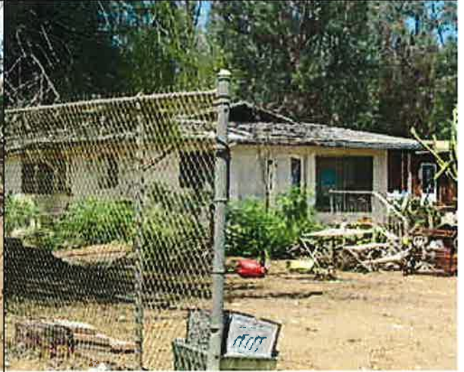
Structure remains substandard-JMorris 7/28/15
