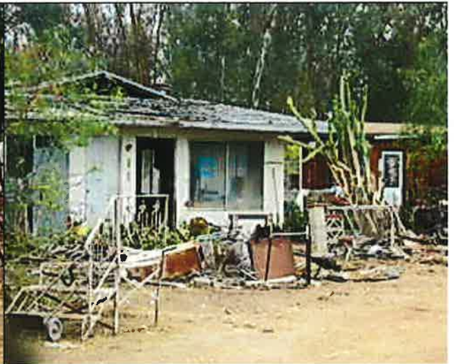
Structure remains substandard-JMorris 5/6/15
