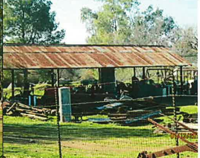
Accumulated Rubbish & Excessive Outside Storage. Lpadilla
