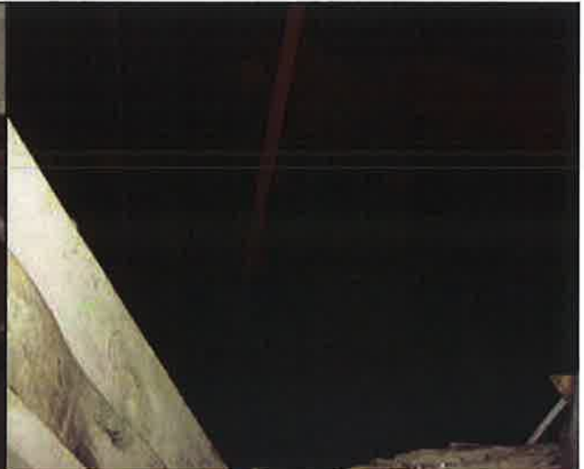
02/05/15 - Substandard Structure - NOD# 11,12,13,14,17 - Pike
