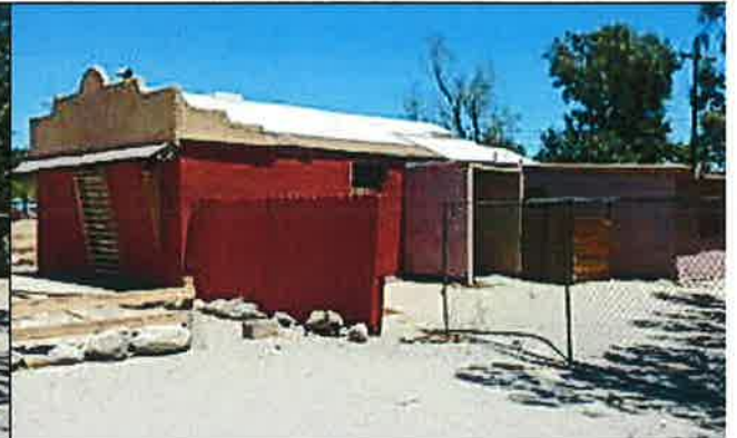
Substandard Structure 7/24/15 J. Cole
