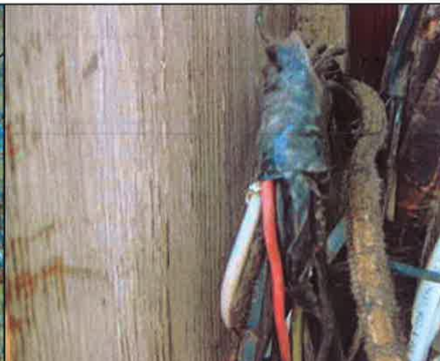
02/05/15 - Substandard Structure - NOD# 6,14,15 Pike
