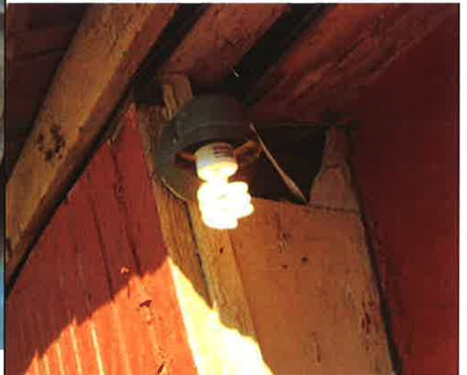
02/05/15 - Substandard Structure - NOD# 6,15 - J
