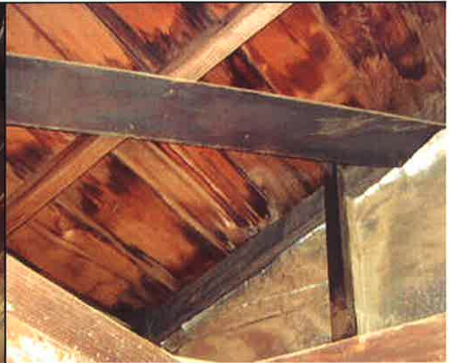
02/05/15 - Substandard Structure - NOD#11,12,13,14,17 - Pike
