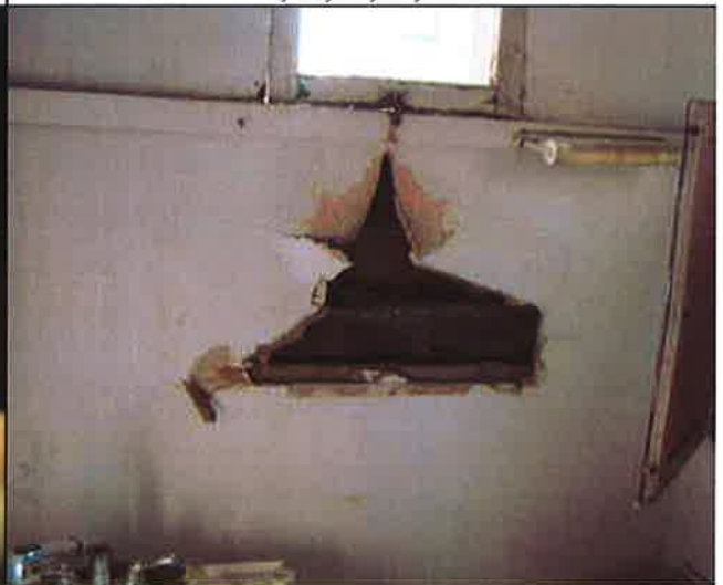
02/05/15 - Substandard Structure - NOD# 11,12,13,14,17 - Pike
