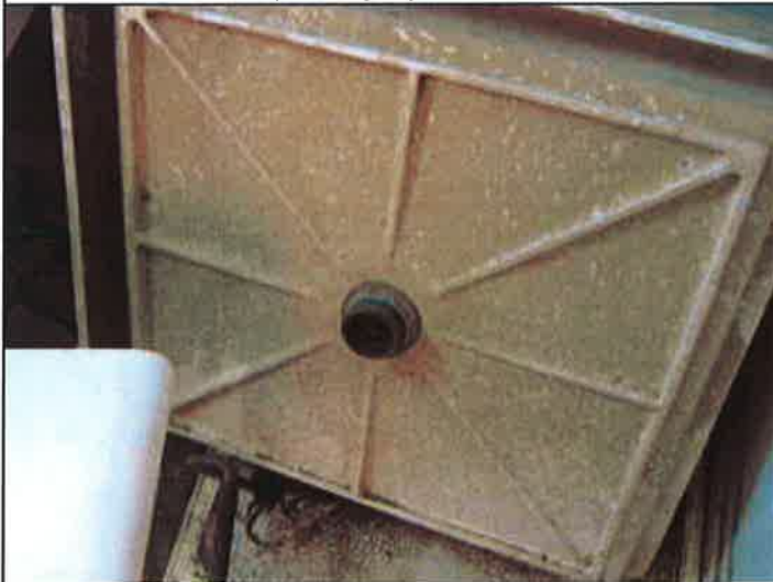
02/05/15 - Substandard Structure - NOD#1,2,3,4,14,17 - Pike
