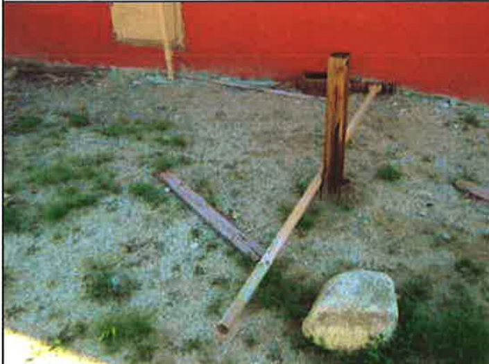
02/05/15 - Substandard Structure - NOD# 4 - Pike
