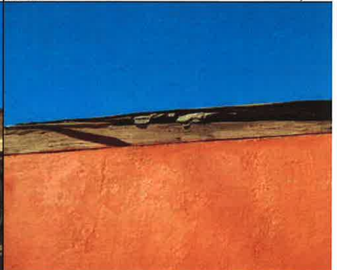
02/05/15 - Substandard Structure - NOD#11,12,13,14,17 - Pike
