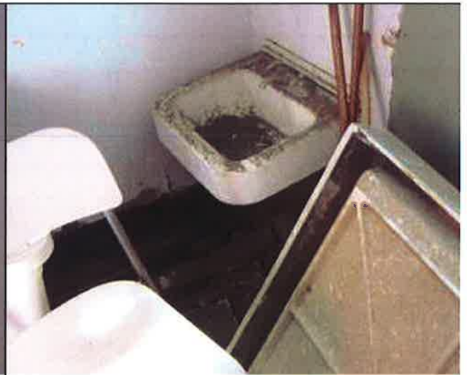
02/05/15 - Substandard Structure - NOD# 1,2,3,4,14,17 - Pike
