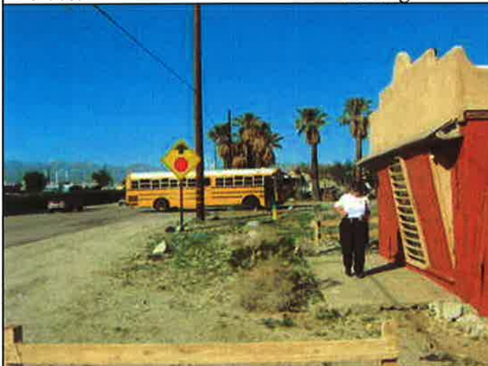
02/05/15 - Substandard Structure - Bus Stop Area - Pike
