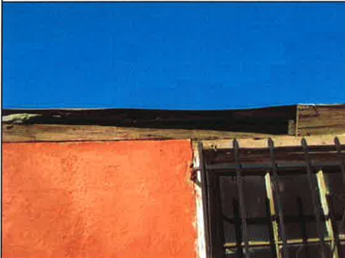
02/05/15 - Substandard Structure - NOD# 11,12,13,14,17- Pike
