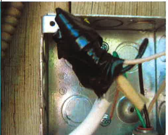
02/05/15 - Substandard Structure - NOD# 6,14,15
