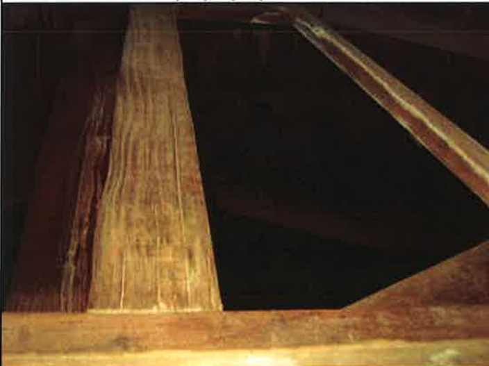
02/05/15 - Substandard Structure - NOD#11,12,13,14,17 - Pike
