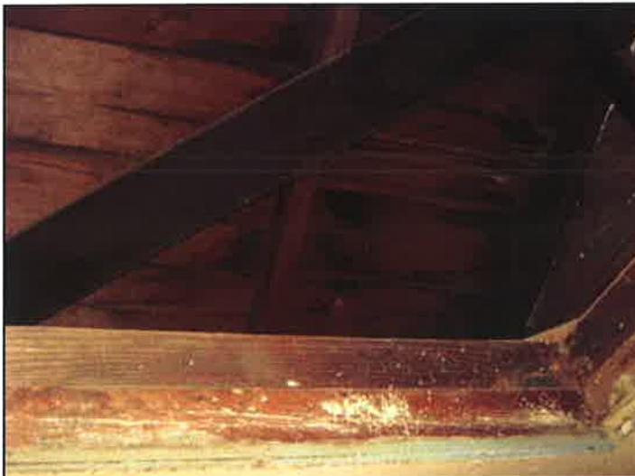
02/05/15 - Substandard Structure - NOD#11,12,13,14,17 - Pike
