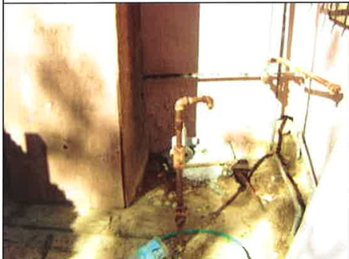
02/05/15 - Substandard Structure - NOD# 7,13,14,17 - Pike
