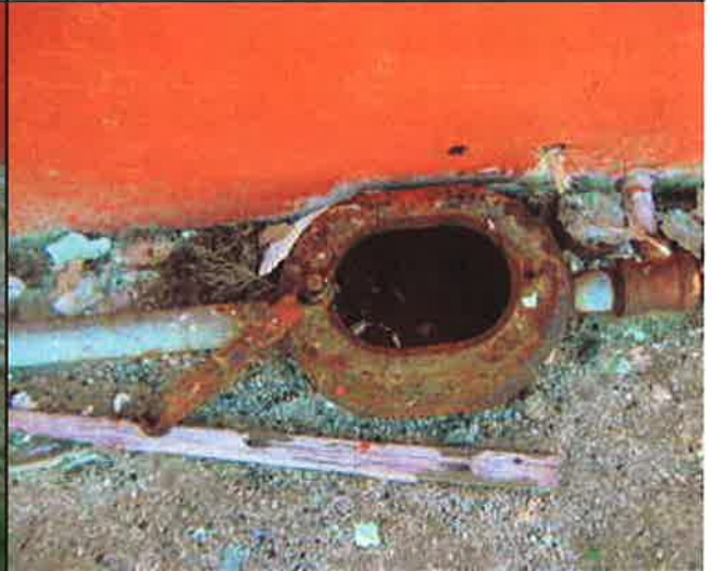
02/05/15 - Substandard Structure - NOD# 4 - Pi
