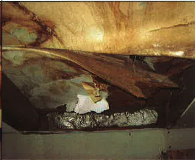
02/05/15 - Substandard Structure - NOD# 11,12,13,14,17 - Pike
