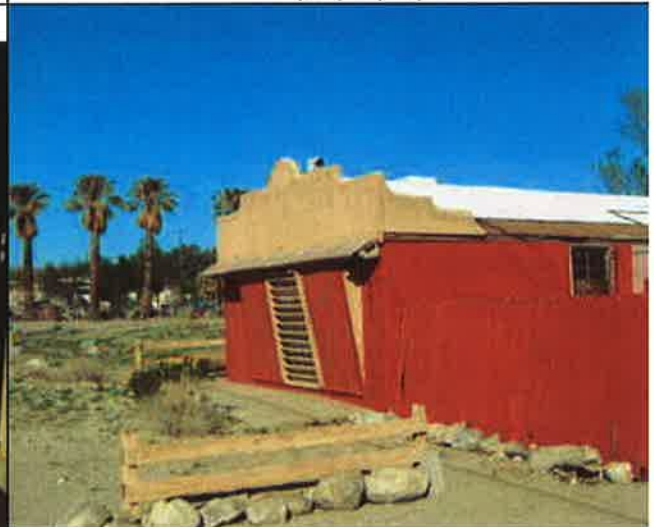
02/05/15 - Substandard Structure - NOD#11,12,13,14,17 - Pike
