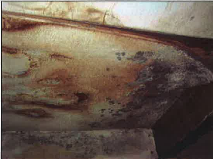
02/05/15 - Substandard Structure - NOD# 11,12,13,14,17 - Pike
