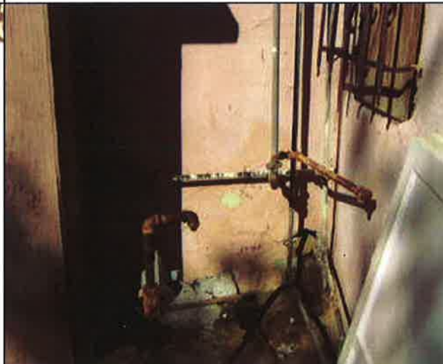
02/05/15 - Substandard Structure - NOD#7,13,14, Pike
