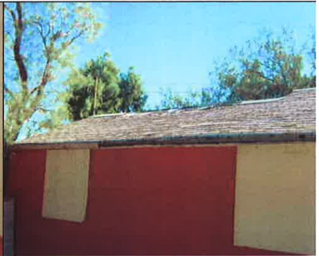
02/05/15 - Substandard Structure - NOD# - Pik
