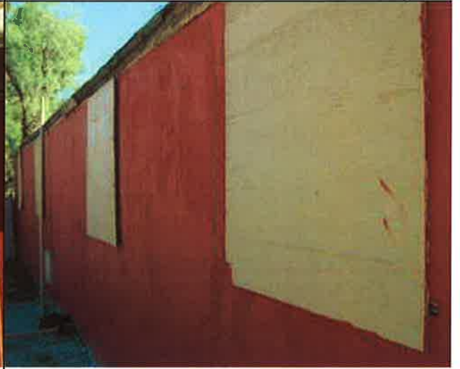
02/05/15 - Substandard Structure - NOD# 17 - P
