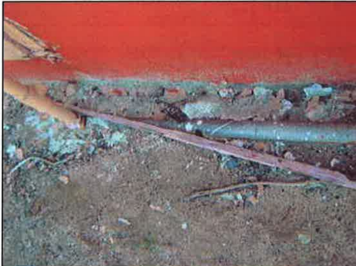
02/05/15 - Substandard Structure - NOD# 4 - Pike
