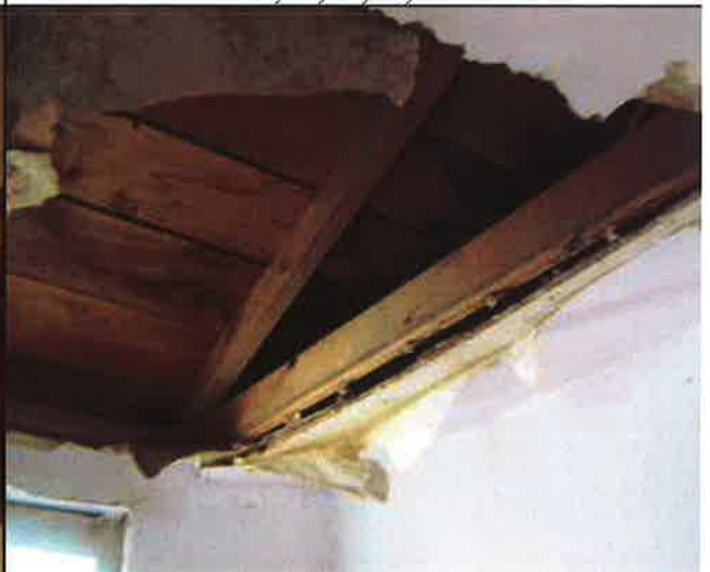
02/05/15 - Substandard Structure - NOD#11,12,13,14,17 - Pike
