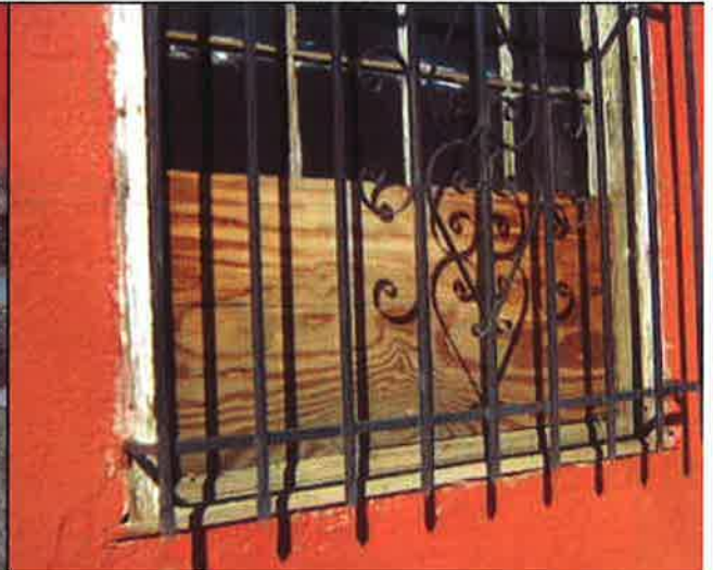
02/05/15 - Substandard Structure - NOD# 12,17 -
