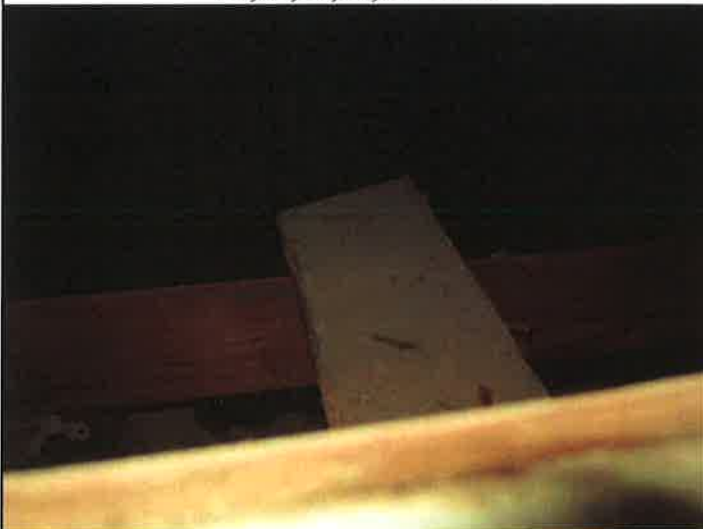
02/05/15 - Substandard Structure - NOD#11,12,13,14,17 - Pike
