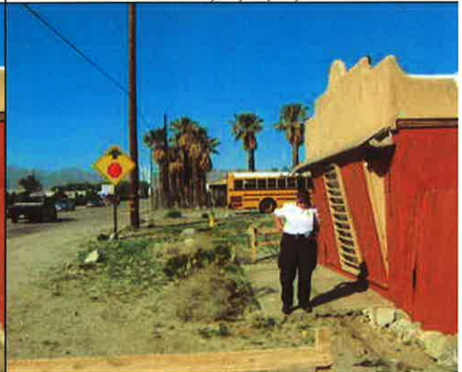
02/05/15 - Substandard Structure - Bus Stop Area Pike
