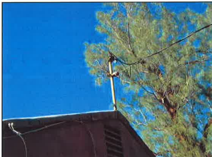
02/05/15 - Substandard Structure - NOD# 6,14,15,17 - Pike
