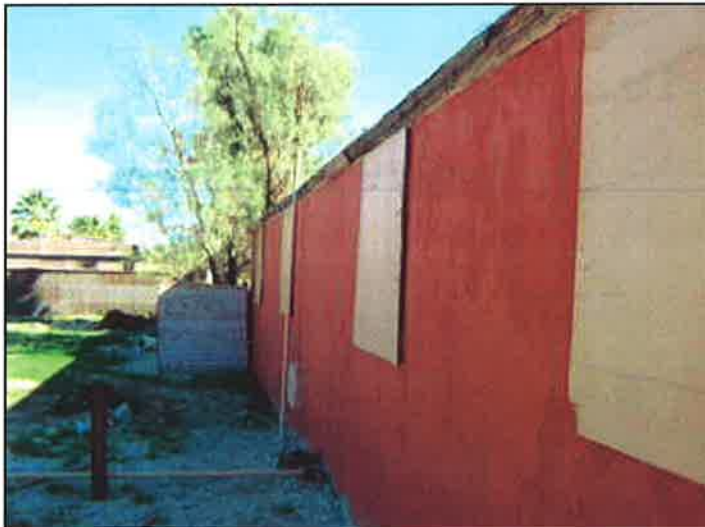
02/05/15 - Substandard Structure - NOD# 17 - Pike
