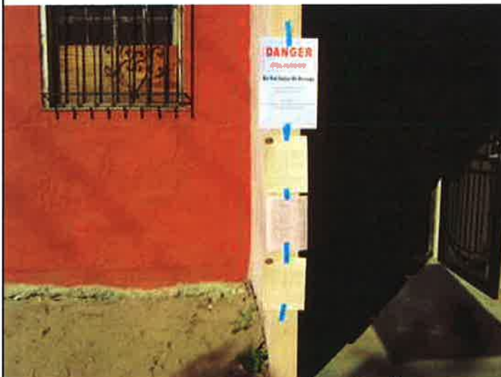
02/05/15 - Substandard Structure - Posting - Pike
