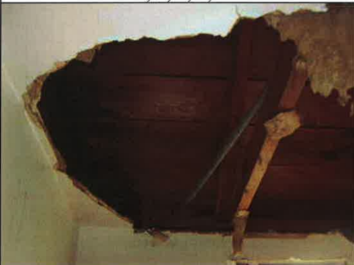
02/05/15 - Substandard Structure - NOD# 11,12,13,14,17 - Pike
