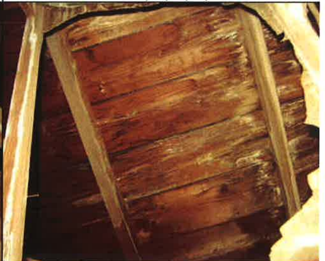
02/05/15 - Substandard Structure - NOD#11,12,13,14,17 - Pike
