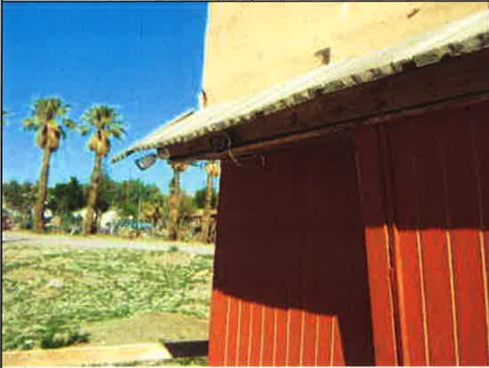
02/05/15 - Substandard Structure - NOD#17 - Pike
