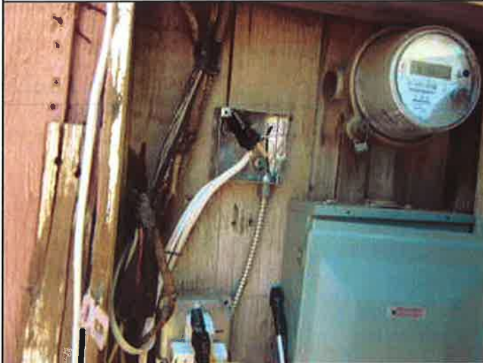
02/05/15 - Substandard Structure - NOD# 6,14,15,17 - Pike
