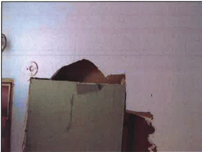
02/05/15 - Substandard Structure - NOD# 11,12,13,14,17 - Pike
