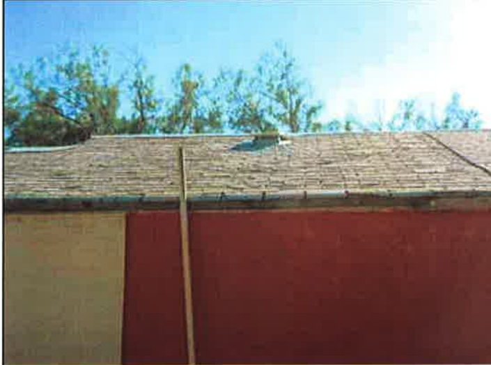
02/05/15 - Substandard Structure - NOD# 17 - Pike
