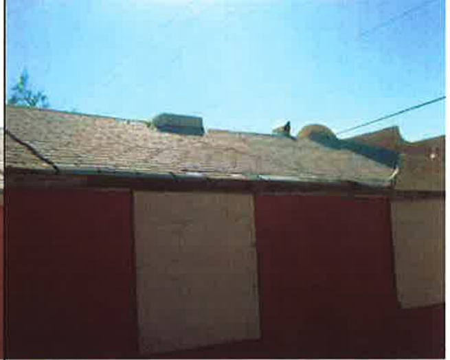
02/05/15 - Substandard Structure - NOD# 17 - P
