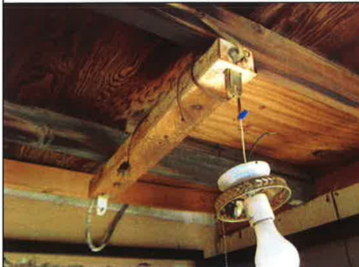
02/05/15 - Substandard Structure - NOD#6,14,15,17 - Pike
