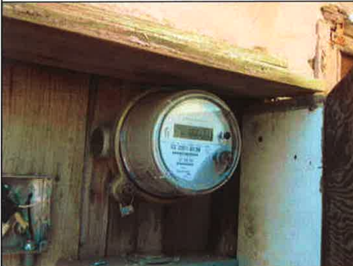
02/05/15 - Substandard Structure - NOD# 6,14,15,17 - Pike
