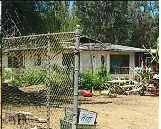
Structure remains substandard-JMorris 7/28/15
