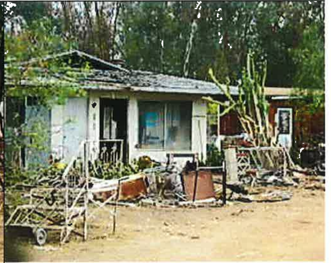
Structure remains substandard-JMorris 5/6/15
