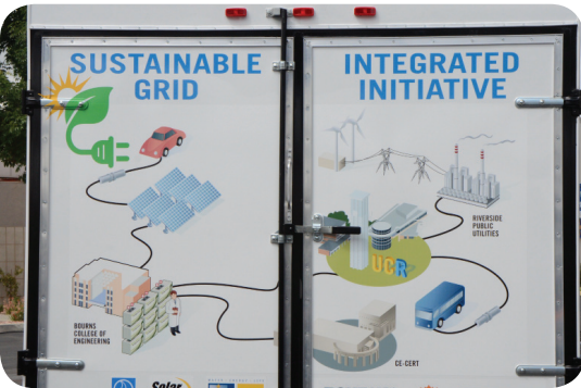
0.5MW Mobile Battery System
