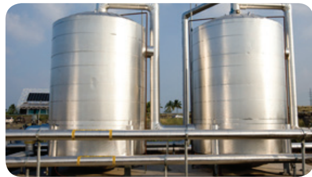
UCR Thermal Energy Storage (TES) Tanks
