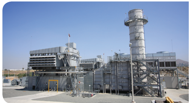
RPU's Natural Gas Peaker Plant
