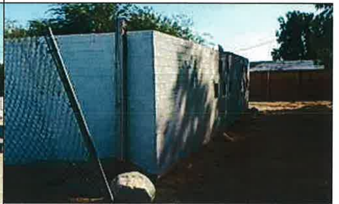
Substandard Block Wall 12/23/15 J. Cole
