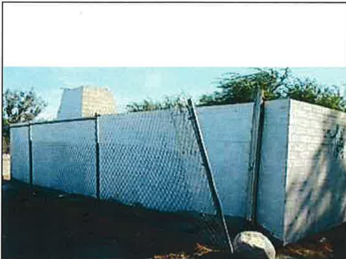
Substandard Block Wall 12/23/15 J. Cole
