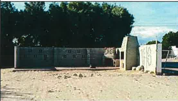
Substandard Block Wall 12/23/15 J. Cole
