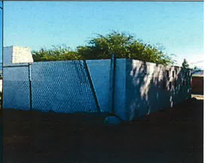
Substandard Block Wall 11/19/15 J. Cole
