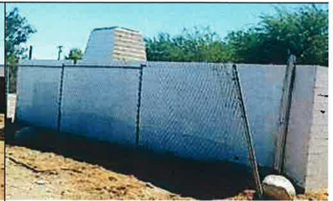
Substandard Wall 10/9/15 J. Cole
