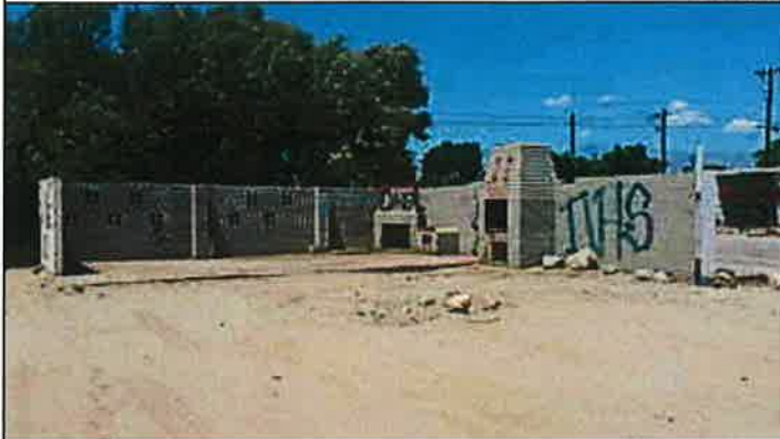
Substandard Block Wall 8/14/15 J. Cole
