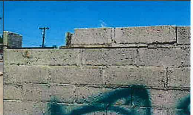
Cracks in the Block Wall 8/14/15 J. Cole
