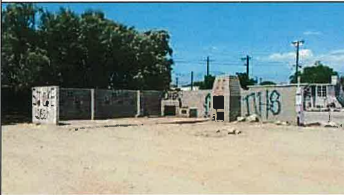
Substandard Block Wall 8/14/15 J. Cole
