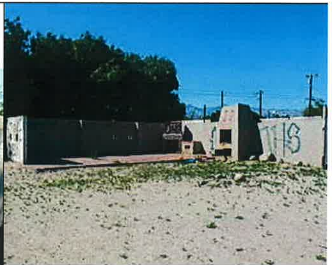
Substandard Block Wall 2/25/16 J. Cole
