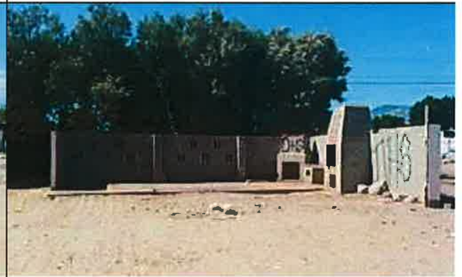
Substandard Wall 10/9/15 J. Cole
