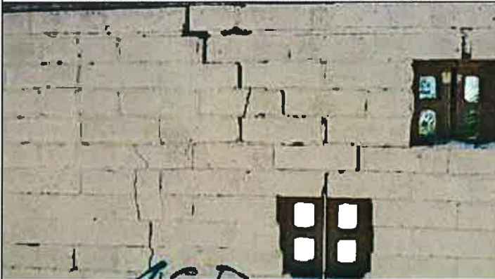
Cracks in the Block Wall 8/14/15 J. Cole
