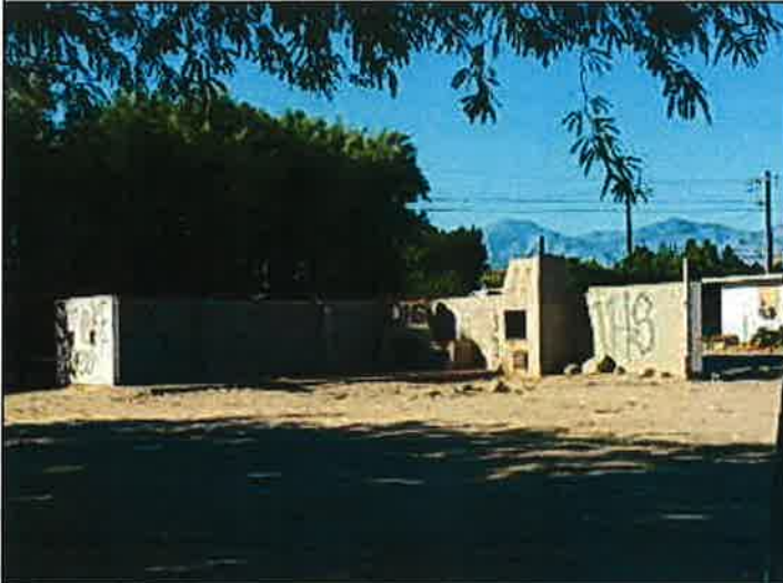
Substandard Block Wall 11/19/15 J. Cole
