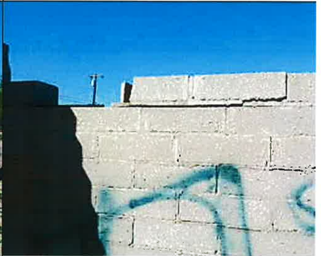
Cracks in the Wall, Graffiti 2/25/16 J. Cole
