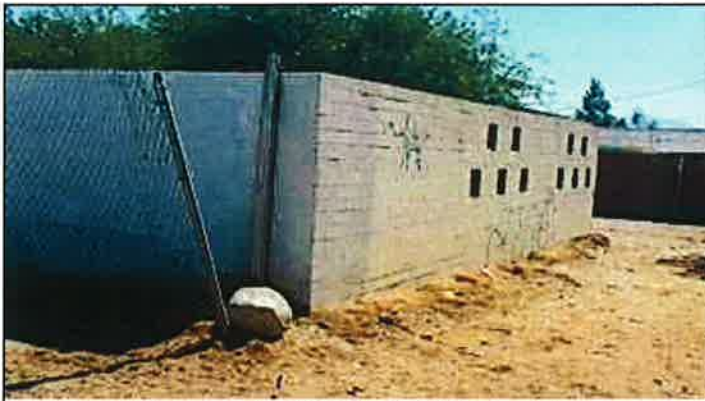
Substandard Wall 10/9/15 J. Cole
