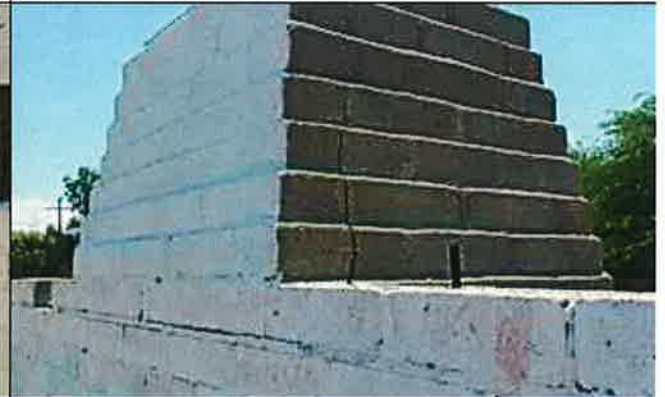
Cracks in the Block Wall 8/14/15 J. Cole
