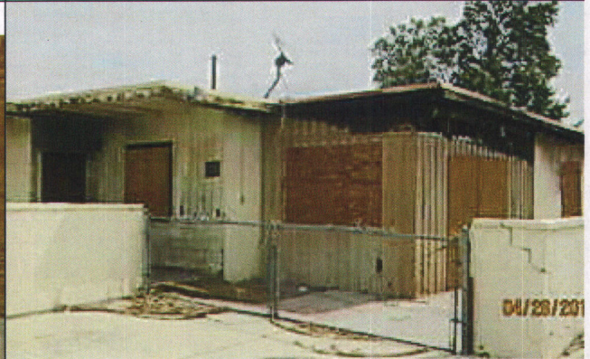
Structure remains substandard, burnt & boarded u of 6.
