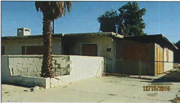
No changes, structure remains boarded up. 1 of 3.
