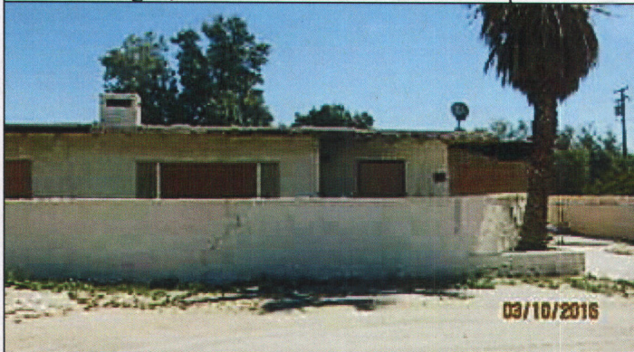
Structure remains substandard, burnt, boarded up and free of trash. 1 of 8.
