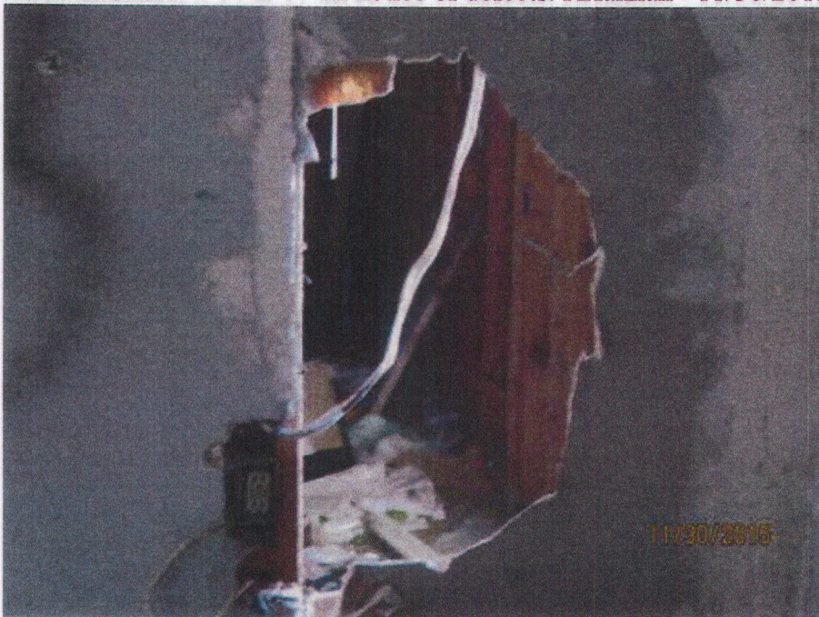
Inside structure. # 14 & 17 on notice of defects. RHannah - 11/30/2015
