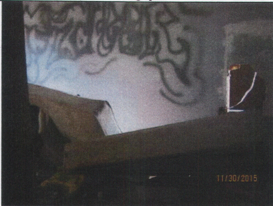
Inside structure. # 14 & 17 on notice of defects. RHannah - 11/30/2015
