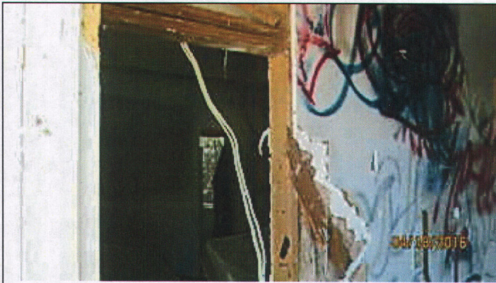
Substandard structure and accumulated rubbish remains unchanged. 1 of 8.
