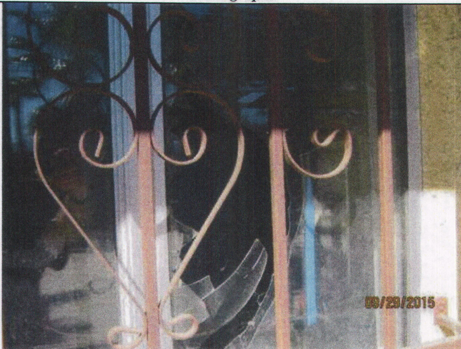
Broken window*, # 14 & 17 on notice of defects. RHannah - 09/29/2015
