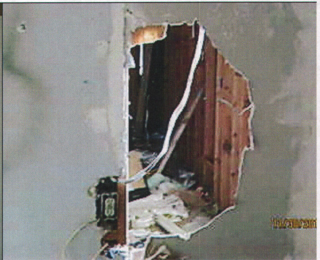
Inside structure. # 14 & 17 on notice of defects RHannah
