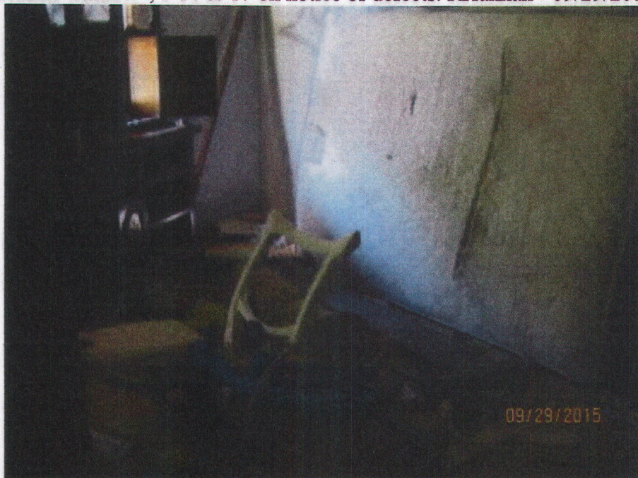
Inside structure*. # 14 & 17 on notice of defects. RHannah - 09/29/2015
