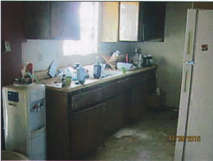
Inside structure'. # 14 & 17 on notice of defects. RHannah
