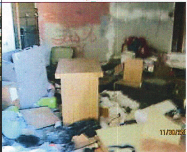
Inside structure!. # 14 & 17 on notice of defect. RHannah
