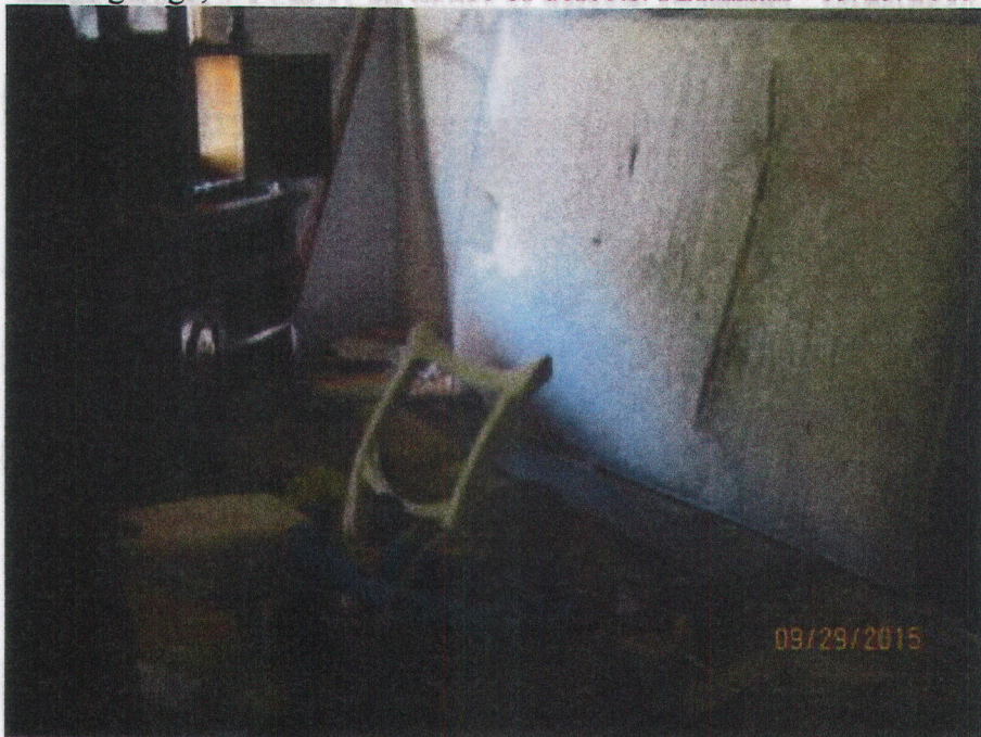
Inside structure. # 14 & 17 on notice of defects. RHannah - 09/29/2015
