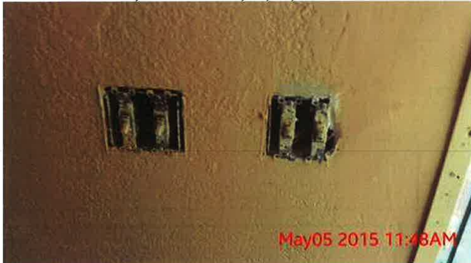
E. Torres; SS2- defects 6, 14, 17, 19 - 05/05/2015
