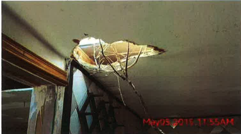
E. Torres; SS1- defects 11, 12, 13, 14, 17, 19 - 05/05/2015
