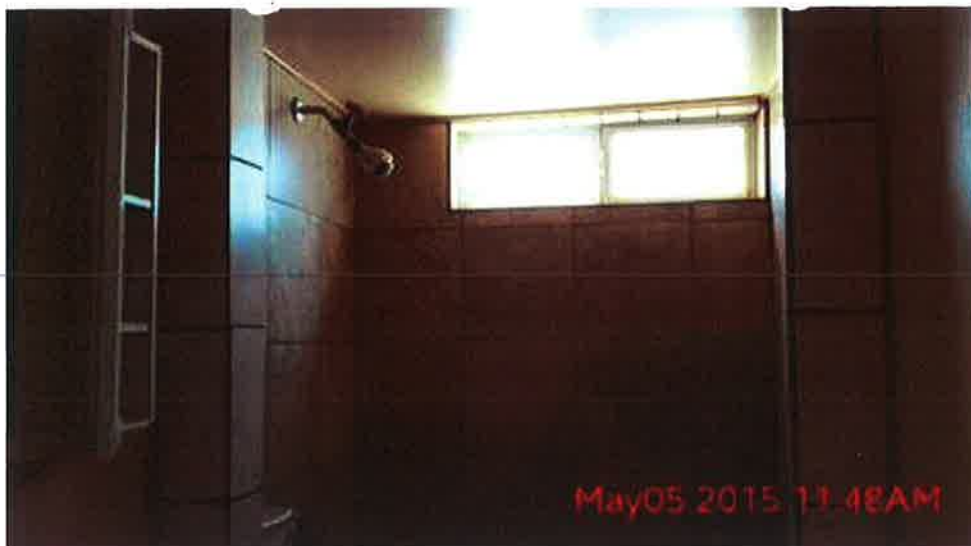
E. Torres; SS2- defects 1, 2, 4, 17, 19 - 05/05/2015
