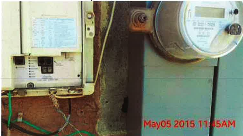
E. Torres; newer electric service panel - 05/05/2015
