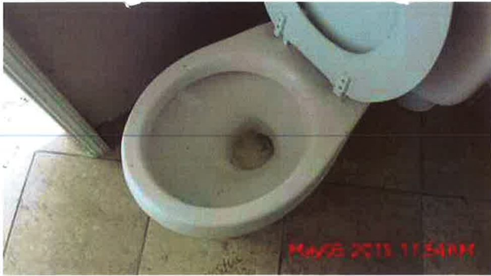
E. Torres; SS1- defects 1, 2, 14, 17 - 05/05/2015
