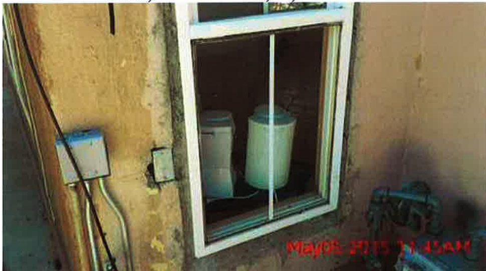
E. Torres; SS1- defects 10, 13, 14, 17, 19 - 05/05/2015
