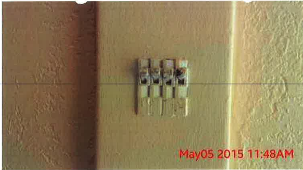
E. Torres; SS2- defects 6, 14, 17, 19 - 05/05/2015
