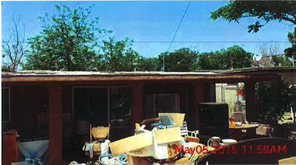
E. Torres; SS1- defects 14, 17, 19 - 05/05/2015
