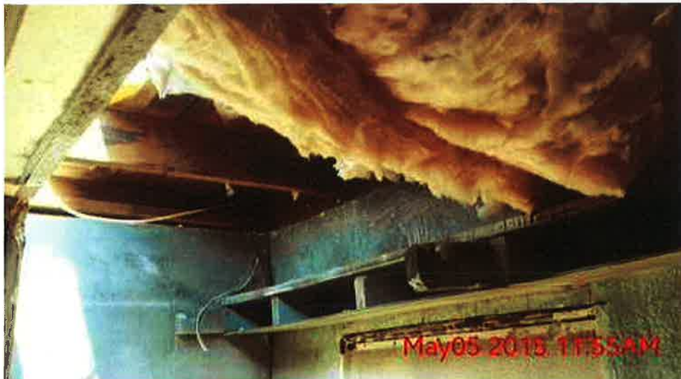
E. Torres; SS1- defects 11, 12, 13, 14, 17, 19 - 05/05/2015
