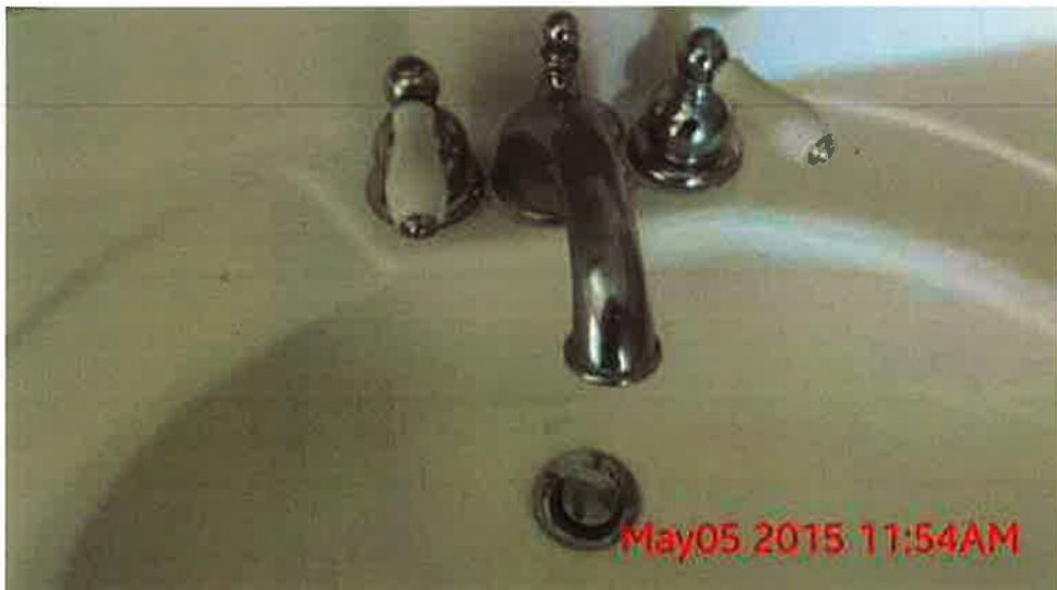
E. Torres; SS1- defects 1, 2, 14, 17 - 05/05/2015
