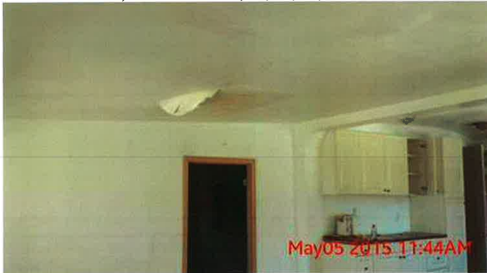
E. Torres; SS1- defects 11, 12, 13, 14, 17, 19 - 05/05/2015
