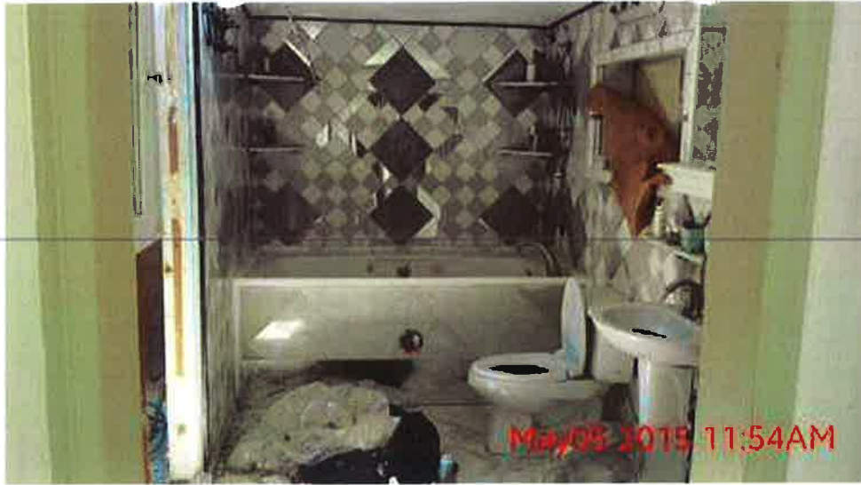
E. Torres; SS1- defects 13, 14, 17, 19 - 05/05/2015
