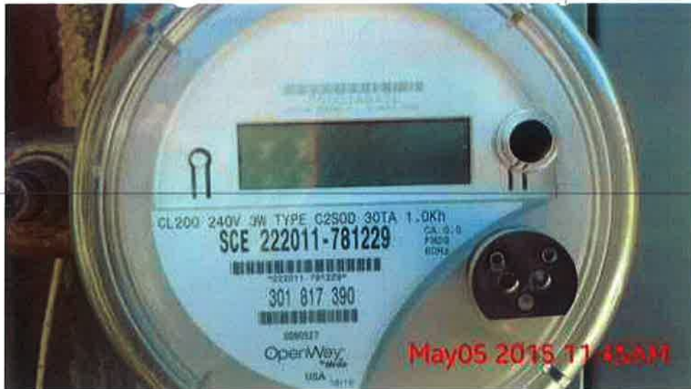
E. Torres; electric meter - 05/05/2015
