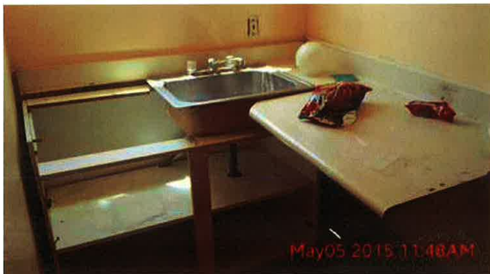
E. Torres; SS2- defects 1, 2, 4, 17, 19 - 05/05/2015
