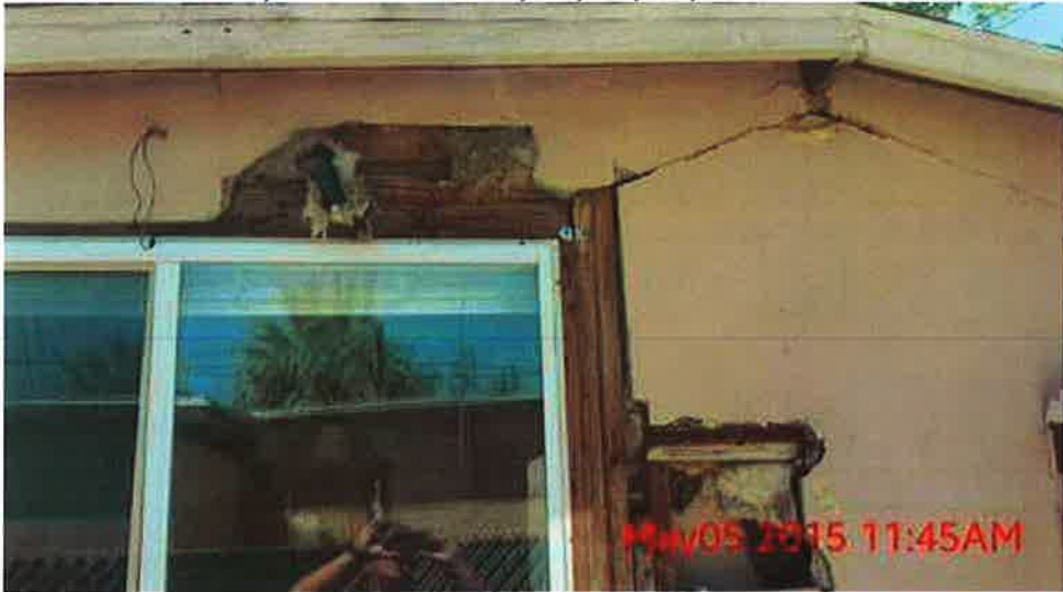
E. Torres; SS1- defects 10, 13, 14, 17, 19 - 05/05/2015
