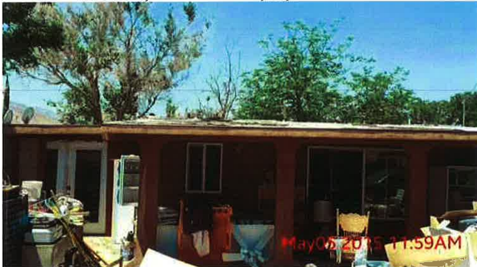
E. Torres; SS1- defects 14, 17, 19 - 05/05/2015
