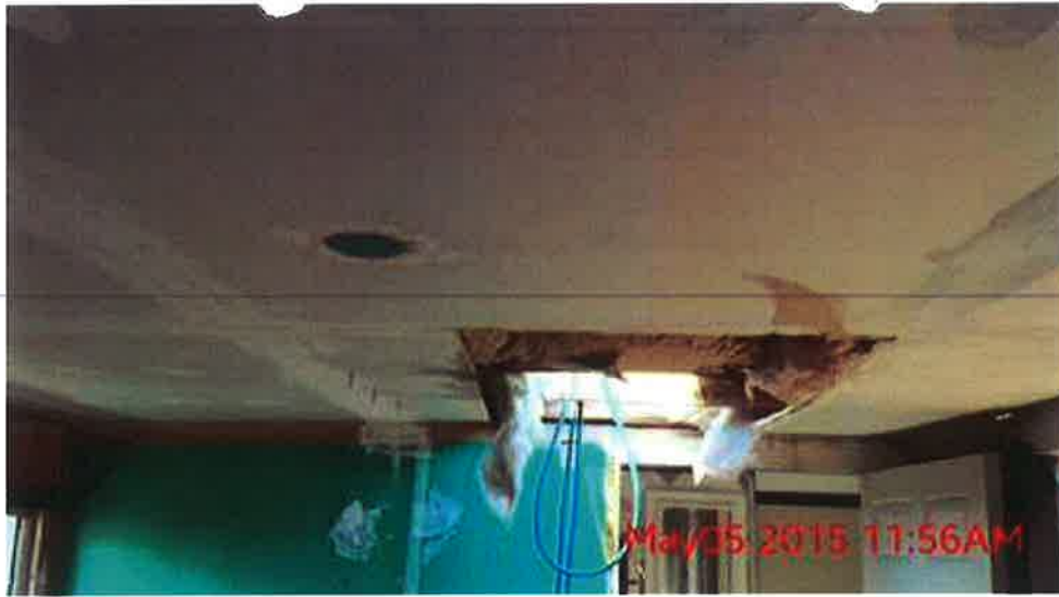
E. Torres; SS1- defects 11, 12, 13, 14, 17, 19 - 05/05/2015
