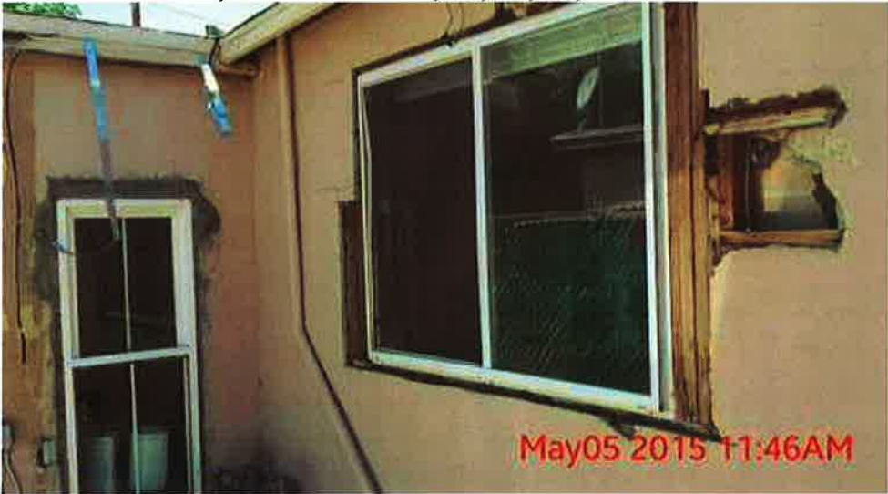
E. Torres; SS1- defects 10, 13, 14, 17, 19 - 05/05/2015
