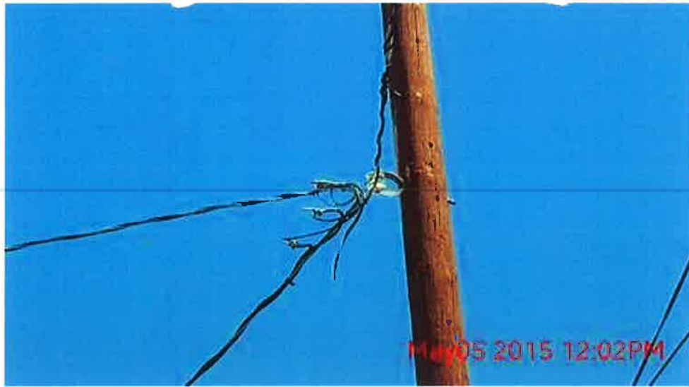
E. Torres; SS 1&2- defects 5 - 05/05/2015
