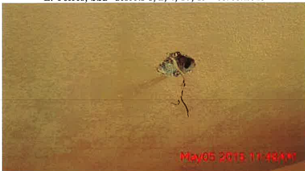
E. Torres; SS2- defects 5, 6, 11, 15, 17, 19 - 05/05/2015
