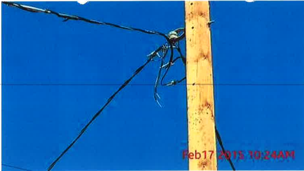
E. Torres; power to property pulled by Edison - 02/17/2015
