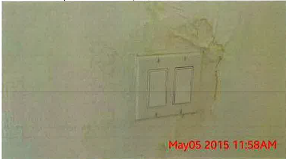
E. Torres; SS1- defects 6, 12, 13, 14, 17, 19 - 05/05/2015
