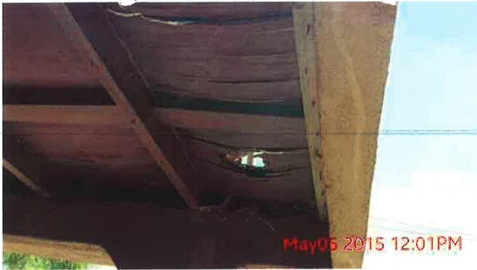
E. Torres; SS1- defects 11, 13, 14, 17, 19 - 05/05/2015
