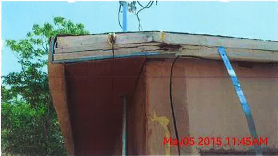
E. Torres; SS1- defects 11, 13, 14, 17, 19 - 05/05/2015
