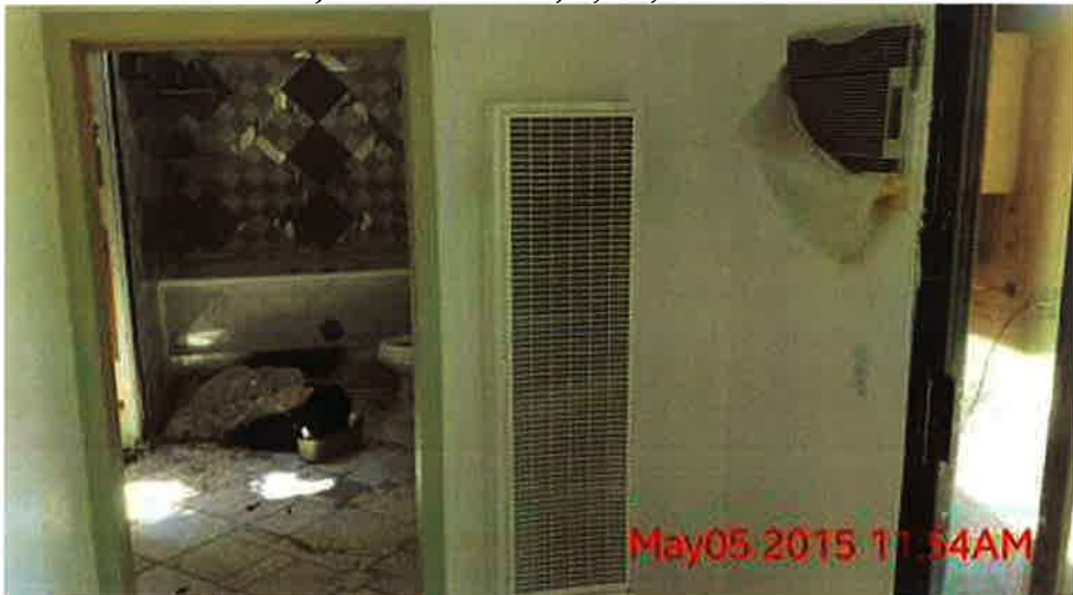
E. Torres; SS1- defects 13, 14, 17, 19 - 05/05/2015
