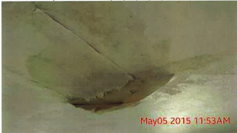
E. Torres; SS1- defects 11, 12, 13, 14, 17, 19 - 05/05/2015
