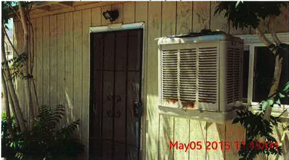
E. Torres; SS2- defects 13, 14, 17, 19 - 05/05/2015
