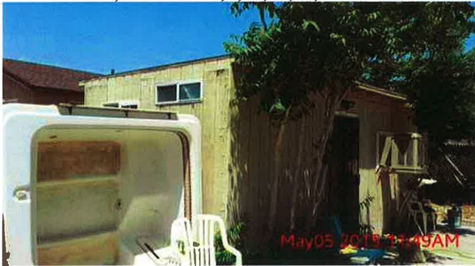
E. Torres; SS2- defects 10, 13, 14, 17, 19 - 05/05/2015
