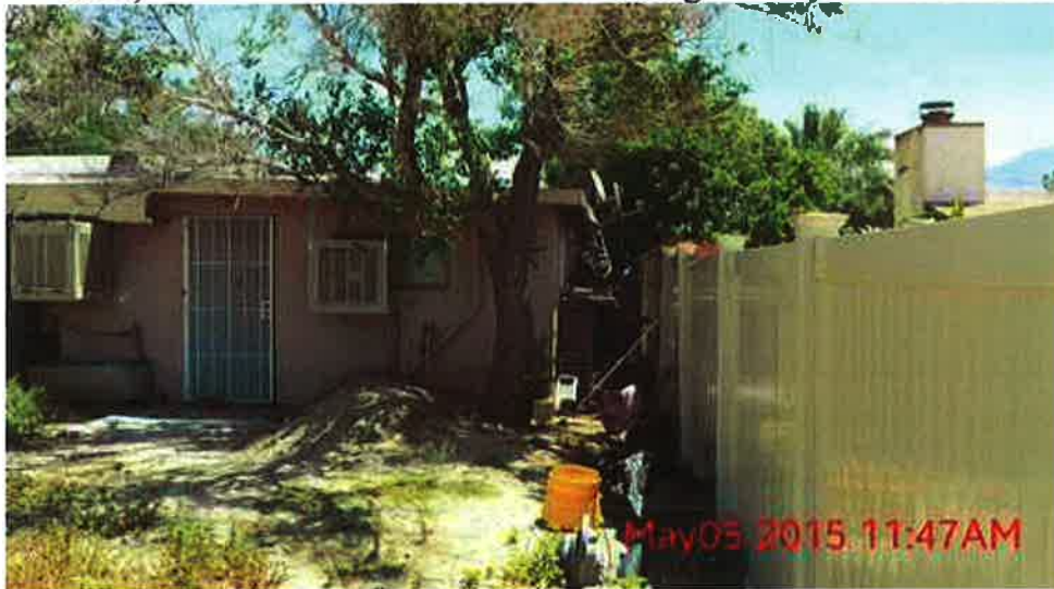
E. Torres; substandard structure #1- defects - 05/05/2015
