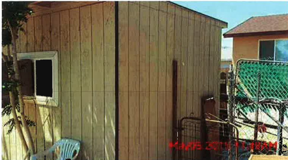
E. Torres; SS2- defects 13, 14, 17, 19 - 05/05/2015
