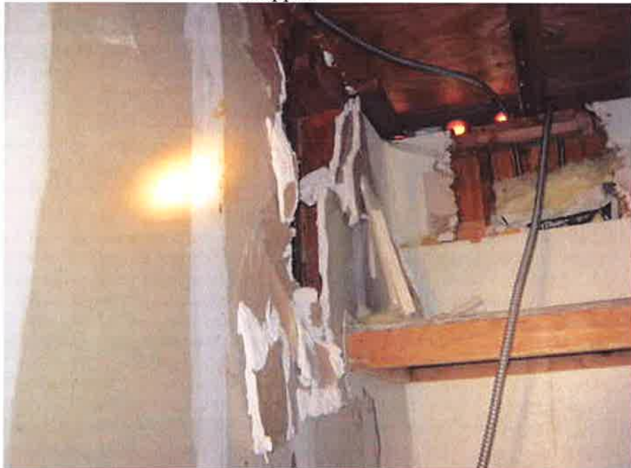
110215 TM damaged drywall - 11/03/2015
