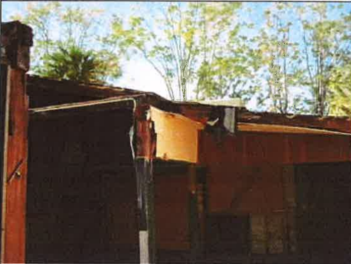
110215 TM missing roof section
