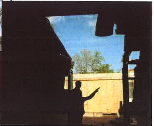
110215 TM missing wall and roof
