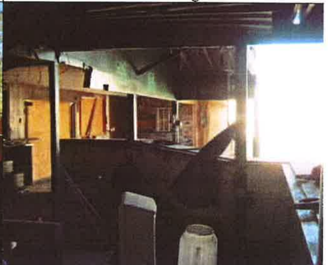
110215 TM missing wall and roof
