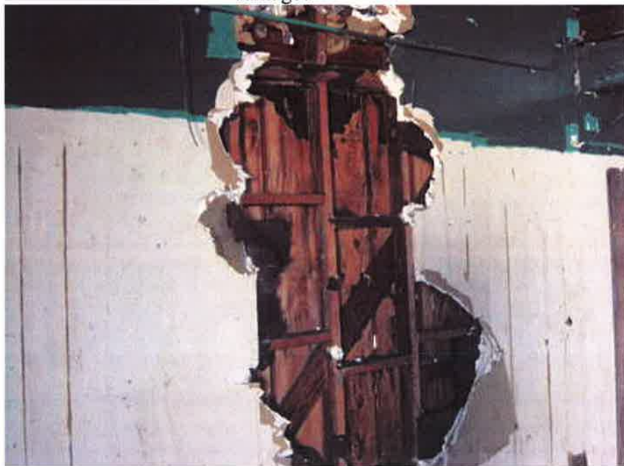
110215 TM damaged exterior wall - 11/03/2015
