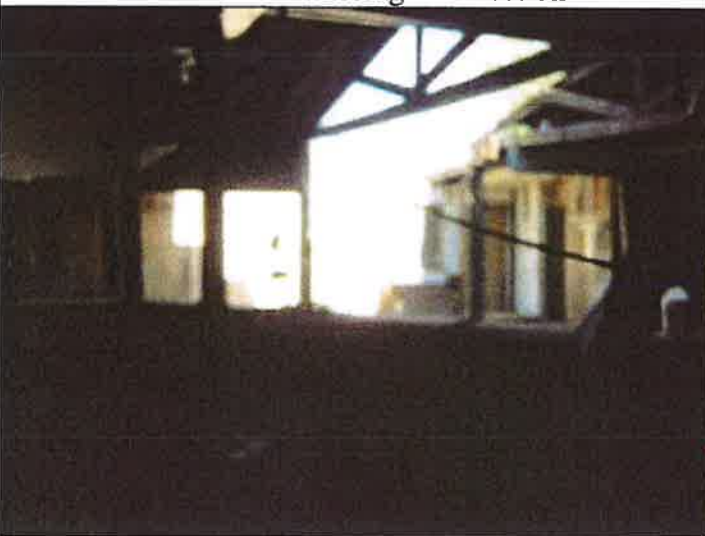
110215 TM missing wall and roof
