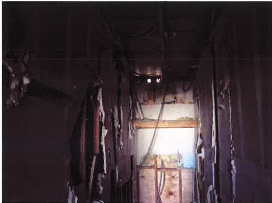
110215 TM damaged interiors - 11/03/2015
