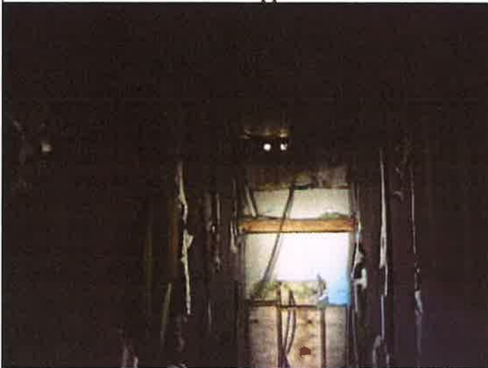
110215 TM damaged interiors
