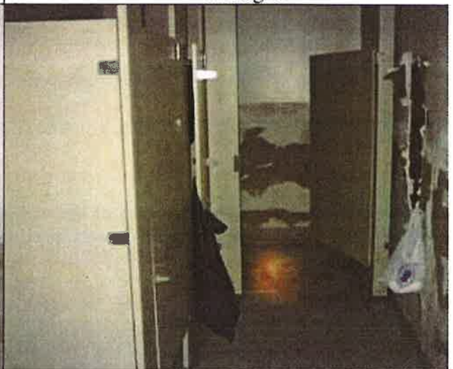
110215 TM damaged bathroom
