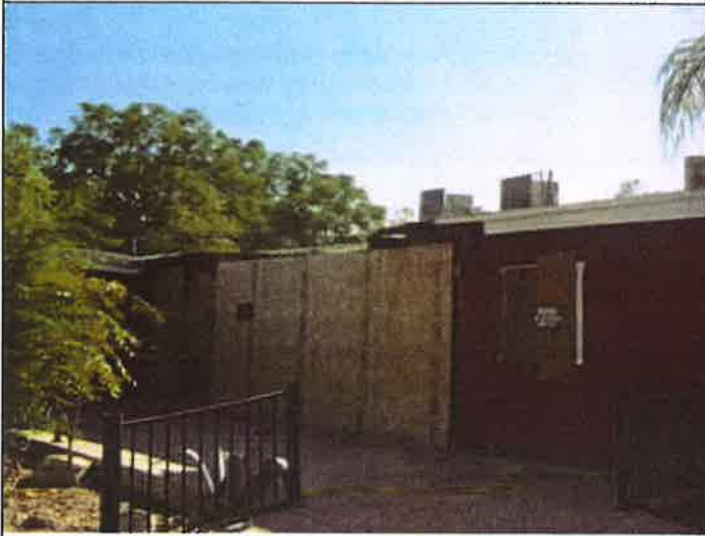
110215 TM lack of exterior wall
