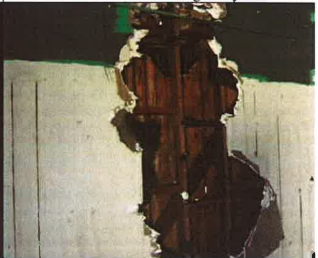
110215 TM damaged exterior wall
