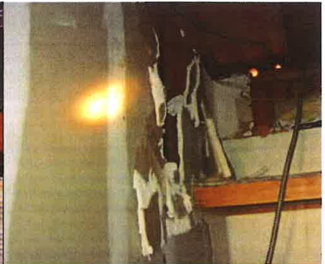
110215 TM damaged drywall
