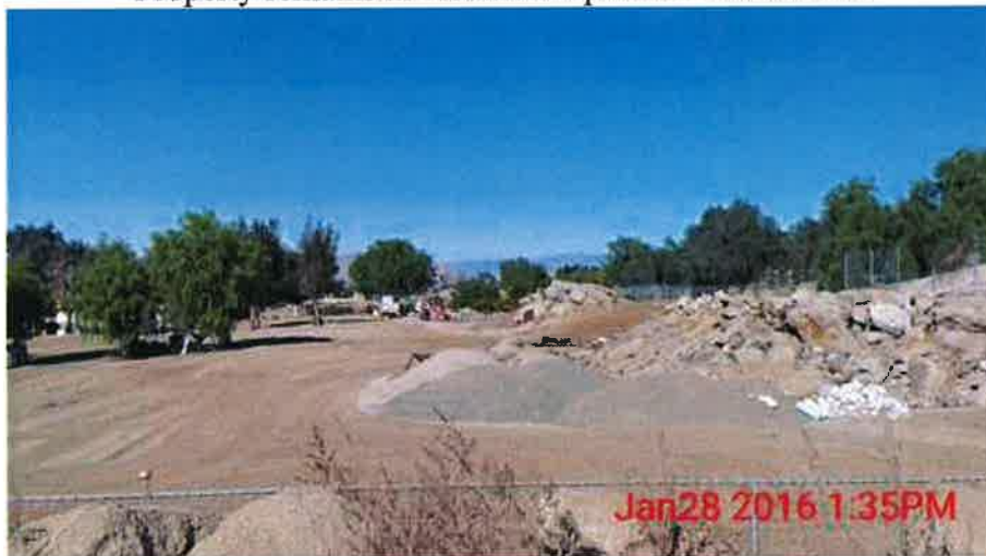
site remains in violation - 01/28/2016
