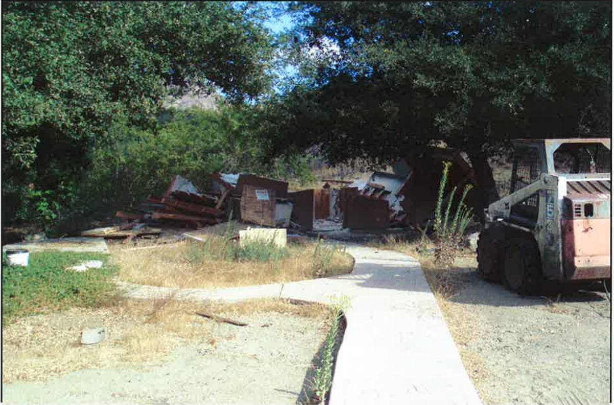
PHOTO # _ 1 _ DATE: _ 09/15/09 _ TIME: _ 0900 AM TAKEN BY: BF # 21 Depicting demolished sub-standard two-story structure _____
