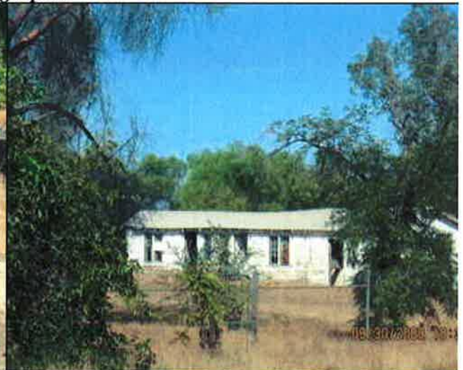
Taken by J. Wagner #80 Substandard structure remains.
