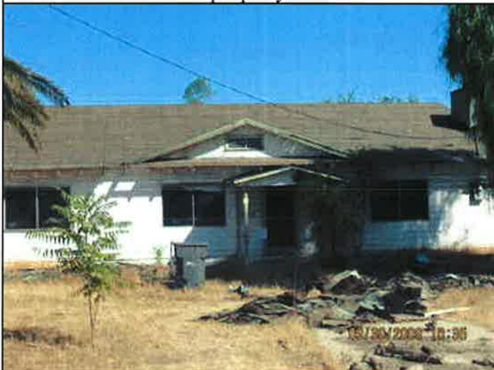
Taken by J. Wagner #80 Substandard home remains on property.
