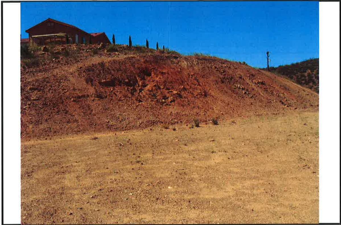
PHOTO # 3 DATE: 07/07/09 TAKEN BY: J. Pike #59 NOTES: Eastern side of the property is eroding from the rains.
