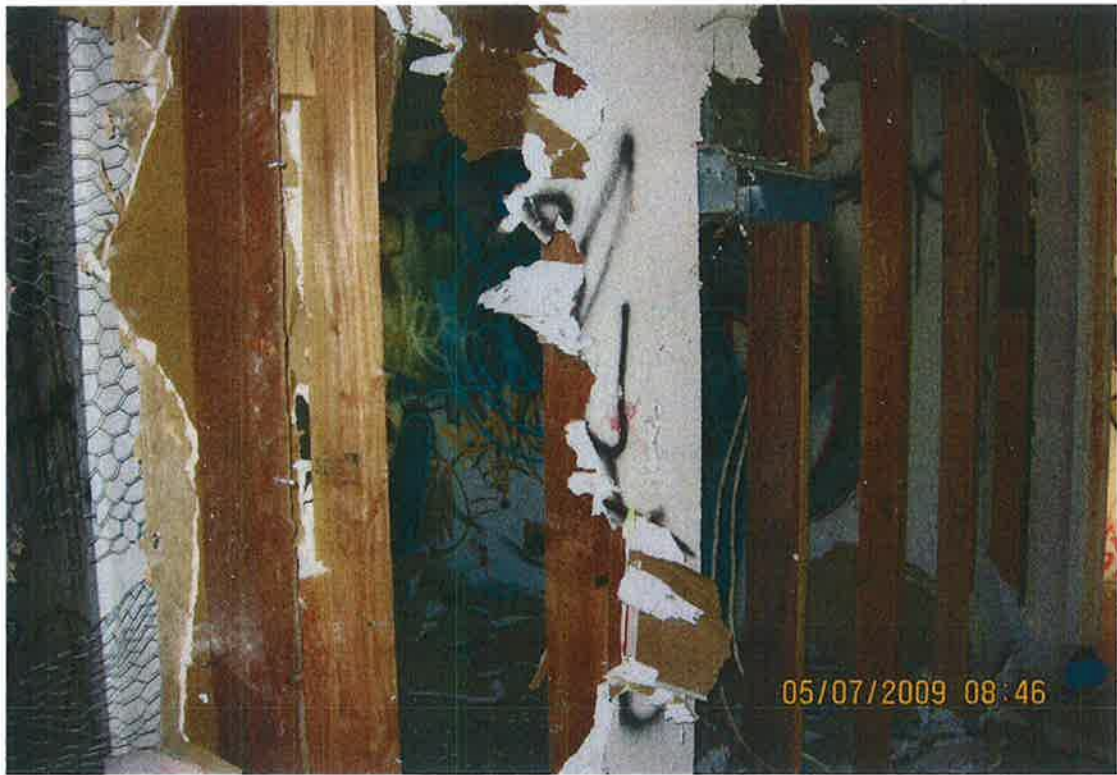
KITCHEN WALLS RIPPED OUT NO CABINETS OR PLUMBING LEFT IN THE KITCHEN
