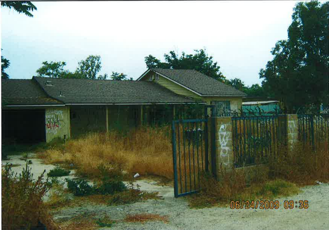
THIS IS THE WEST FRONT SIDE OF THE PROPERTY FROM CHANDLER STREET GRAFFITI STILL COVERING THE RESIDENCE AND BLOCK PILLARS TRASH, DEBRIS AND EOS (ILLEGALLY DUMPED ITEMS)
