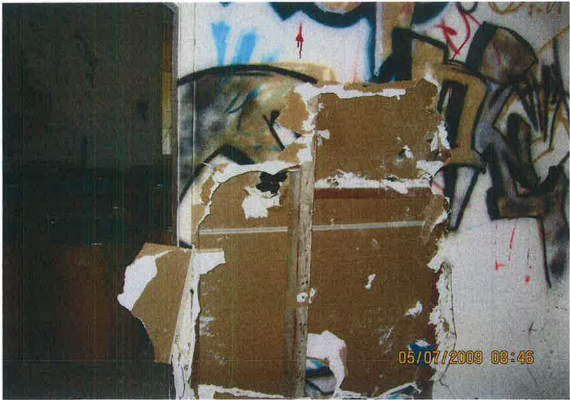
KITCHEN WALL DRYWALL RIPPED FROM THE WALL
