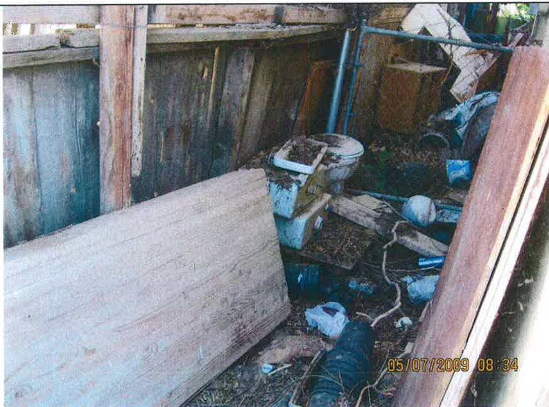
THIS IS THE EXTERIOR AREA JUST WEST OF THE GARAGE AREA IS SO FULL OF EOS AND AR I COULD NOT WALK BACK THERE
