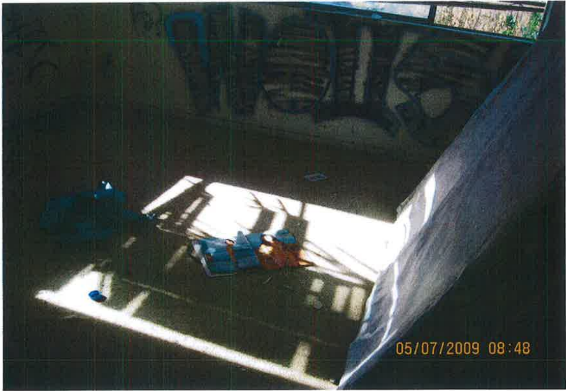
FRONT BEDROOM #3, BROKEN WINDOW, GRAFFITI AND PORNOGRAPHY SCATTERED ABOUT THE ROOM
