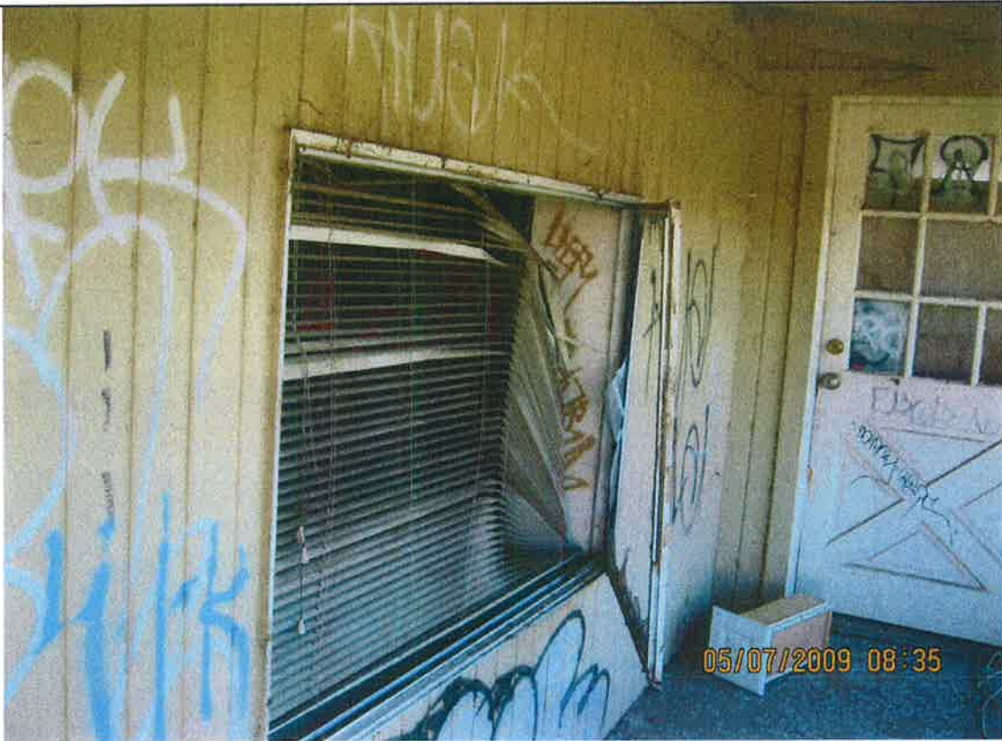
FRONT WINDOW COMPLETELY BROKEN OUT WITH FRAME
