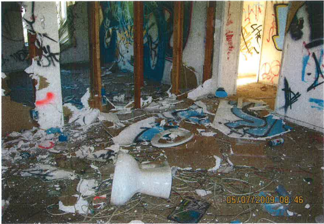
LIVING ROOM - DRYWALL BROKEN OUT MORE GRAFFITI AND A TOILET ON THE FLOOR
