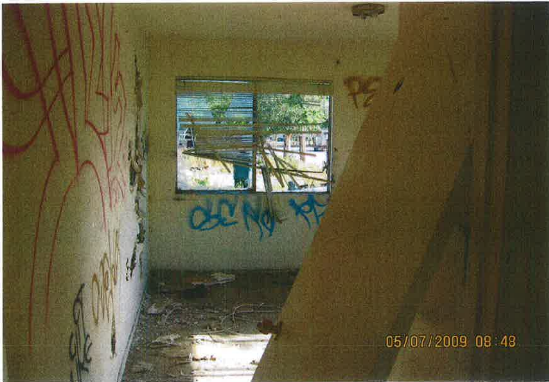
MASTER BEDROOM - BROKEN WINDOW, BROKEN DOOR AND MORE GRAFFITI COVERING THE WALLS
