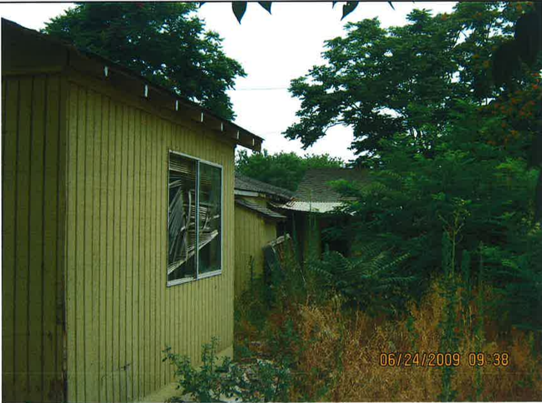
ALL WINDOWS AND DOOR TO PROPERTY ARE BROKEN
