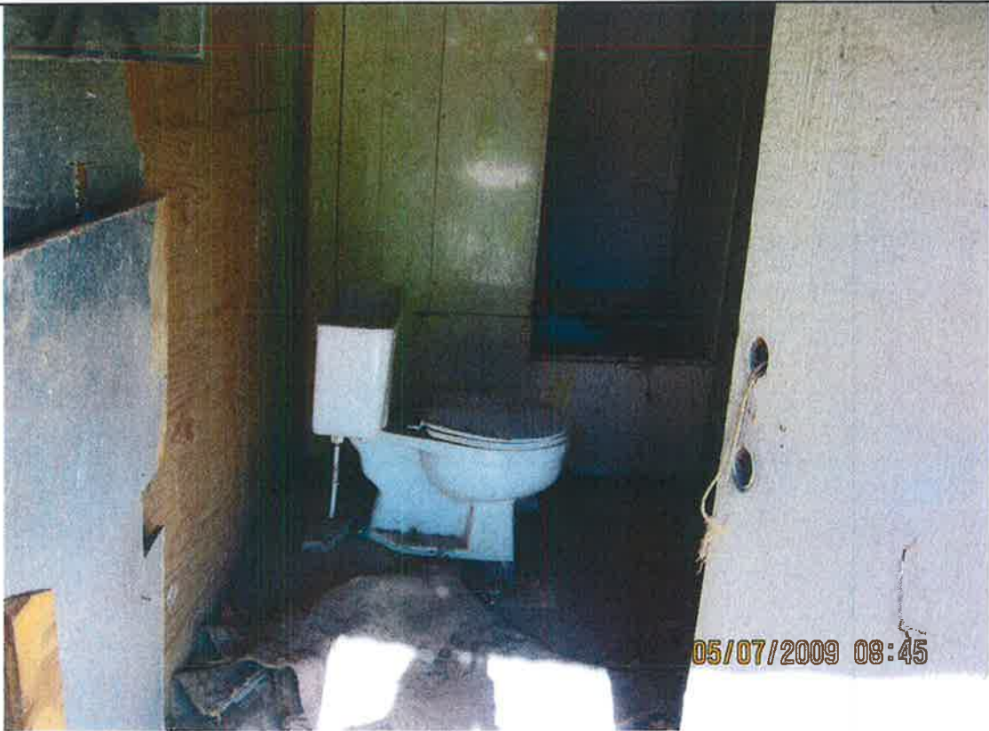
BATHROOM IN THE UNPERMITTED ROOM ADDITION
