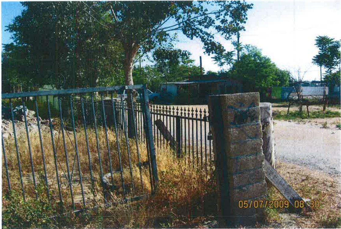
EAST SIDE ENTRY WAY GATE DAMAGED MAKING THE PROPERTY OPEN AND ACCESSIBLE
