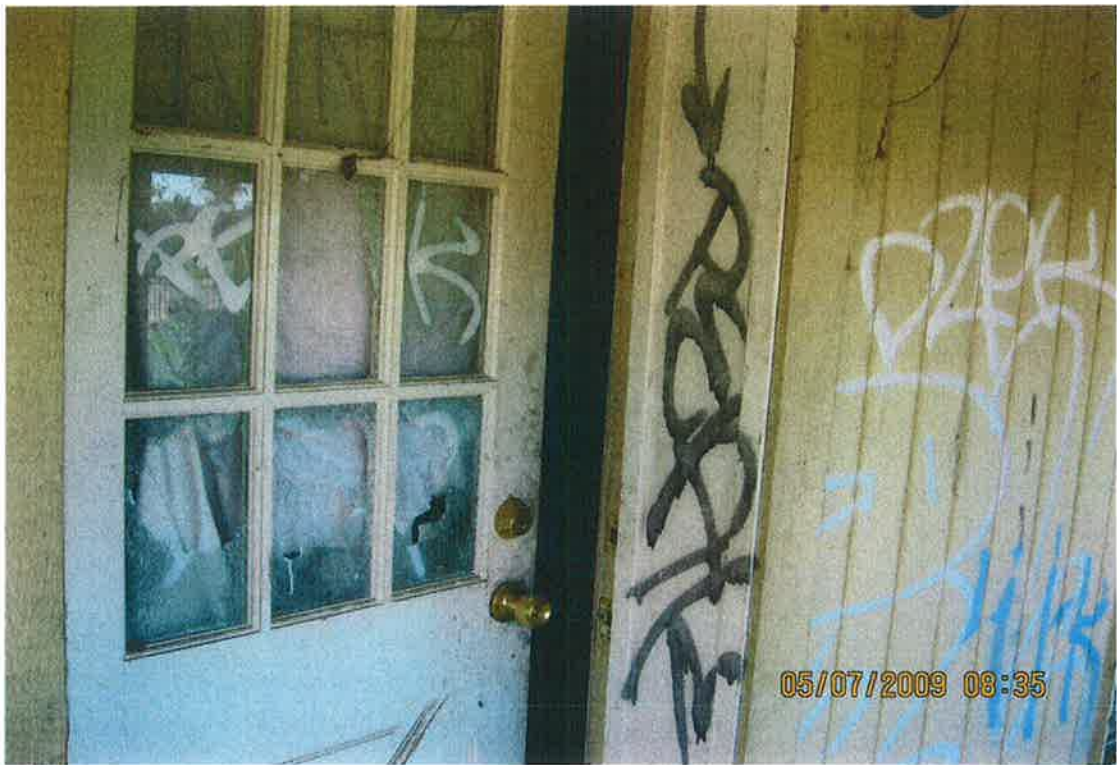
FRONT ENTRY WAY DOOR - DOOR LOCK BROKEN ALONG WITH THE WINDOWS IN THE DOOR
