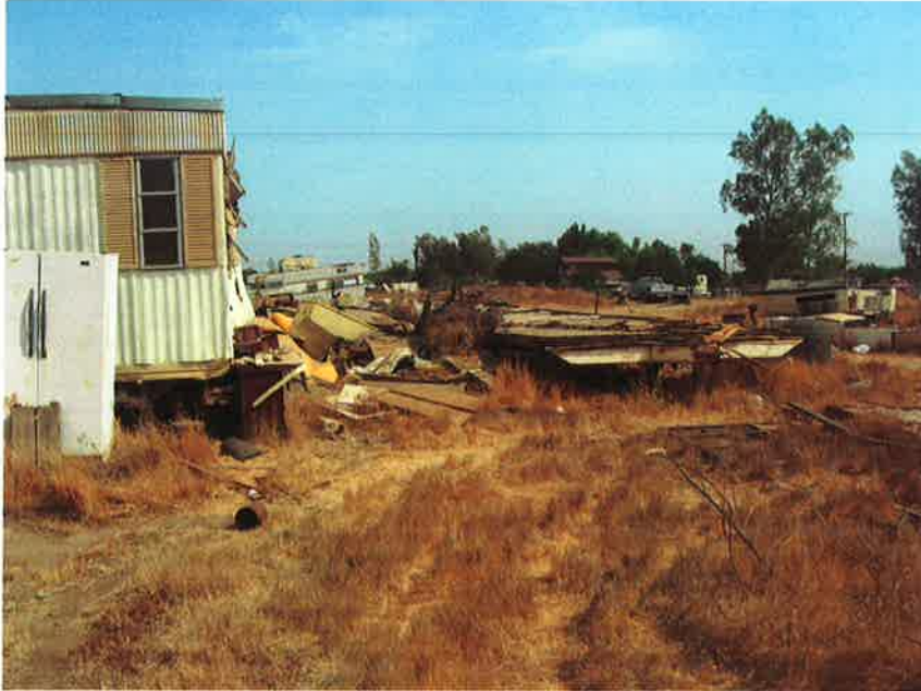
Photo #29 – demolition debris and trash
