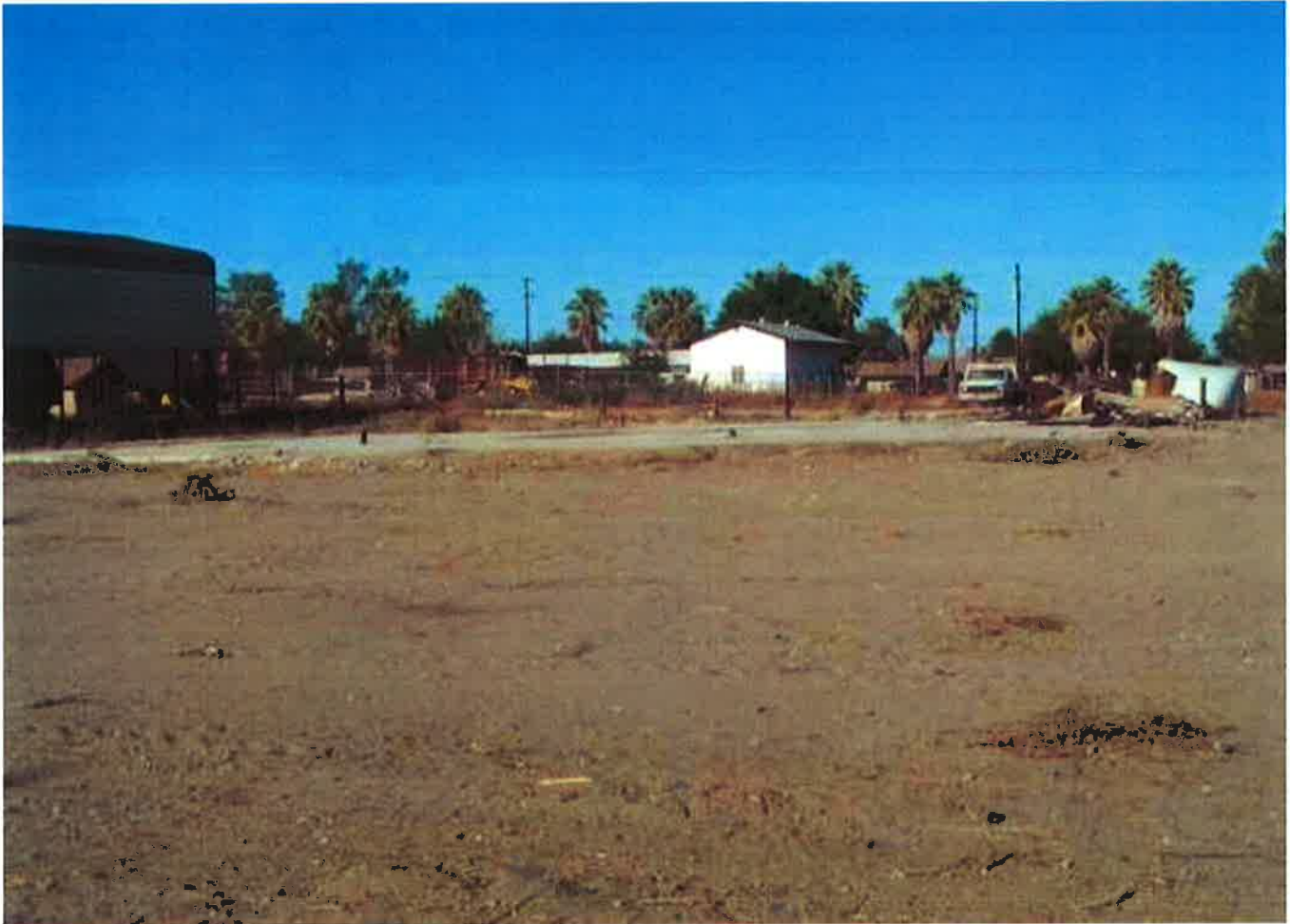
Overview of south end of parcel. A building was dismantled and the pile of rubbish and debris in photo located on right side of this photo. - 10/05/2009
