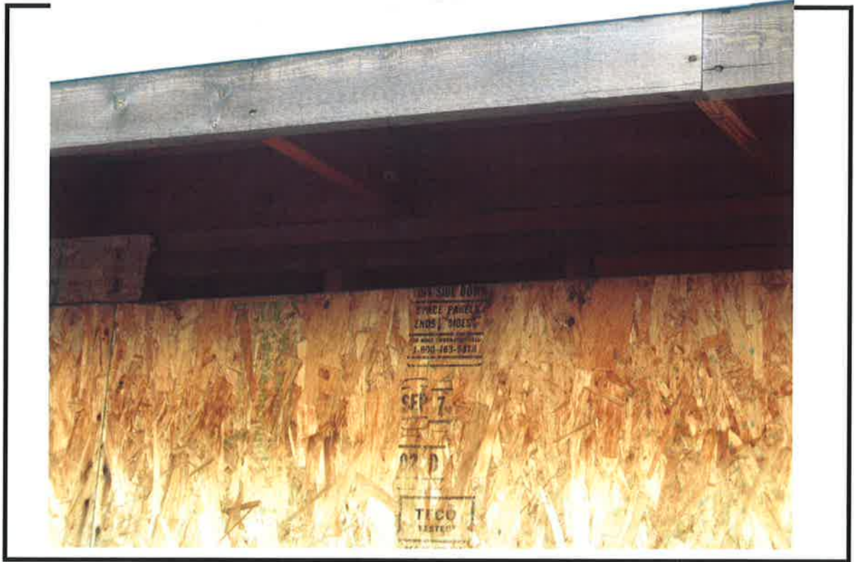
PHOTO # 13 DATE: 01/08/08 TAKEN BY: A Green#69 NOTES: EXPOSED WALLS N.O.D. # 7
