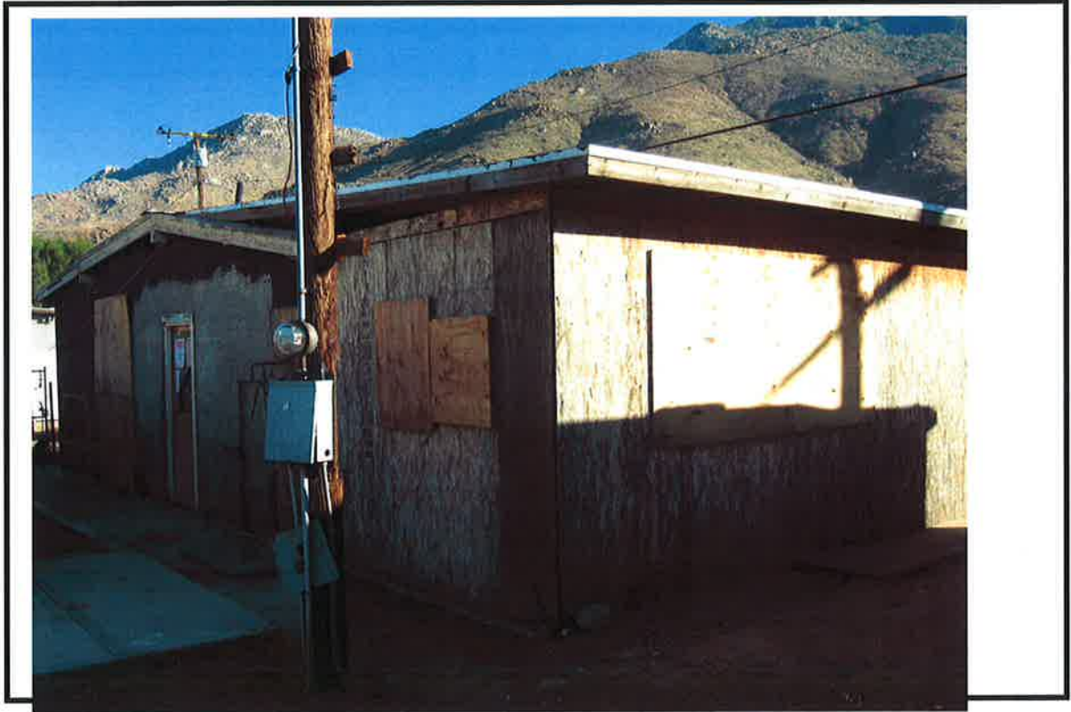
PHOTO # 3 DATE: 01/08/08 TAKEN BY: A Green#69 NOTES: EXPOSED WALLS N.O.D.# 13
