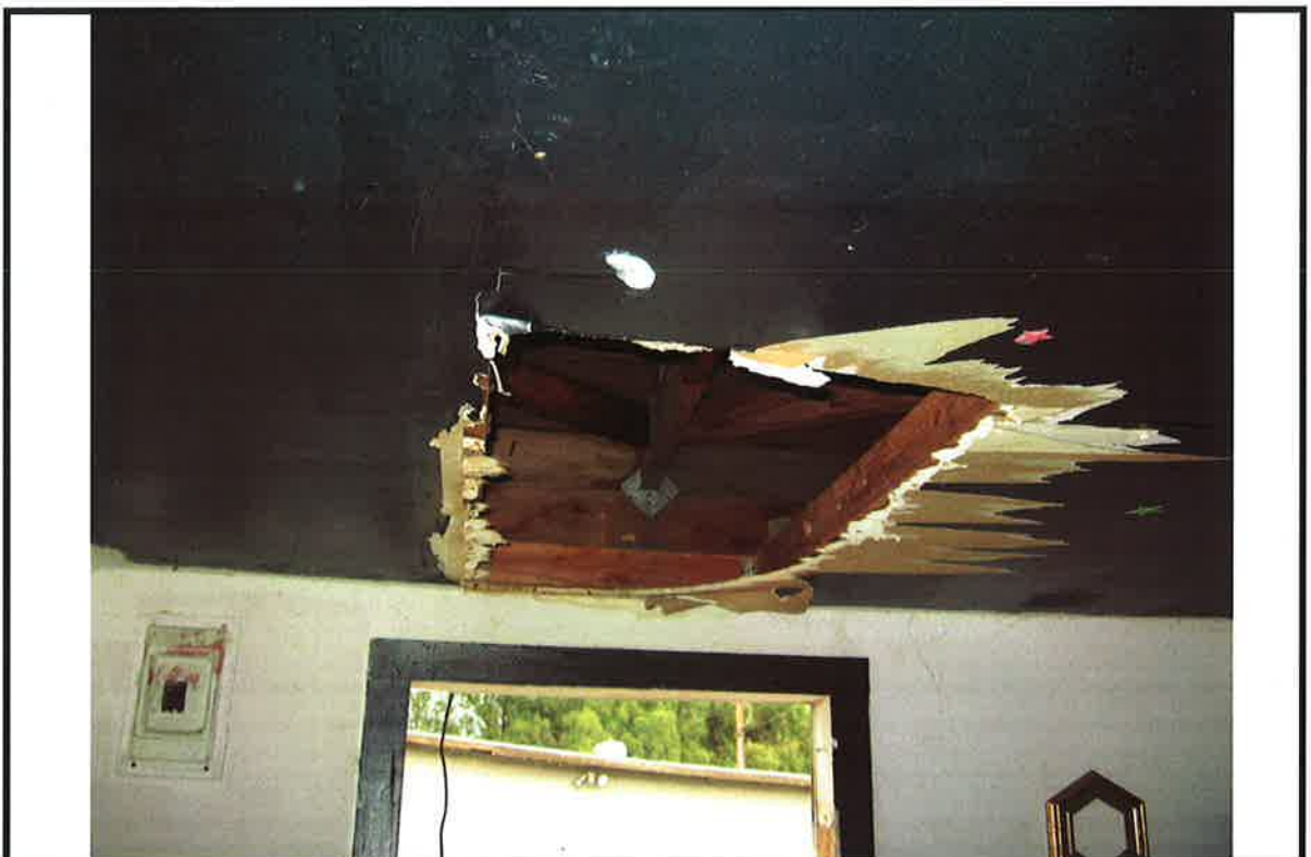
PHOTO # 8 DATE: TAKEN BY: # NOTES: Hole in ceiling CEILING BUCKLING N.O.D.# 11,
