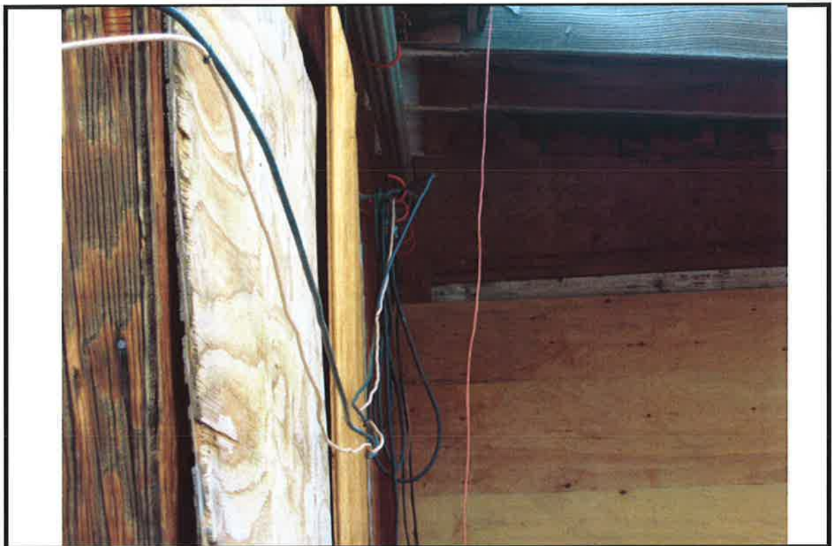
PHOTO # 4 DATE: TAKEN BY: # NOTES: ELECTRICAL WIRES HANGING FROM CEILING N.O.D. # 6
