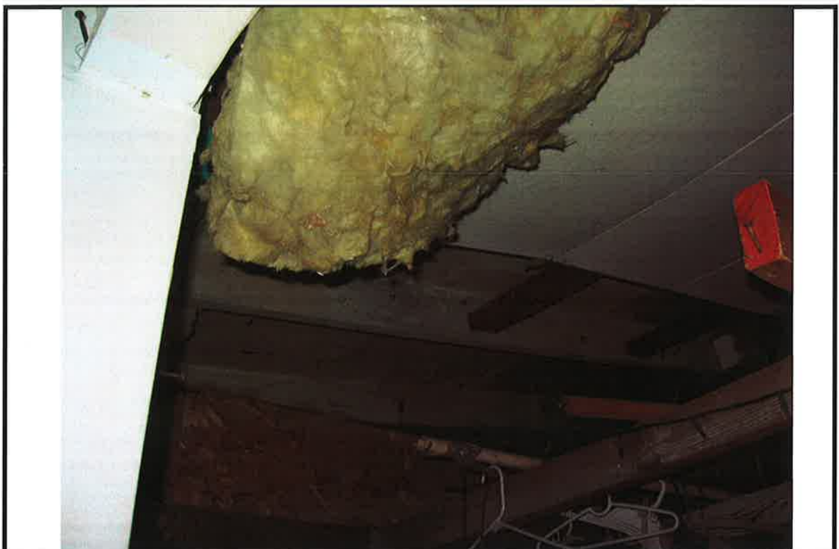
PHOTO # 10 DATE: TAKEN BY: # NOTES: INSULATION EXPOSED N.O.D. # 13
