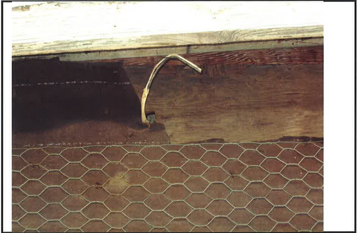
PHOTO # 5 DATE: 01/08/08 TAKEN BY: A Green#69 NOTES: chicken wire and exposed electrical wire. N.o.d. #6, 7
