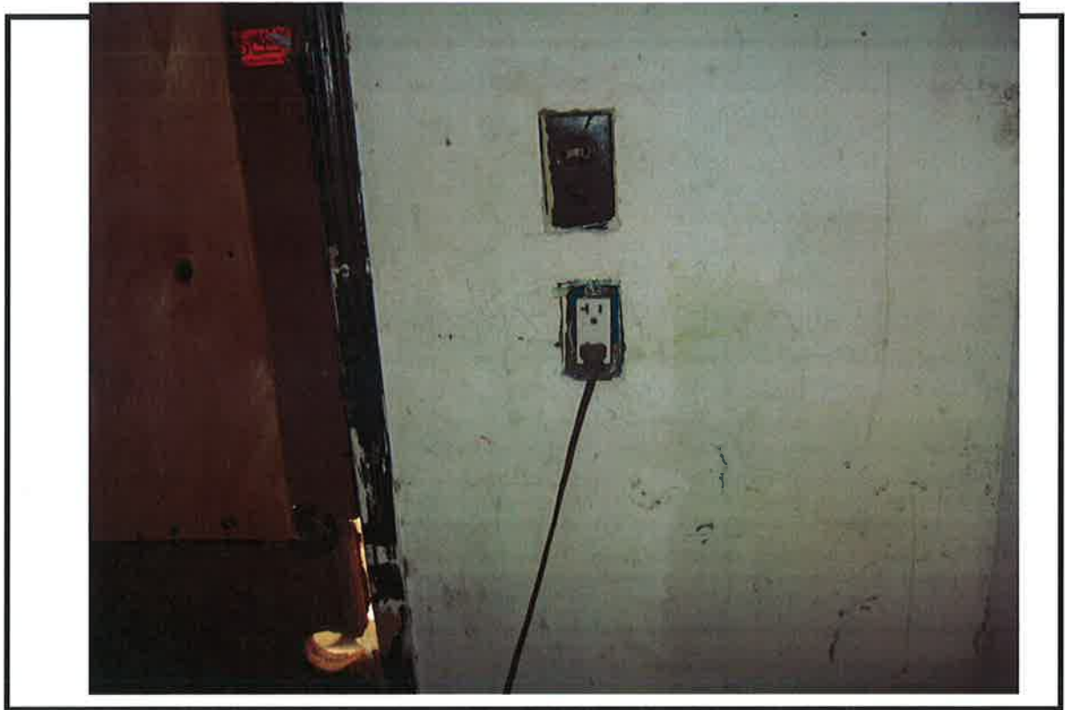
PHOTO # 11 DATE: 01/08/08 TAKEN BY: A Green#69 NOTES: EXPOSED Wires and socket area. N.O.D. #6
