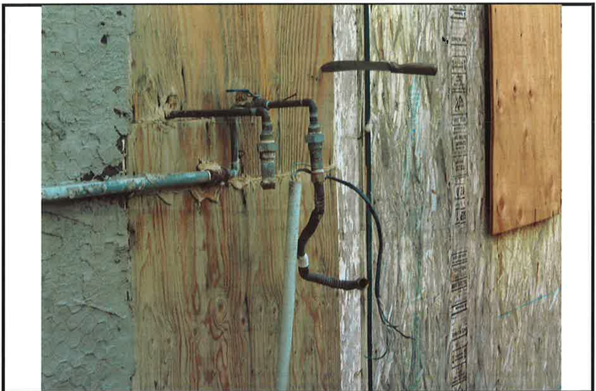
PHOTO # 6 DATE: TAKEN BY: # NOTES: Faulty electrical wires and plumbing N.O.D. 3 , 6
