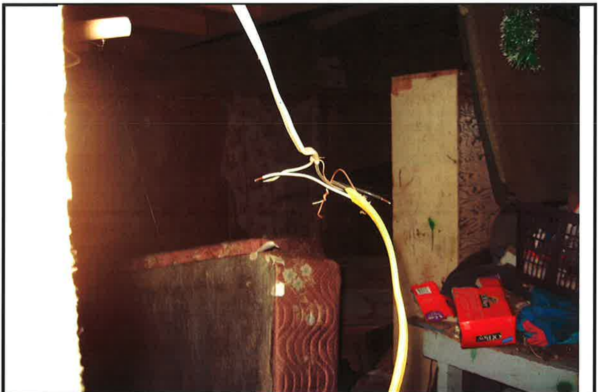
PHOTO # 12 DATE: TAKEN BY: # NOTES: exposed wires N.O.D. #6
