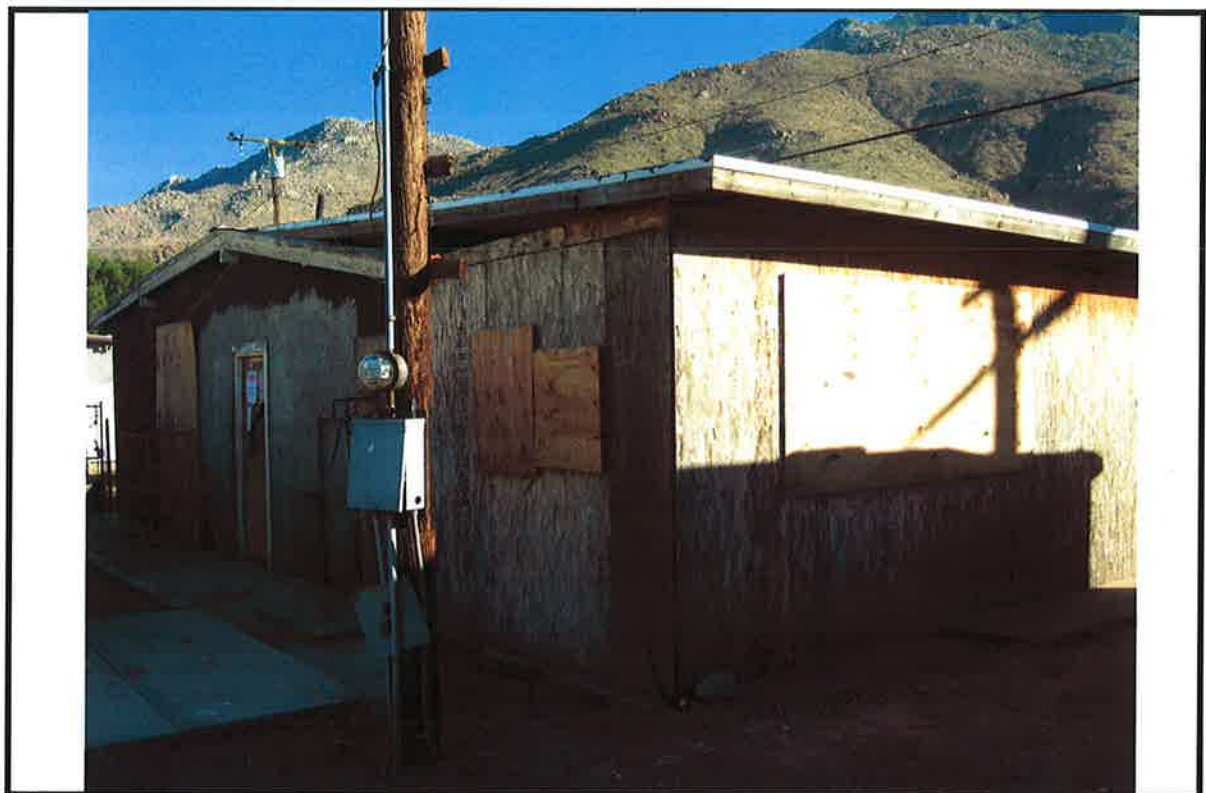
PHOTO # 14 DATE: TAKEN BY: # NOTES: No stucco all plywood for outside walls. N.O.D. #13
