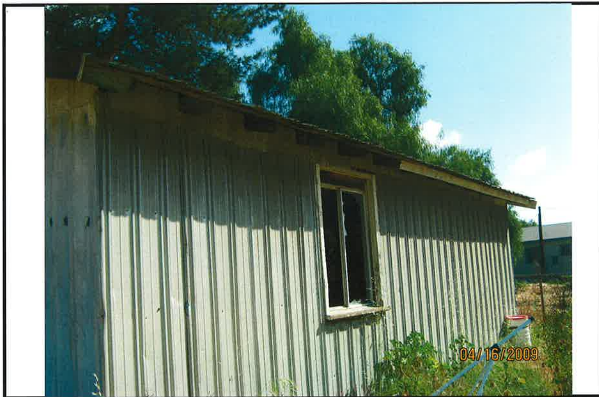
PHOTO #3 Notes: Building is vacant and abandoned.
