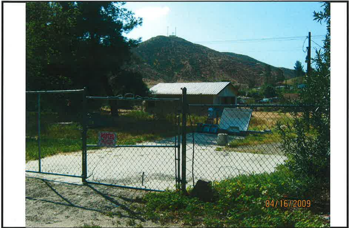
PHOTO# 1 Notes: Substandard Garage
