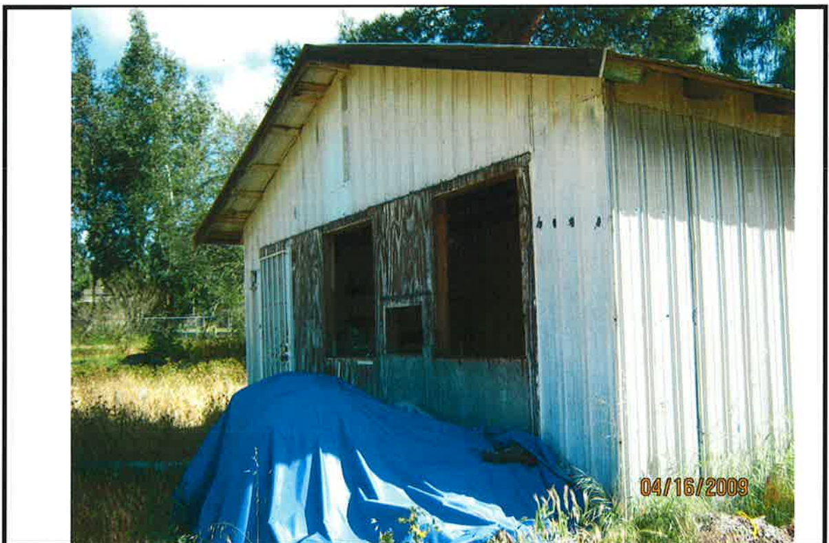
PHOTO #2 Notes: Defect # 10, 11, 12, 13 – Exterior walls deteriorated, roof not secure onto building, broken/missing window allowing elements to enter.
