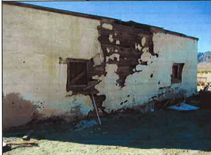
Structure # 1 - Garage Defect # 10, 11, 13, 14 & 17
