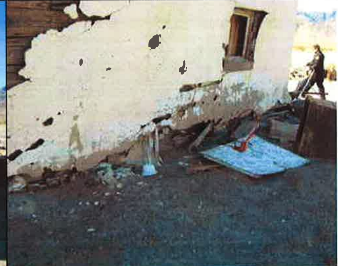
Structure # 1 - Garage Defect # 10, 11, 13, 14 &
