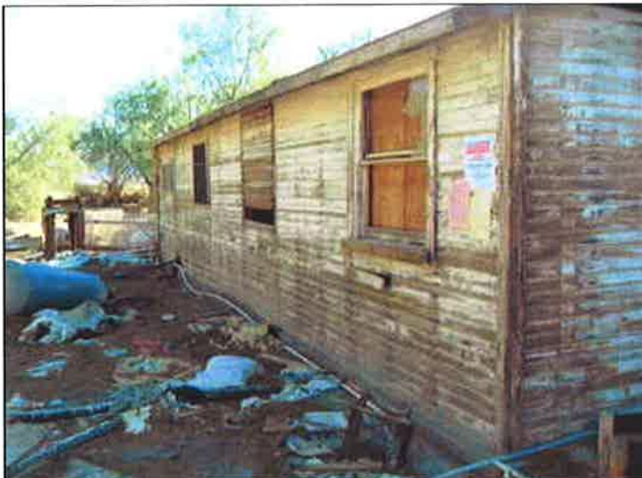
Structure # 3 - House Defect # 11, 13, 14 & 17
