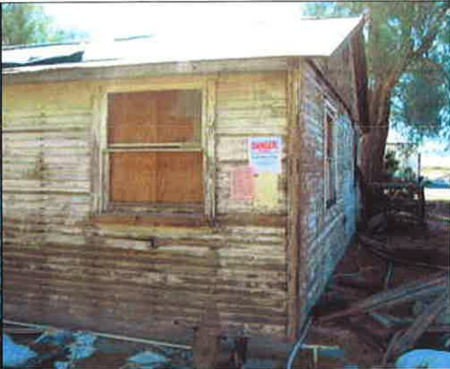
Structure # 3 - House Defect # 11, 13, 14 & 17
