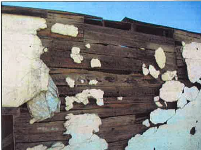
Structure # 1 - Garage Defect # 10, 11, 13, 14 & 17
