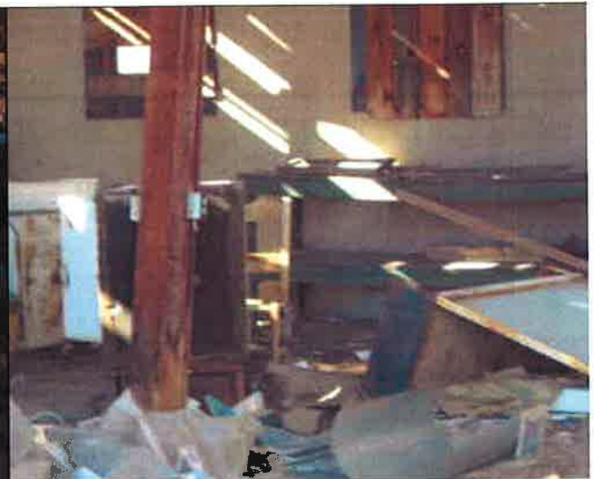
Accumulated Rubbish in Structure
