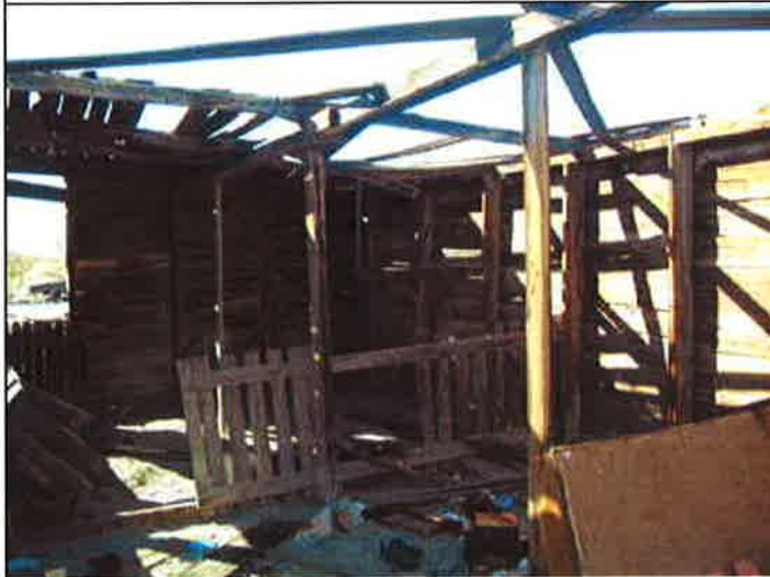
Structure # 2 - Ag. Building Defect # 10, 11, 13, 14 & 17
