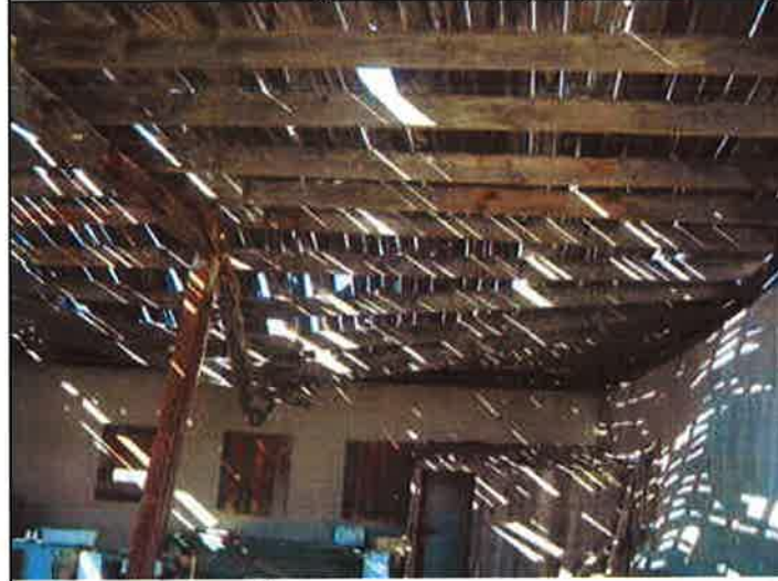
Structure # 1 - Garage Defect # 10, 11, 13, 14 & 17
