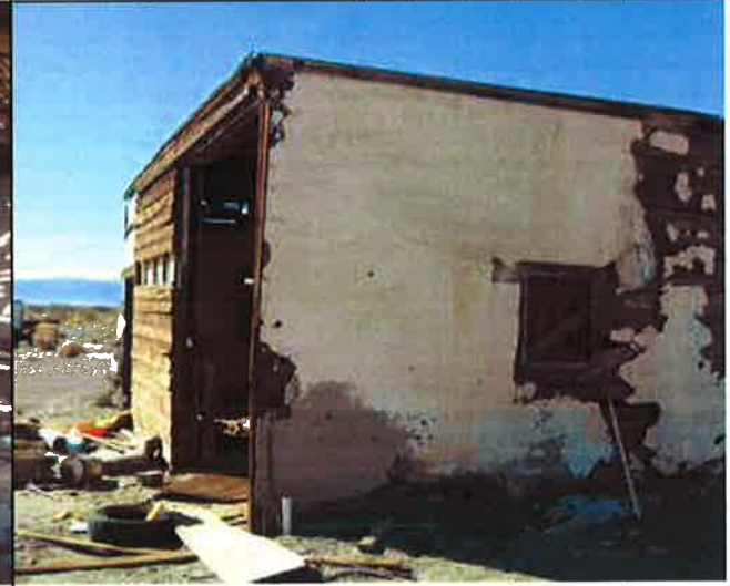
Structure # 1 - Garage Defect # 10, 11, 13, 14 &
