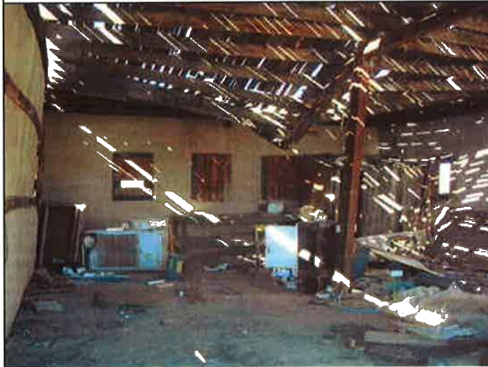
Structure # 1 - Garage Defect # 10, 11, 13, 14 & 17
