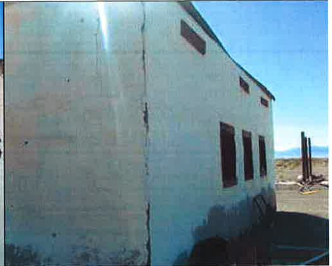
Structure # 1 - Garage Defect # 10, 11, 13, 14 &
