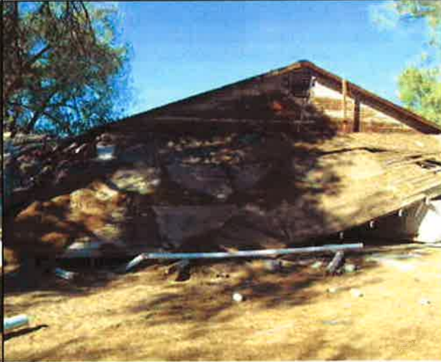
Structure # 3 - House Defect # 11, 13, 14 & 17
