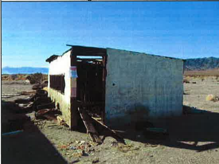
Structure # 2 - Ag. Building Defect # 10, 11, 13, 14 & 17
