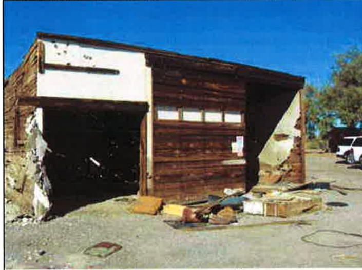
Structure # 1 - Garage Defect # 10, 11, 13, 14 & 17
