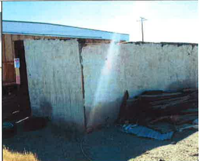
Structure # 2 - Ag. Building Defect # 10, 11, 13, 14 & 17
