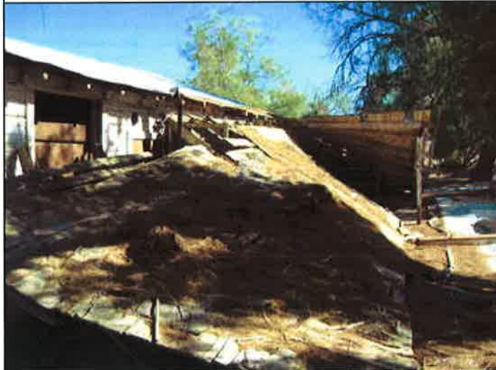
Structure # 3 - House Defect # 11, 13, 14 & 17
