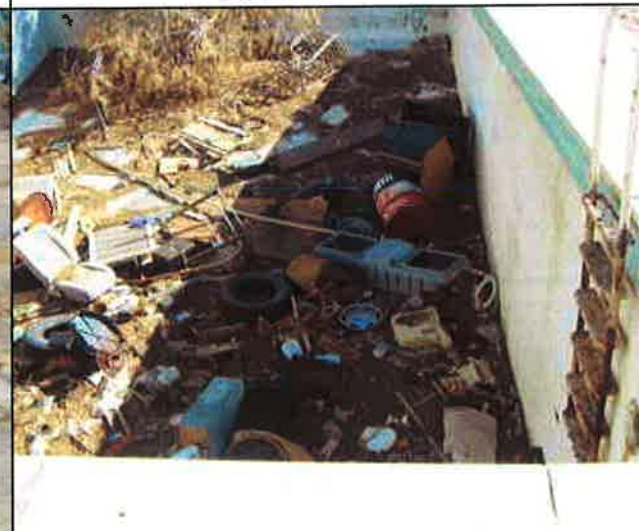
Accumulated Rubbish in Pool
