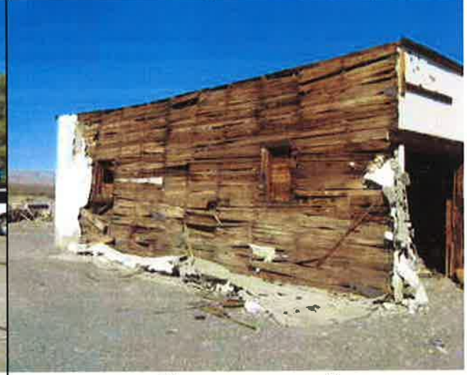
Structure # 1 - Garage Defect # 10, 11, 13, 14 &
