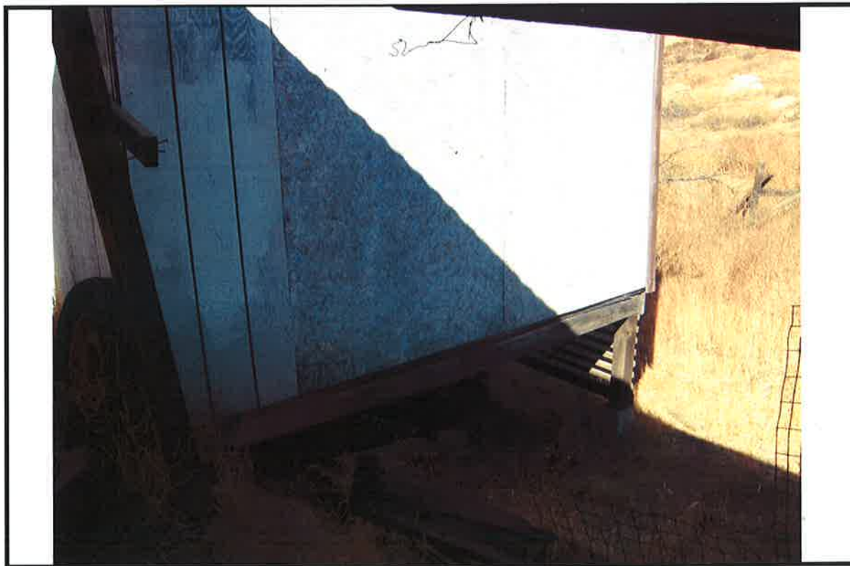
PHOTO # 15 DATE: 10/15/2008 TAKEN BY: LPADILLA 26580 PEACH ST, DEFECTS 8,9
