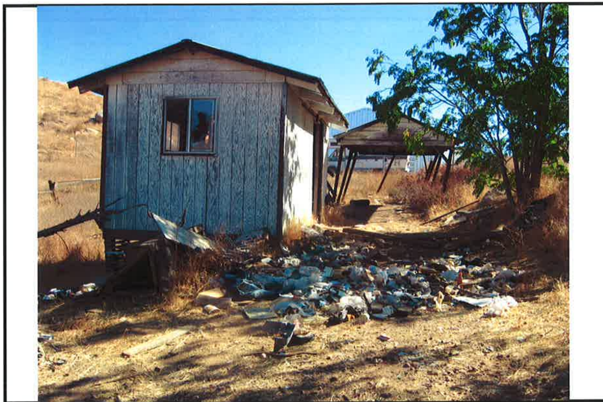
PHOTO # 19 DATE: 10/15/2008 TAKEN BY: LPADILLA 26580 PEACH ST, SUBSTANDARD STRUCTURE #4 CARPORT
