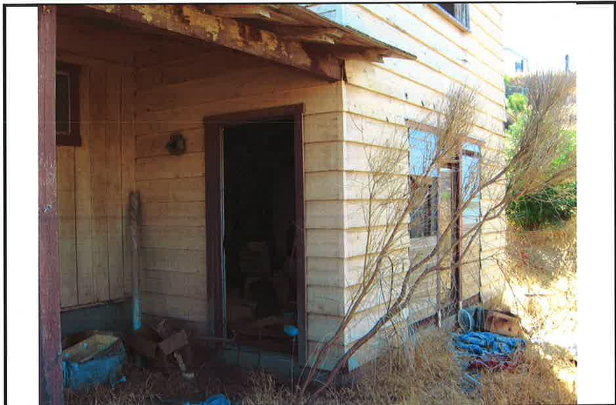
PHOTO # 10 DATE: 10/15/2008 TAKEN BY: LPADILLA 26580 PEACH ST, DEFECTS 8 DETERIORATED OR INADEQUATE FOUNDATION. END OF STRUCTURE 1 PHOTOS OF DEFECTS.
