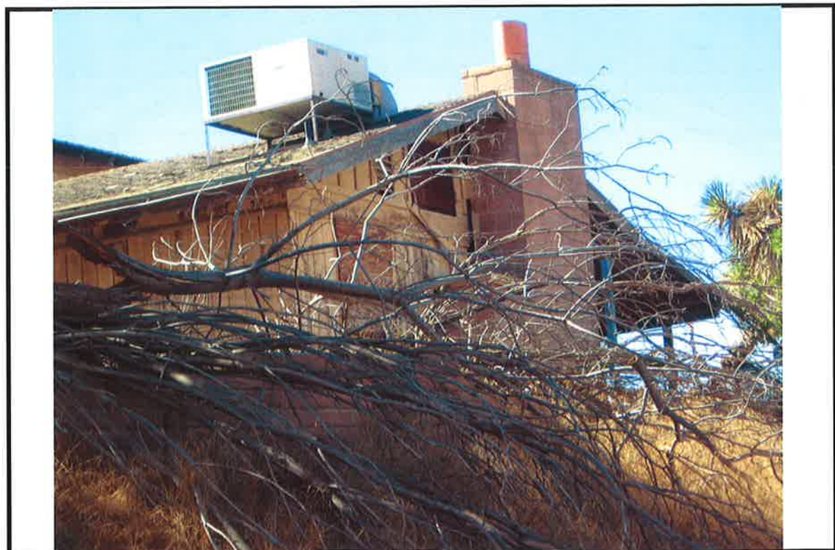
PHOTO # 2 DATE: 10/15/2008 TAKEN BY: LPADILLA 26580 PEACH ST, SUBSTANDARD STRUCTURE 1 MAIN DWELLING
