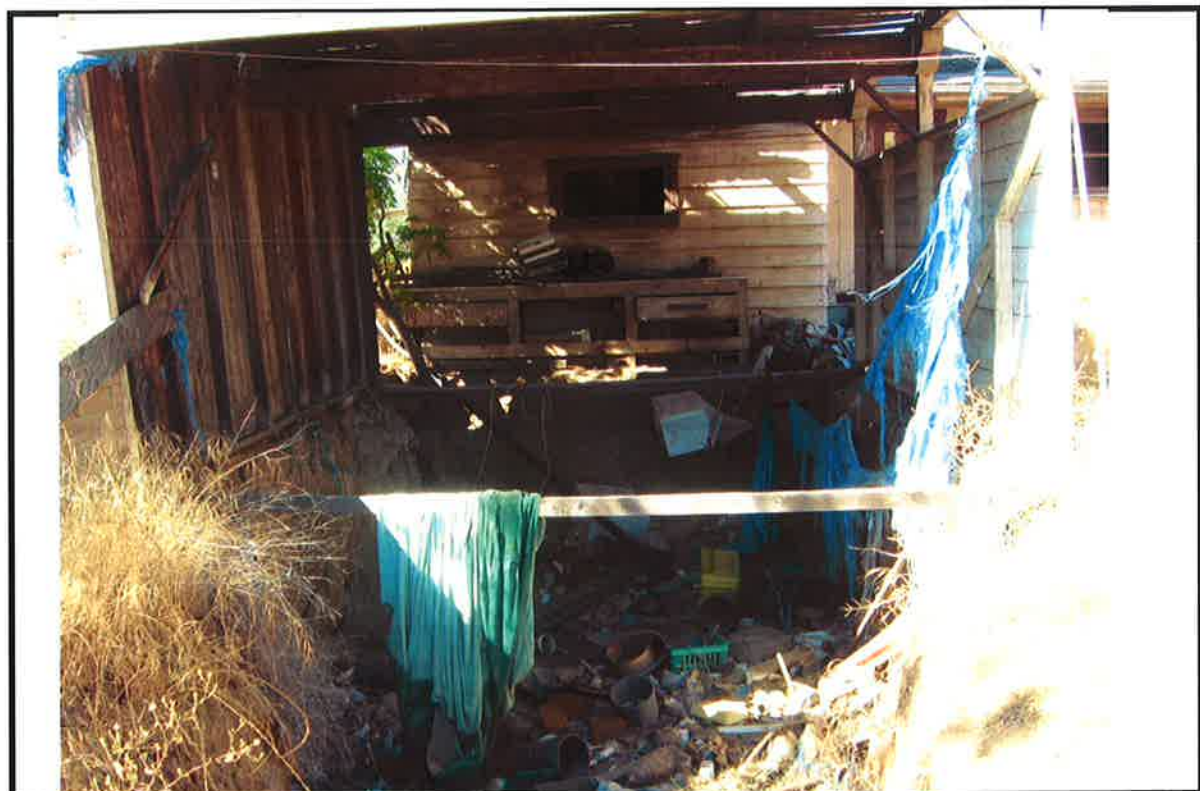
PHOTO # 12 DATE: 10/15/2008 TAKEN BY: LPADILLA 26580 PEACH ST, DEFECTS 9,11,14,17.
