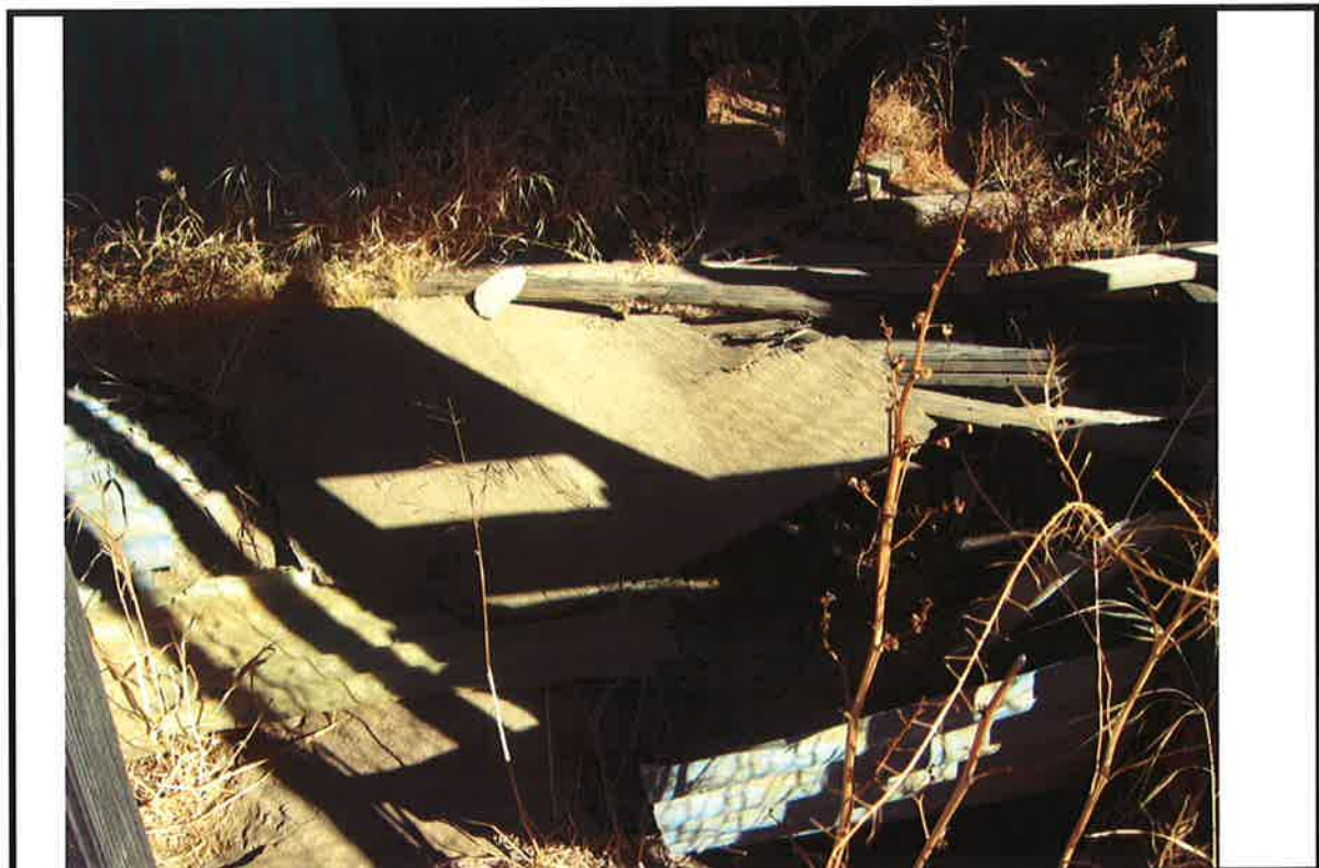
PHOTO # 22 DATE: 10/15/2008 TAKEN BY: LPADILLA 26580 PEACH ST, DEFECTS 8,9.
