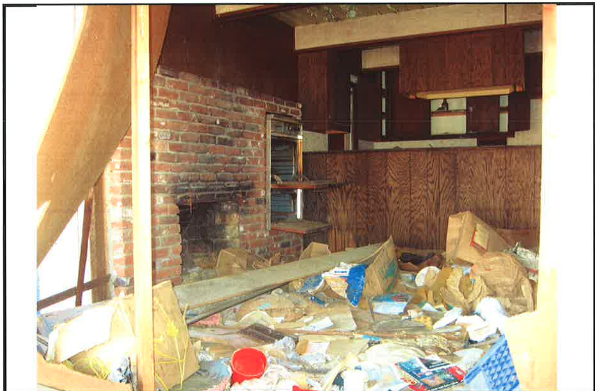
PHOTO # 8 DATE: 10/15/2008 TAKEN BY: LPADILLA 26580 PEACH ST, DEFECT 7 INADEQUATE HEATING FACILITIES, HEATER REMOVED.
