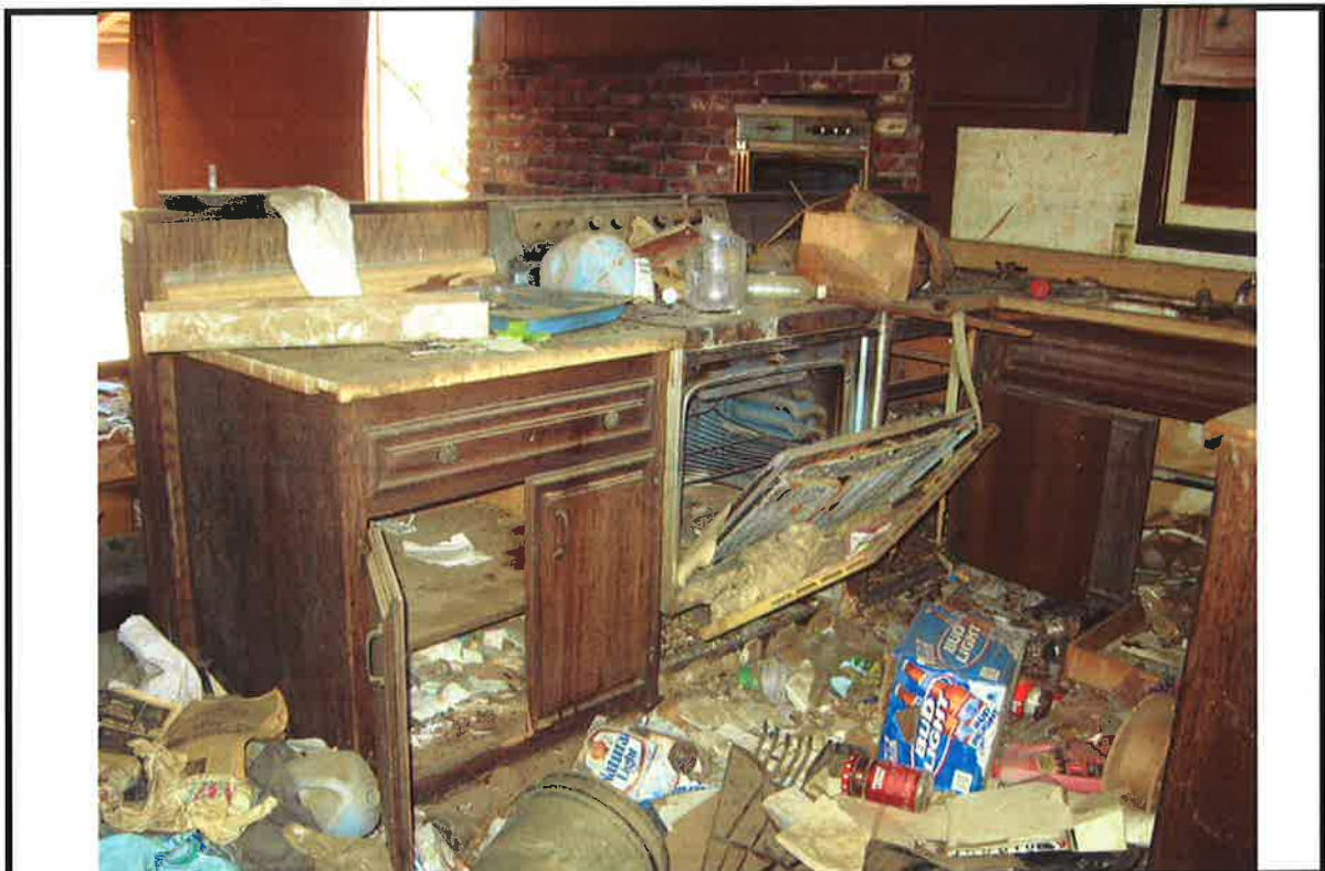
PHOTO # 6 DATE: 10/15/2008 TAKEN BY: LPADILLA 26580 PEACH ST, KITCHEN FILLED WITH RUBBISH
