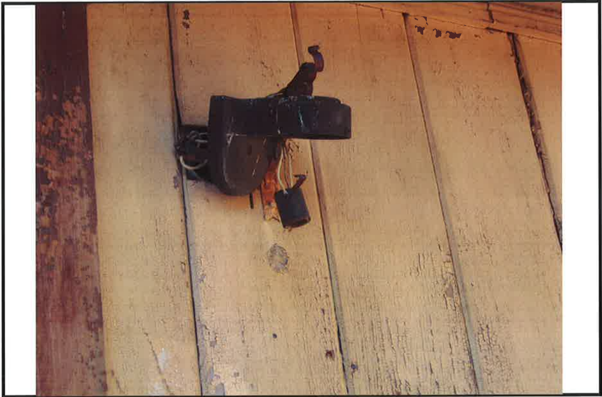
PHOTO # 5 DATE: 10/15/2008 TAKEN BY: LPADILLA 26580 PEACH ST, DEFECTS 5,6. HAZARDOUS ELECTRIC AND LACK OF ELECTRICITY.
