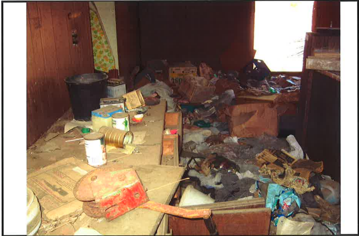
PHOTO # 7 DATE: 10/15/2008 TAKEN BY: LPADILLA 26580 PEACH ST, PERRIS SUBSTANDARD STRUCTURES X5
