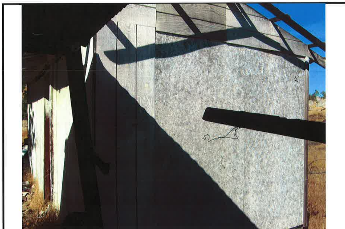
PHOTO # 16 DATE: 10/15/2008 TAKEN BY: LPADILLA 26580 PEACH ST, DEFECTS 14,15
