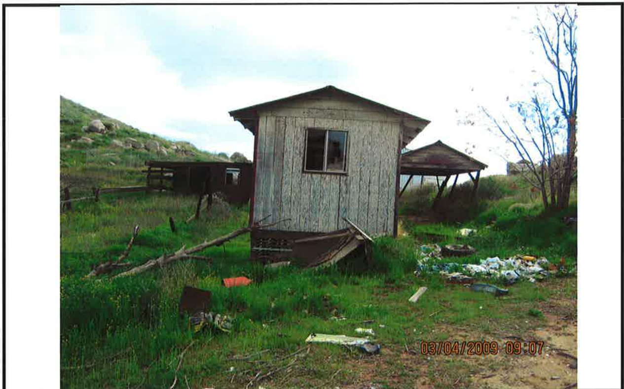
PHOTO # 3 TAKEN BY: J DIETRICH NOTES : Sub-Standard Structures # 3,4 & 5
