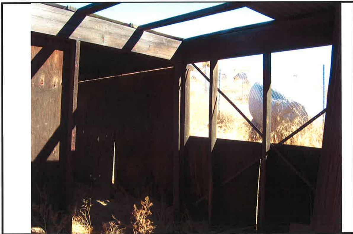
PHOTO # 23 DATE: 10/15/2008 TAKEN BY: LPADILLA 26580 PEACH ST, DEFECTS 10,11,15,17.
