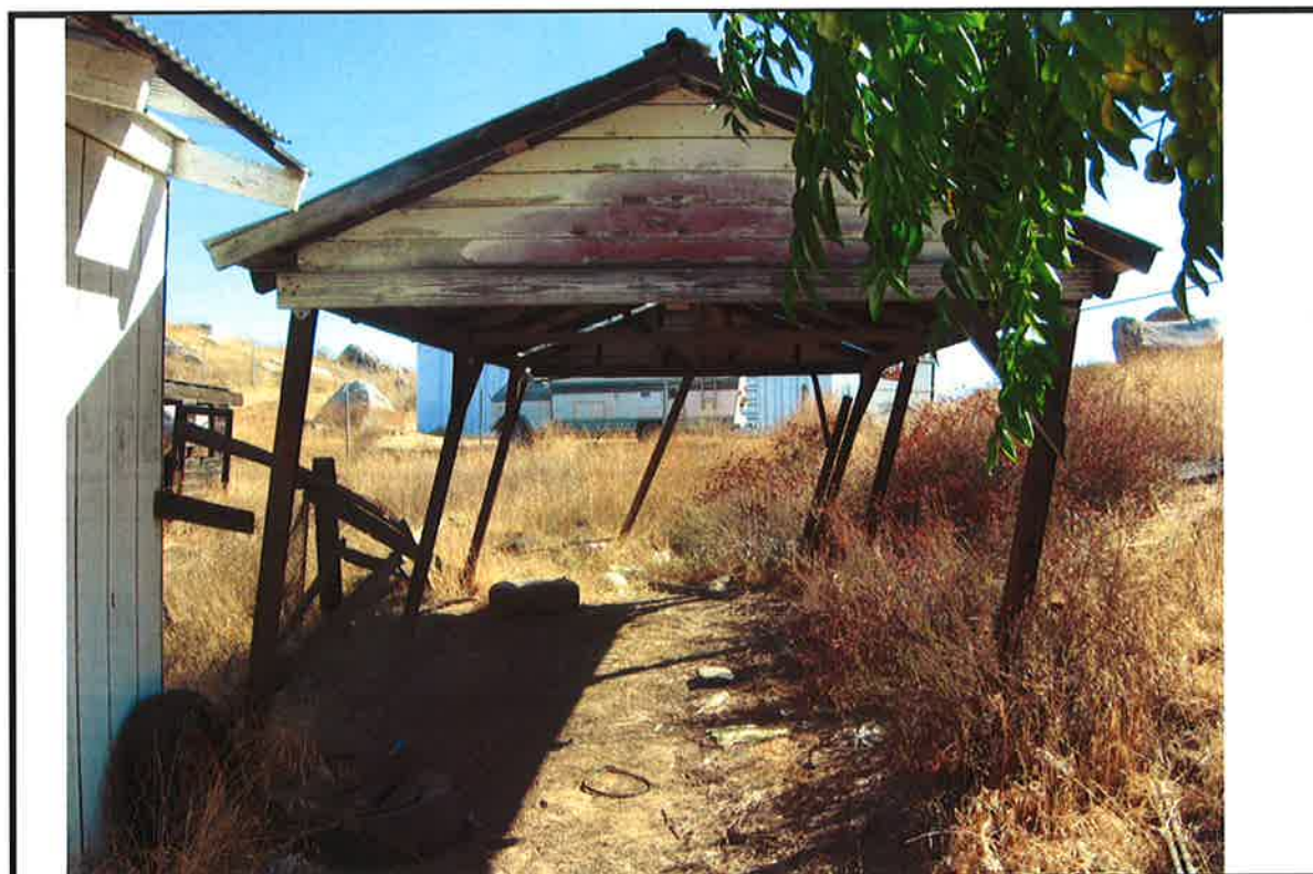
PHOTO # 20 DATE: 10/15/2008 TAKEN BY: LPADILLA 26580 PEACH ST, DEFECTS 11,14,17. END OF SSS #4 PHOTOS
