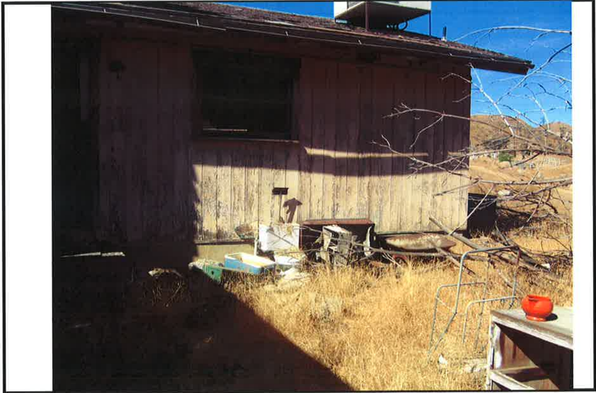
PHOTO # 3 DATE: 10/15/2008 TAKEN BY: LPADILLA 26580 PEACH ST, DEFECTS 12,13,14
