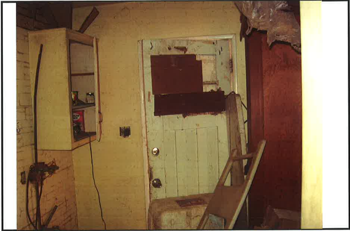
PHOTO # 9 DATE: 10/15/2008 TAKEN BY: LPADILLA 26580 PEACH ST, DEFECTS LACK OF HOT AND COLD RUNNING WATER
