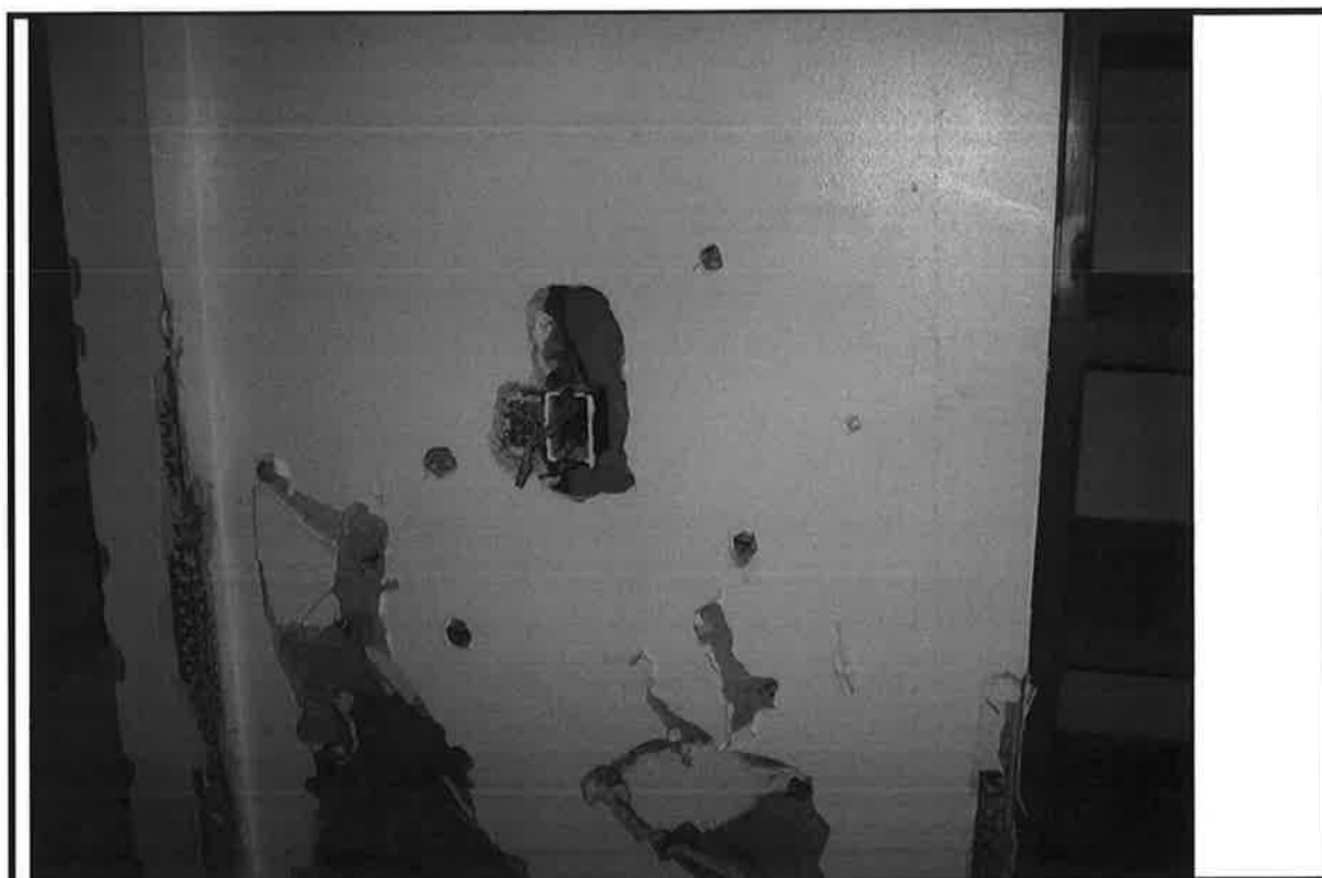
PHOTO # 6 DATE: 04/27/09 TAKEN BY: a. green #69 NOTES: #6, 14 WALLS HAVE HOLES.
