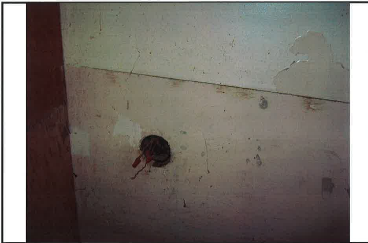
PHOTO # 11 DATE: 04/27/09 TAKEN BY: A Green#69 NOTES CEILING LIGHTING MISSING. N.O.D.# 5
