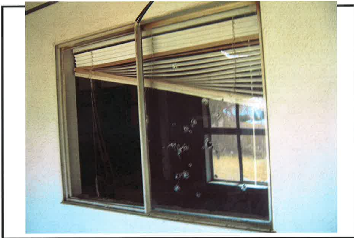
PHOTO # 3 DATE: 04/27/09 TAKEN BY: A Green#69 NOTES broken windows, bullet holes
