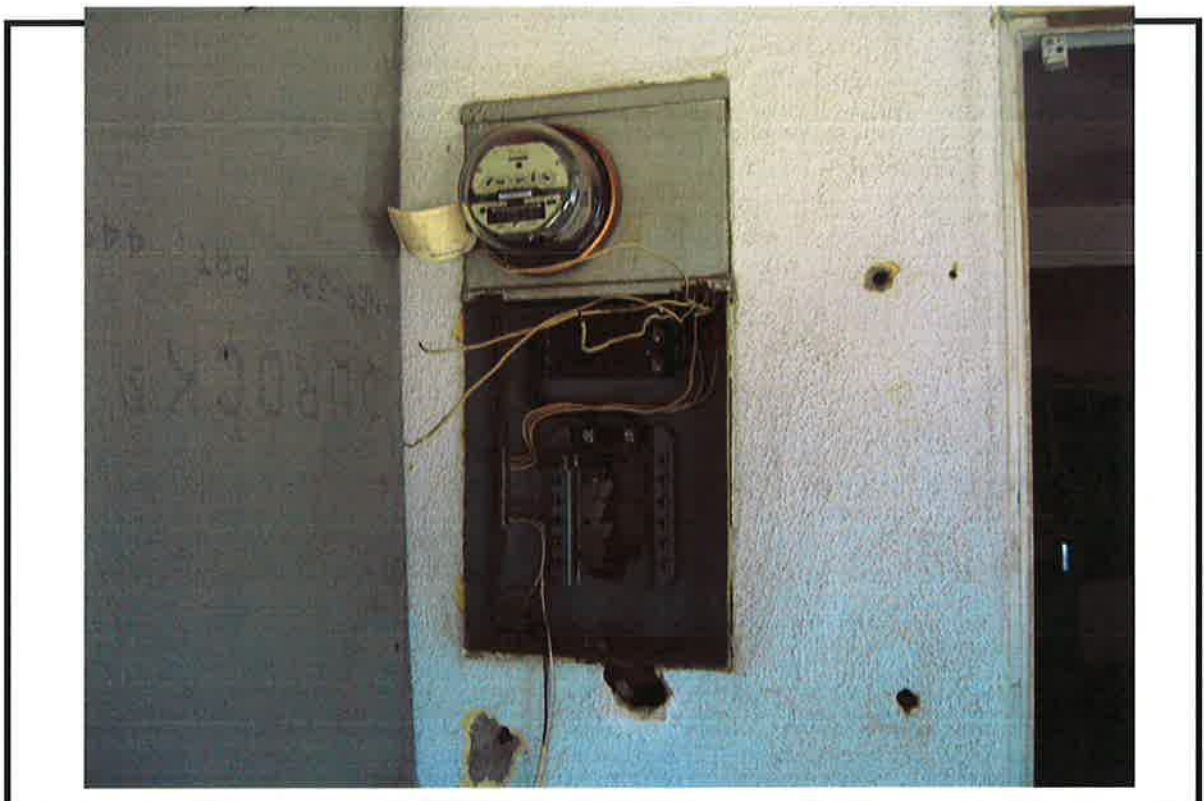
PHOTO # 10 DATE: 04/27/09 TAKEN BY: a. green #69 NOTES: N.O.D. # 6 POWER BOX
