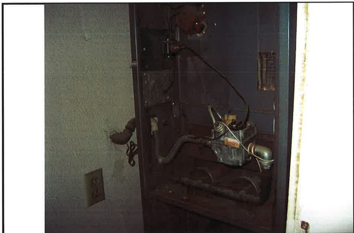
PHOTO # 8 DATE: 04/27/09 TAKEN BY: a. green #69 NOTES: HEATER MISSING PARTS N.O.D. # 7
