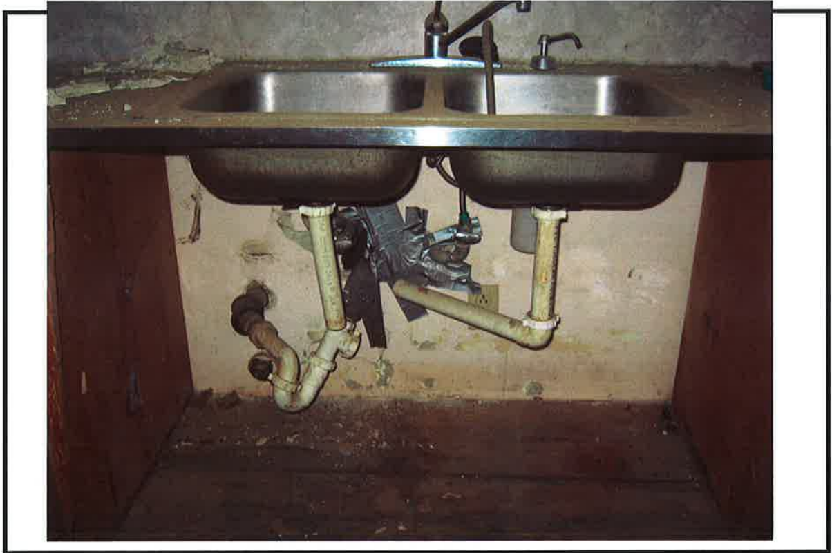
PHOTO # 9 DATE: 04/27/09 TAKEN BY: A Green#69 NOTES PLUMBING PIPES BROKEN N.O.D.# 4
