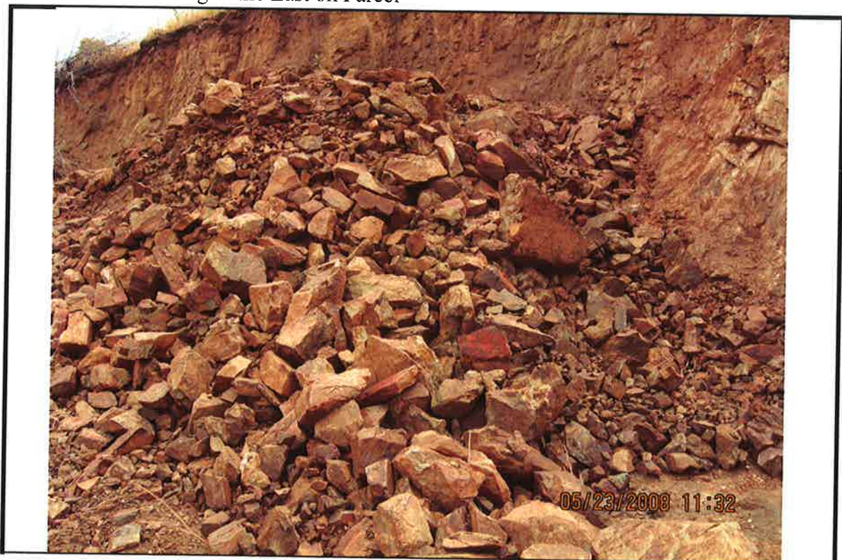
PHOTO # 12 TAKEN BY: D Jurden, CET ADDRESS: 20775 Gardenias Street NOTES: Photo of recent grading
