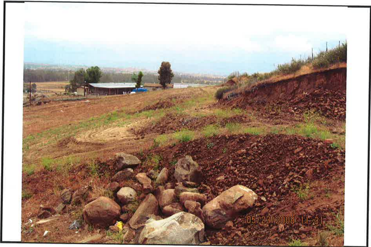
PHOTO # 11 TAKEN BY: D Jurden, CET ADDRESS: 20775 Gardenias Street NOTES: Looking to the East on Parcel
