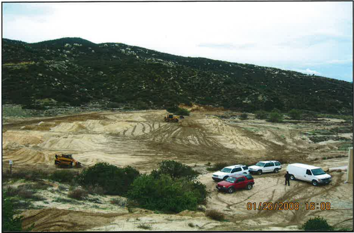
R Welch PHOTO # NOTES: Site in progress of being graded. Found by Officer S Stoll
