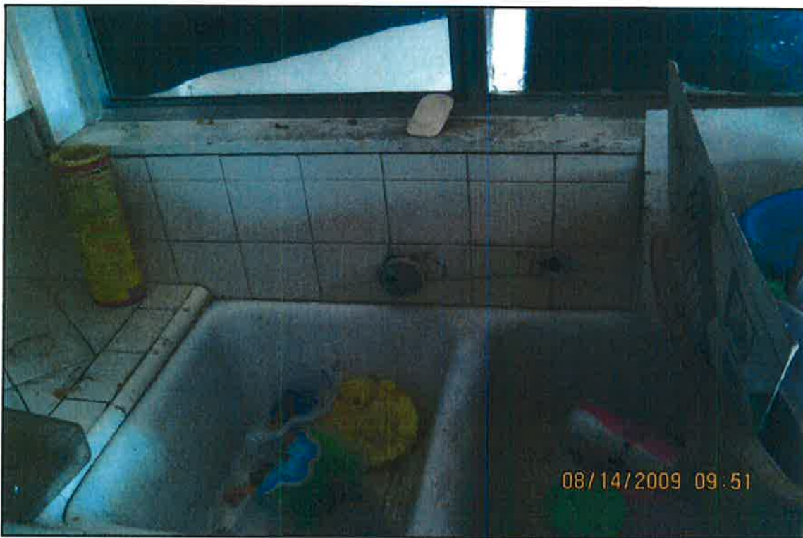
PHOTO # 1 NOTES: 2) Lack of hot and cold running water to plumbing fixture
