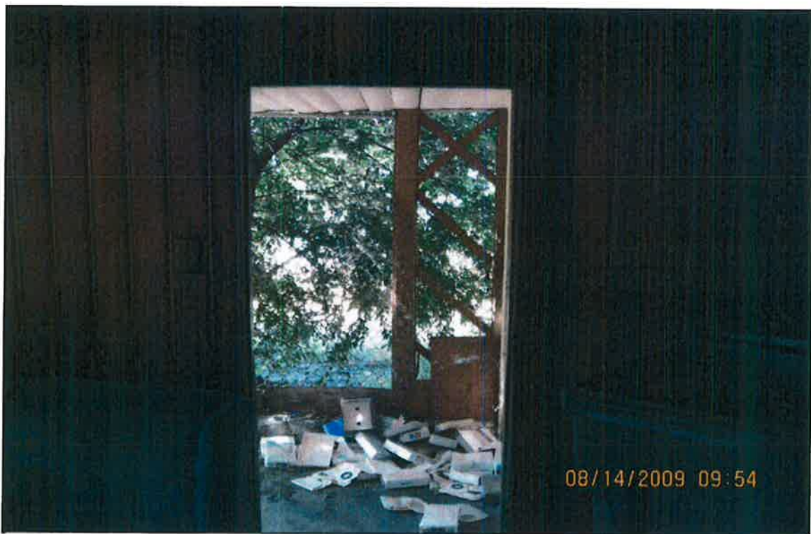
PHOTO # 2 NOTES: 13) Faulty weather protection
