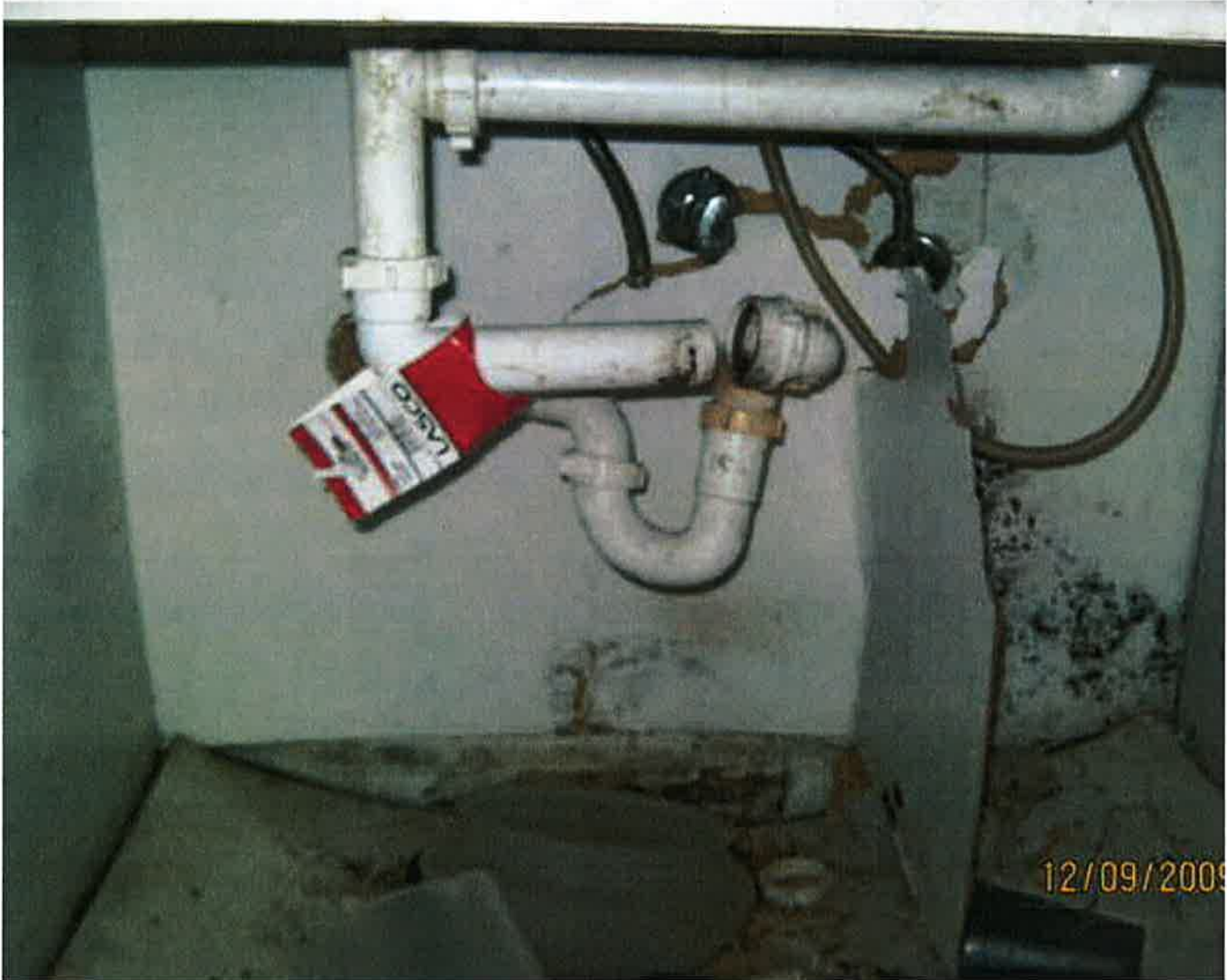
wdurant/photo of broken pipes under kitchen sink #4 - 12/09/2009
