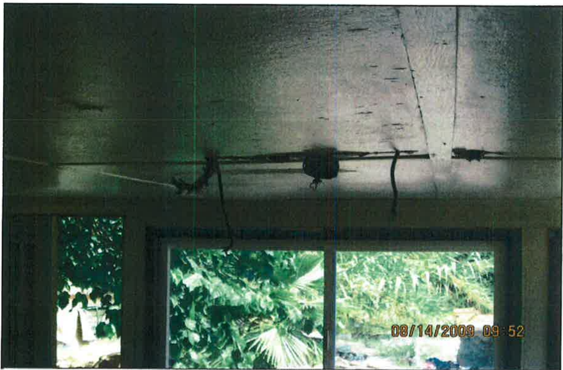
PHOTO # 2 NOTES: 6) Hazardous Wiring
