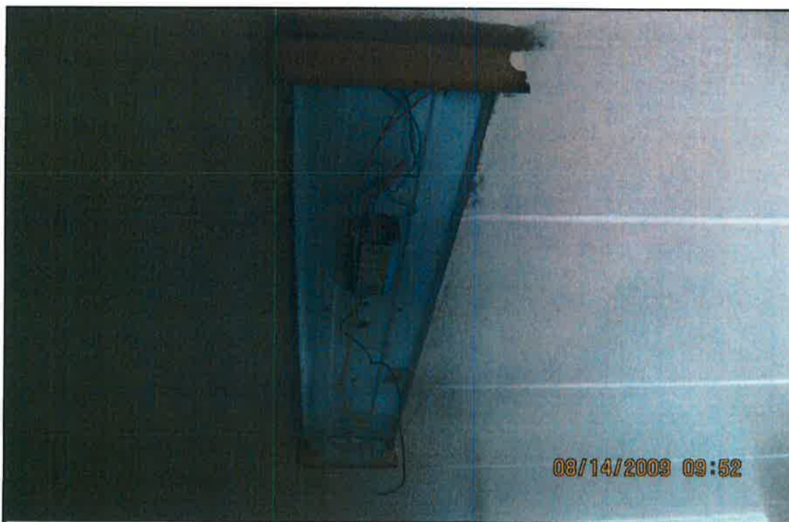
PHOTO # 2 NOTES: 5) Lack of required electrical lighting
