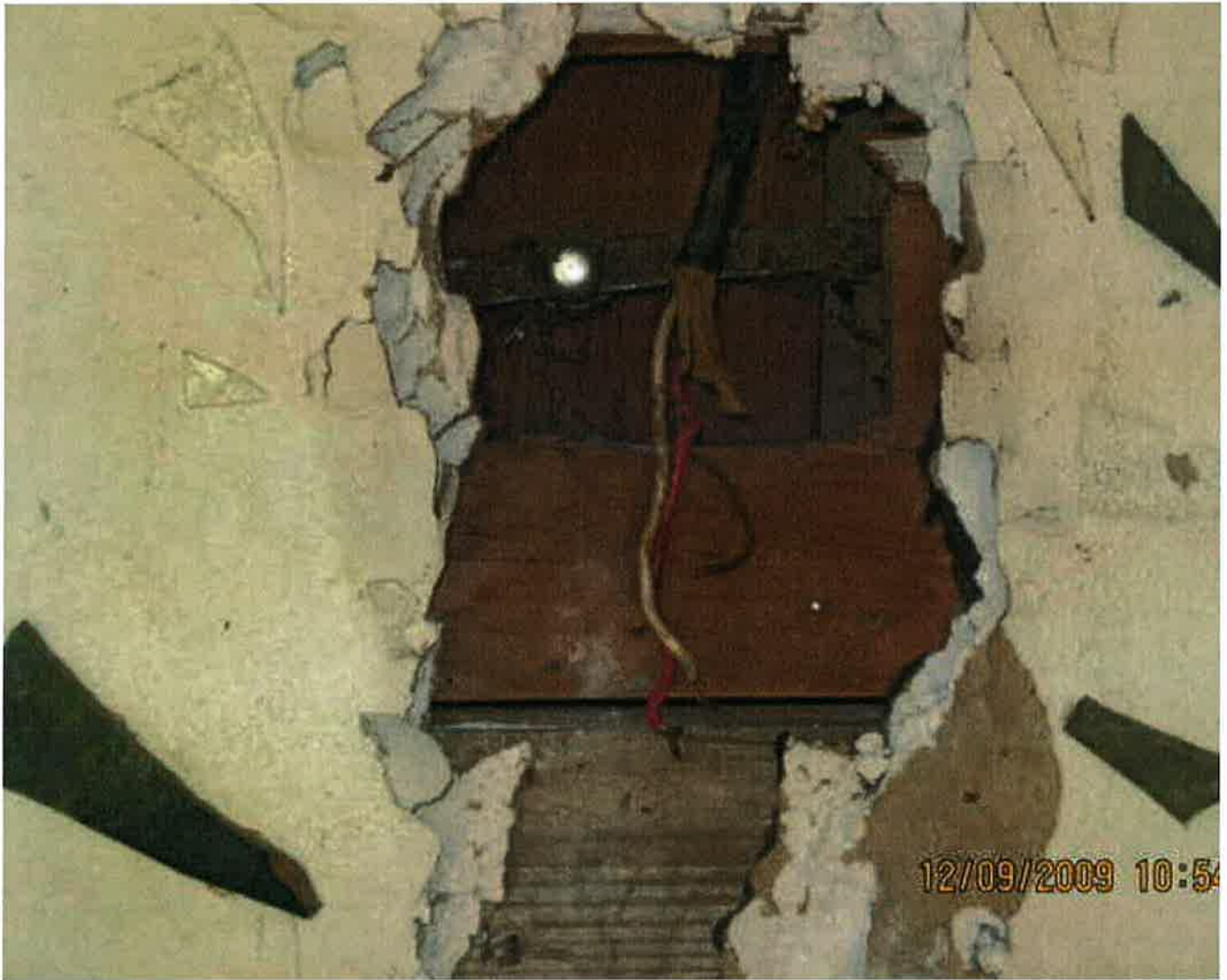
# 6 Hazardous wiring. CEO Frazier, A - 12/09/2009
