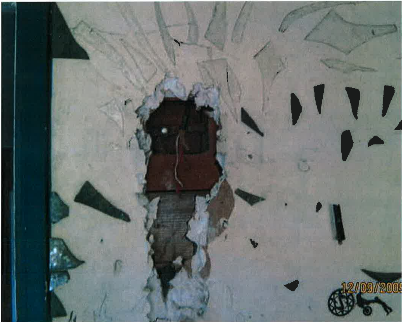
wdurant/photo of electrical wiring exposed #6 - 12/09/2009
