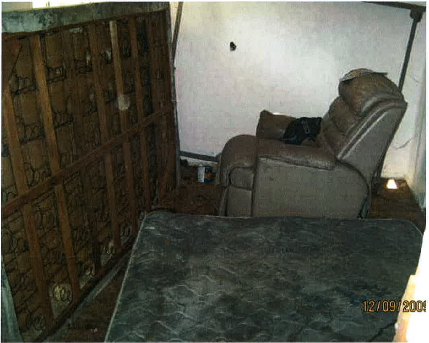
wdurant/photo of trash and debris in bedroom #14 - 12/09/2009
