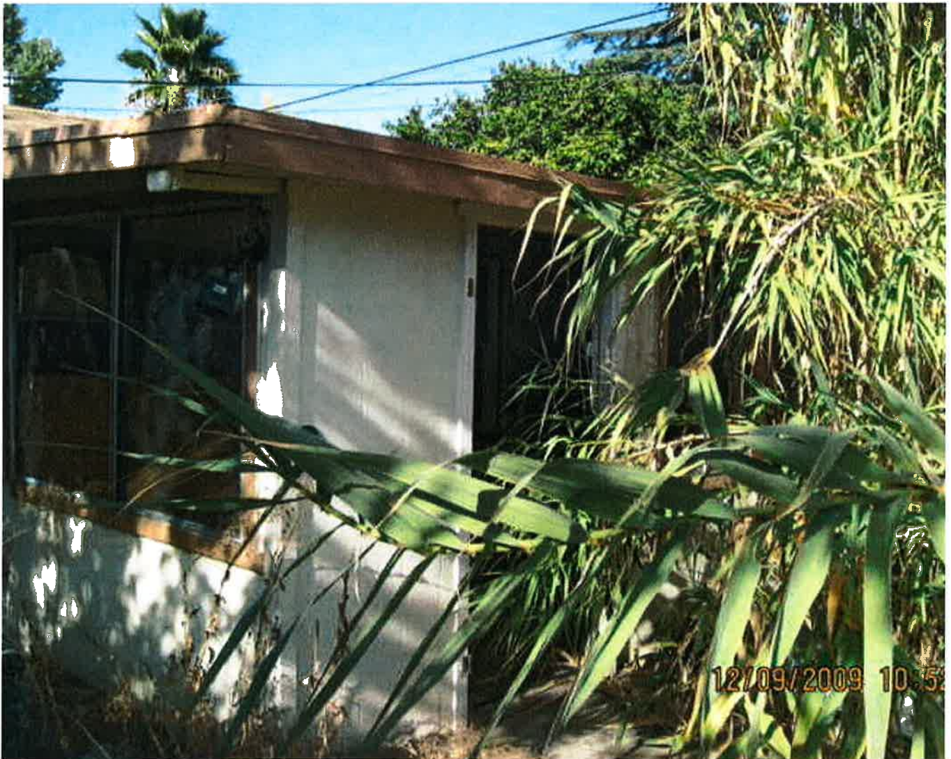
#12 Dampness of habitable rooms. No front door. CEO Frazier - 12/09/2009
