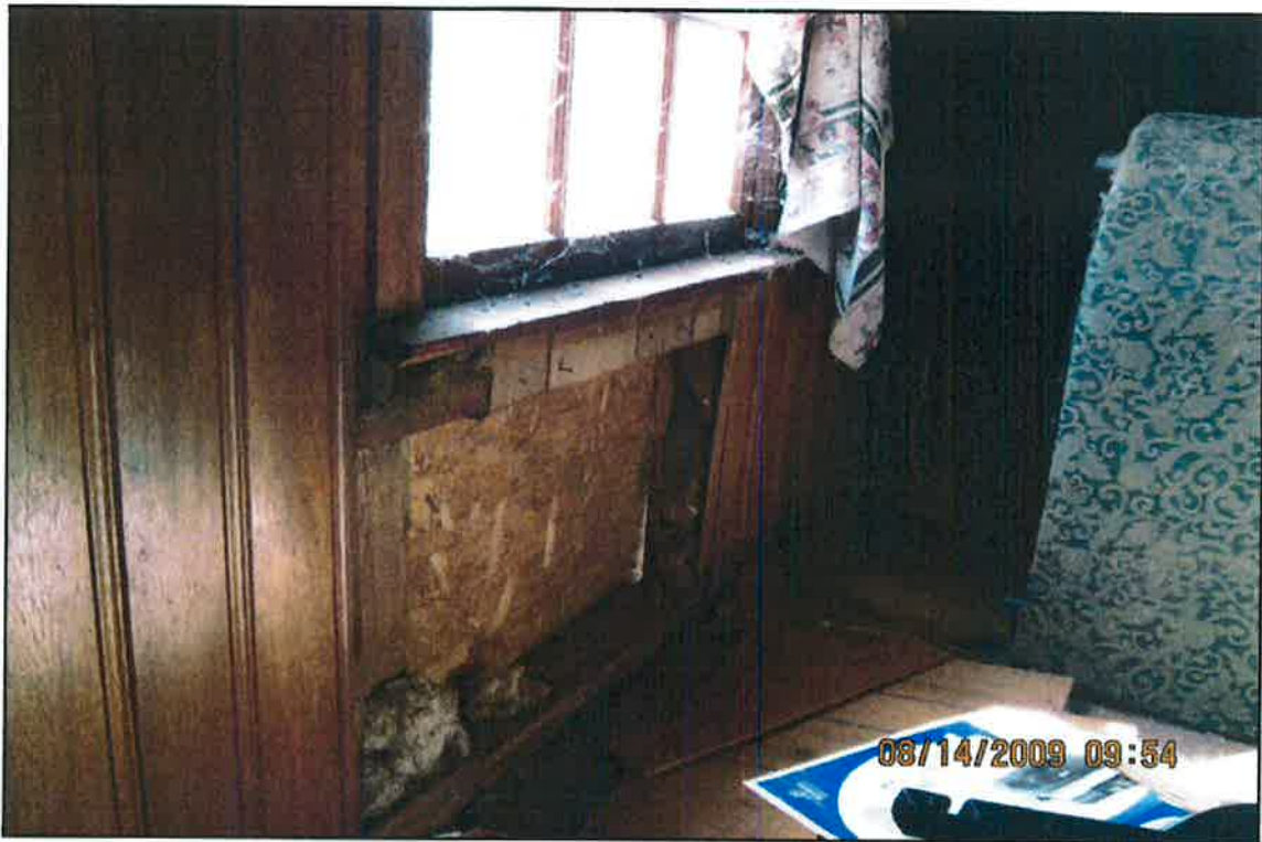
PHOTO # 1 NOTES: 13) Faulty weather protection
