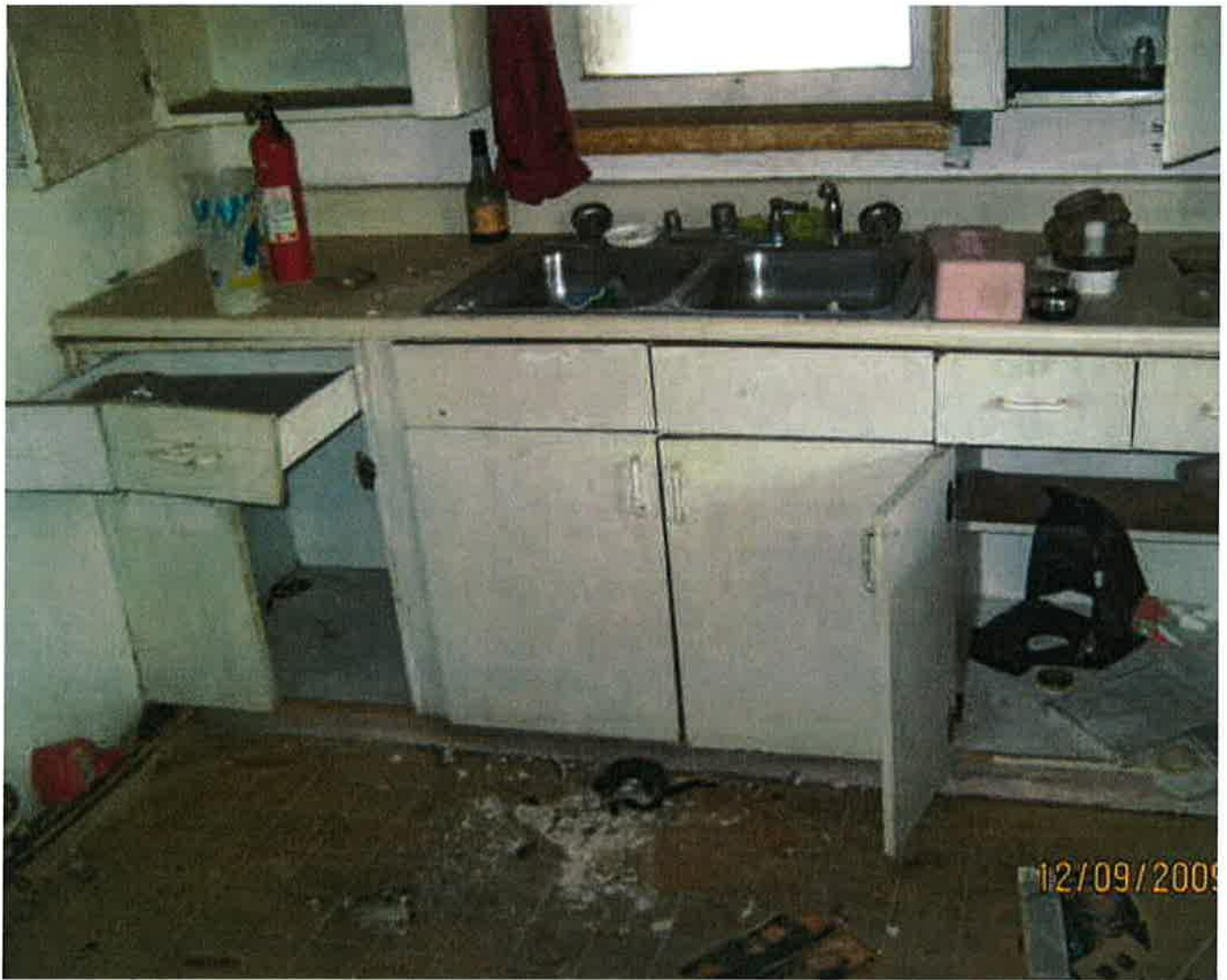
wdurant/photo of substandard kitchen area - 12/09/2009
