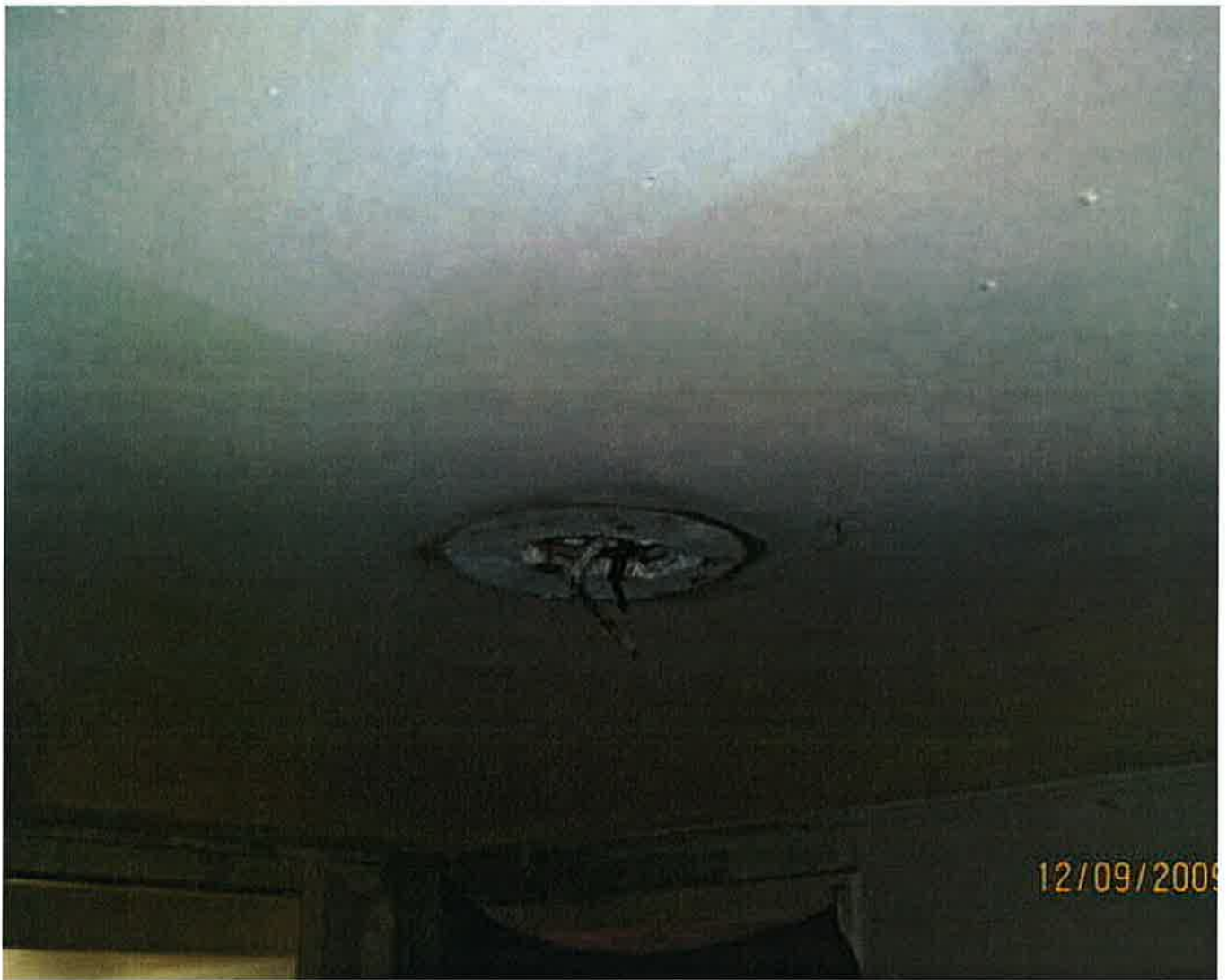
w Durant/photo of electrical wiring exposed #6 - 12/09/2009
