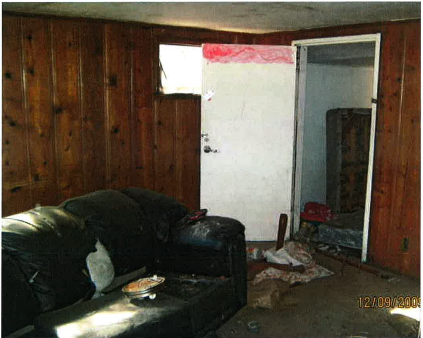
wdurant/photo of living room with trash and debris #16 - 12/09/2009
