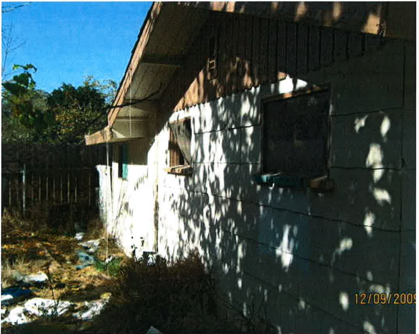
wdurant/exterior photo of substandard second unit - 12/09/2009
