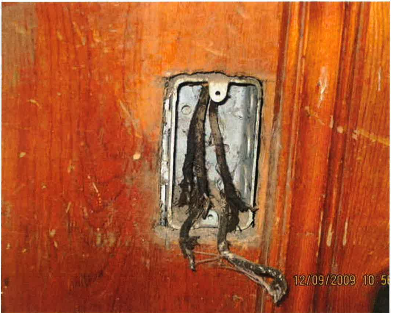
# 6 Hazardous wiring. CEO Frazier, A - 12/09/2009
