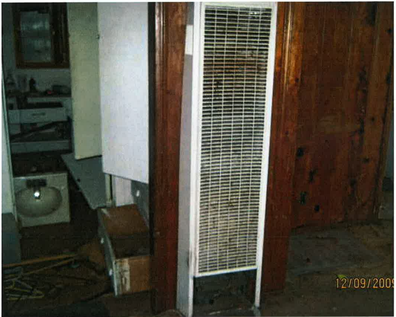
wdurant/photo of heater unit missing cover plate #7 - 12/09/2009
