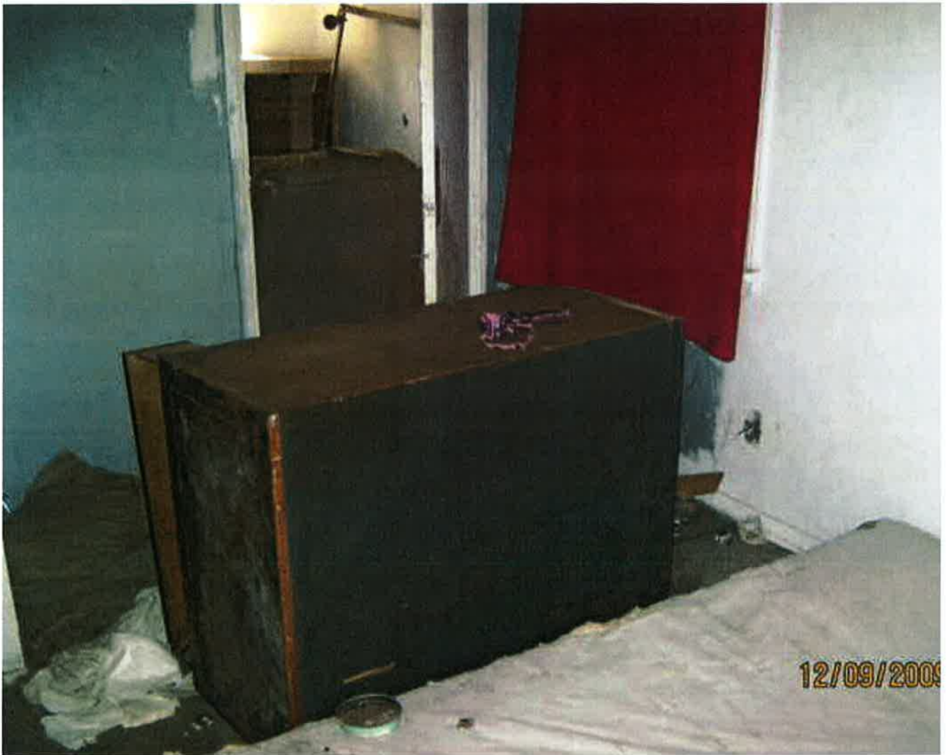
wdurant/photo of trash and debris in bedroom - 12/09/2009
