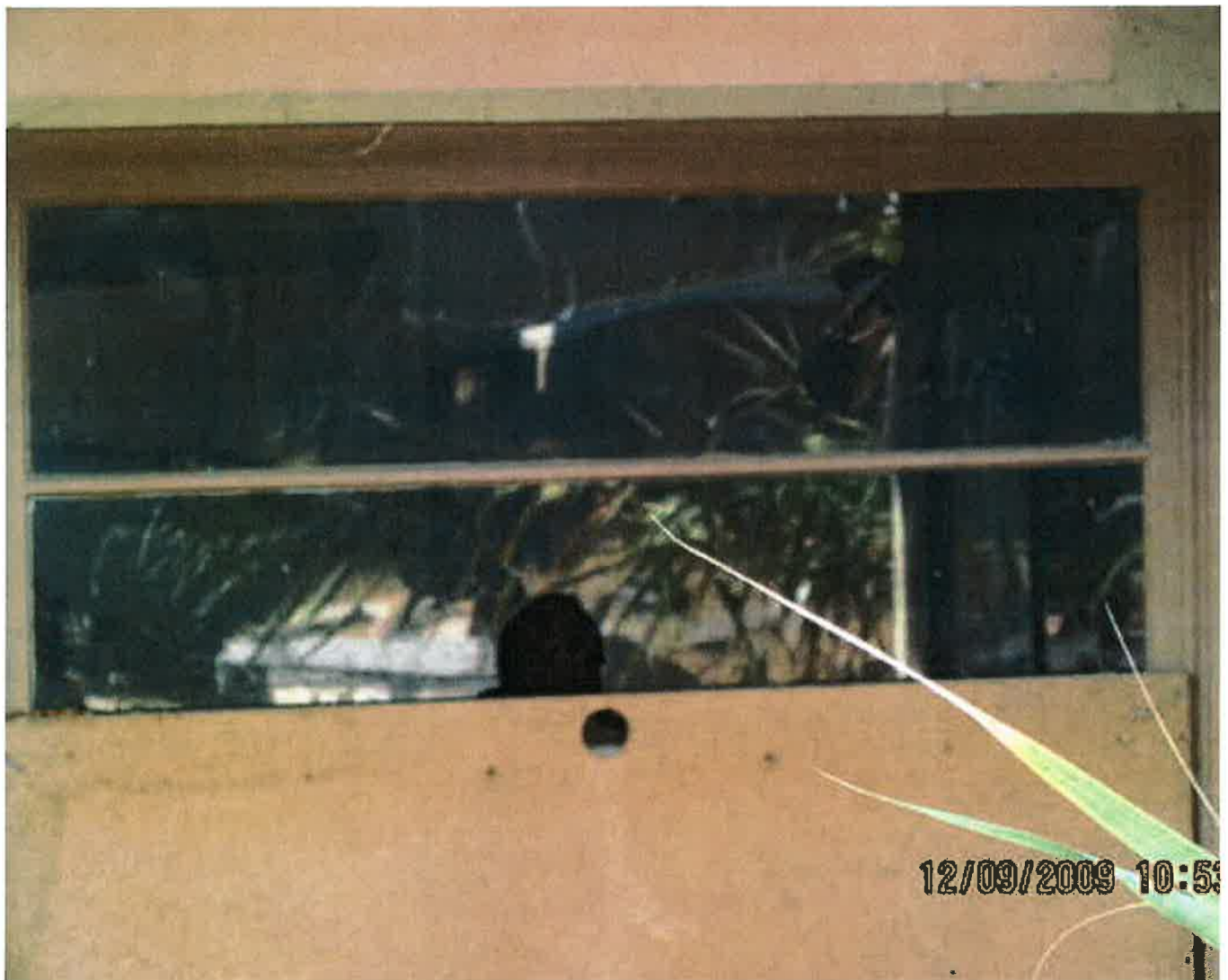
#13 Faulty weather protection. CEO Frazier, A - 12/09/2009
