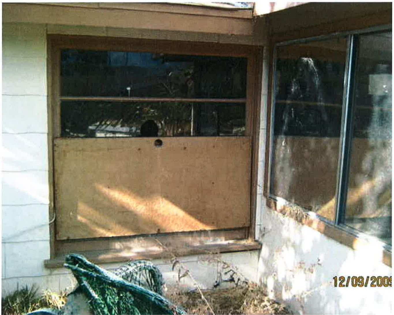
wdurant/photo of broken window glass #13 - 12/09/2009
