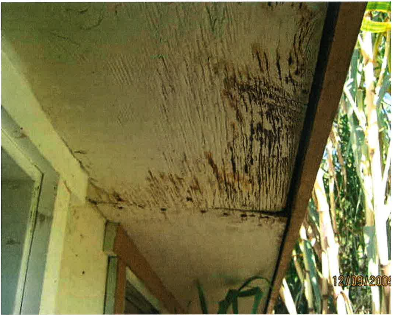
wdurant/photo of water damage and wood rot #10 - 12/09/2009
