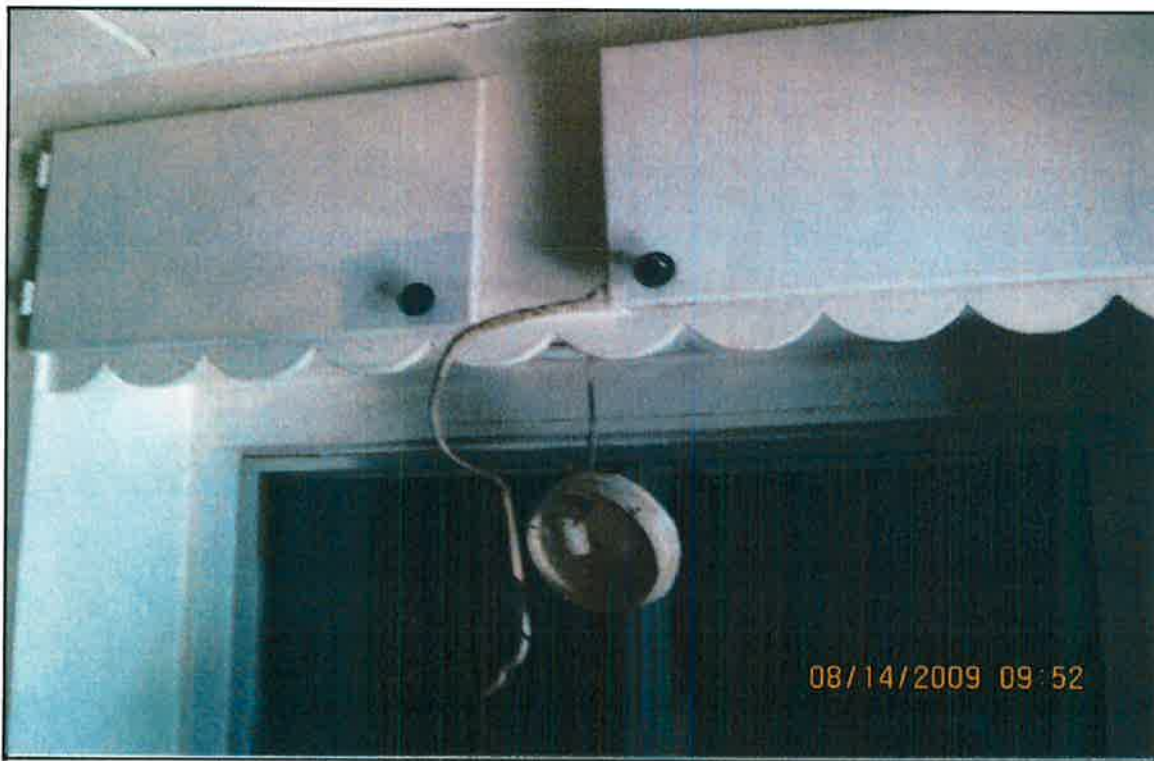
PHOTO # 2 NOTES: 6) Hazardous Wiring
