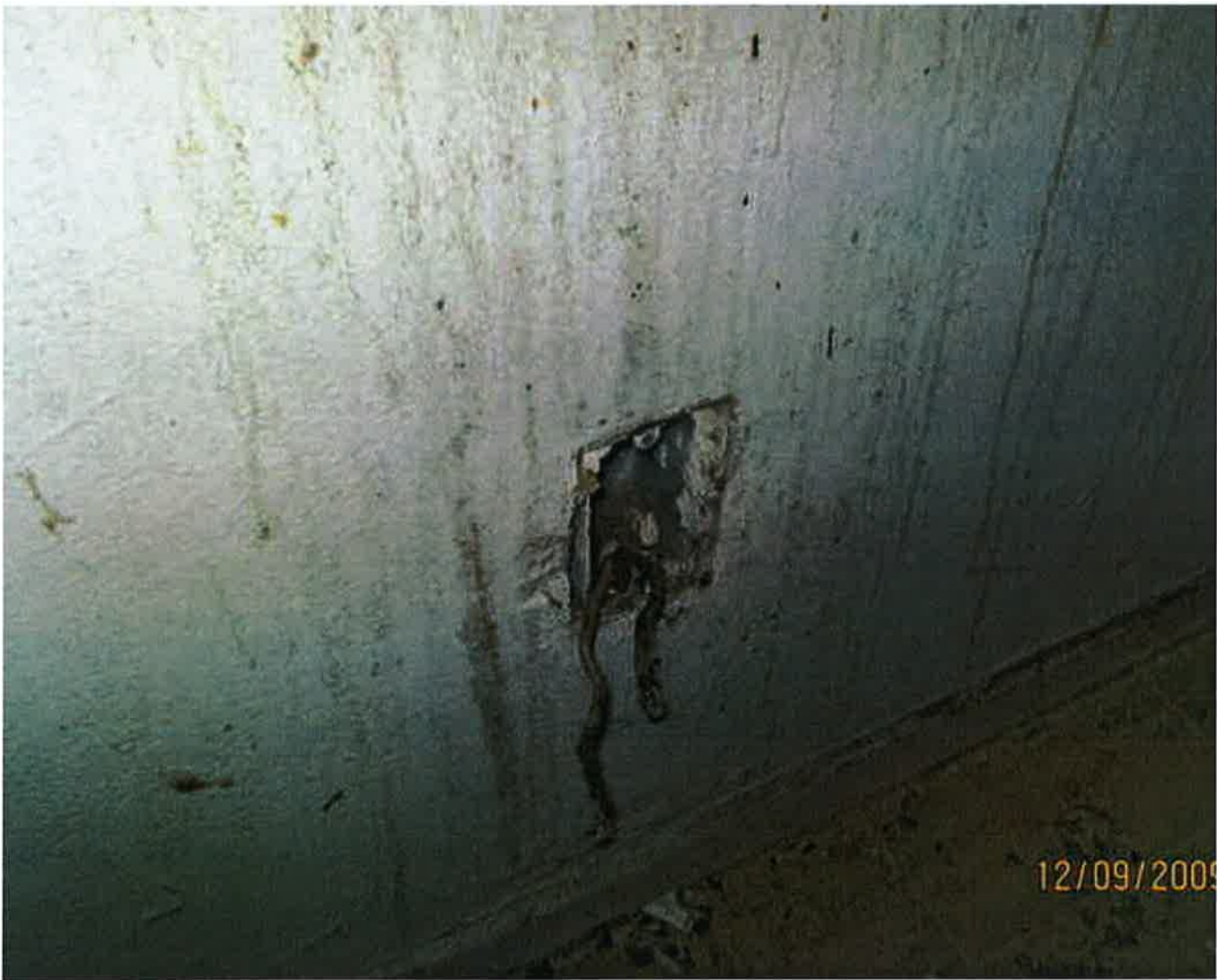
wdurant/photo of electrical wiring exposed #6 - 12/09/2009
