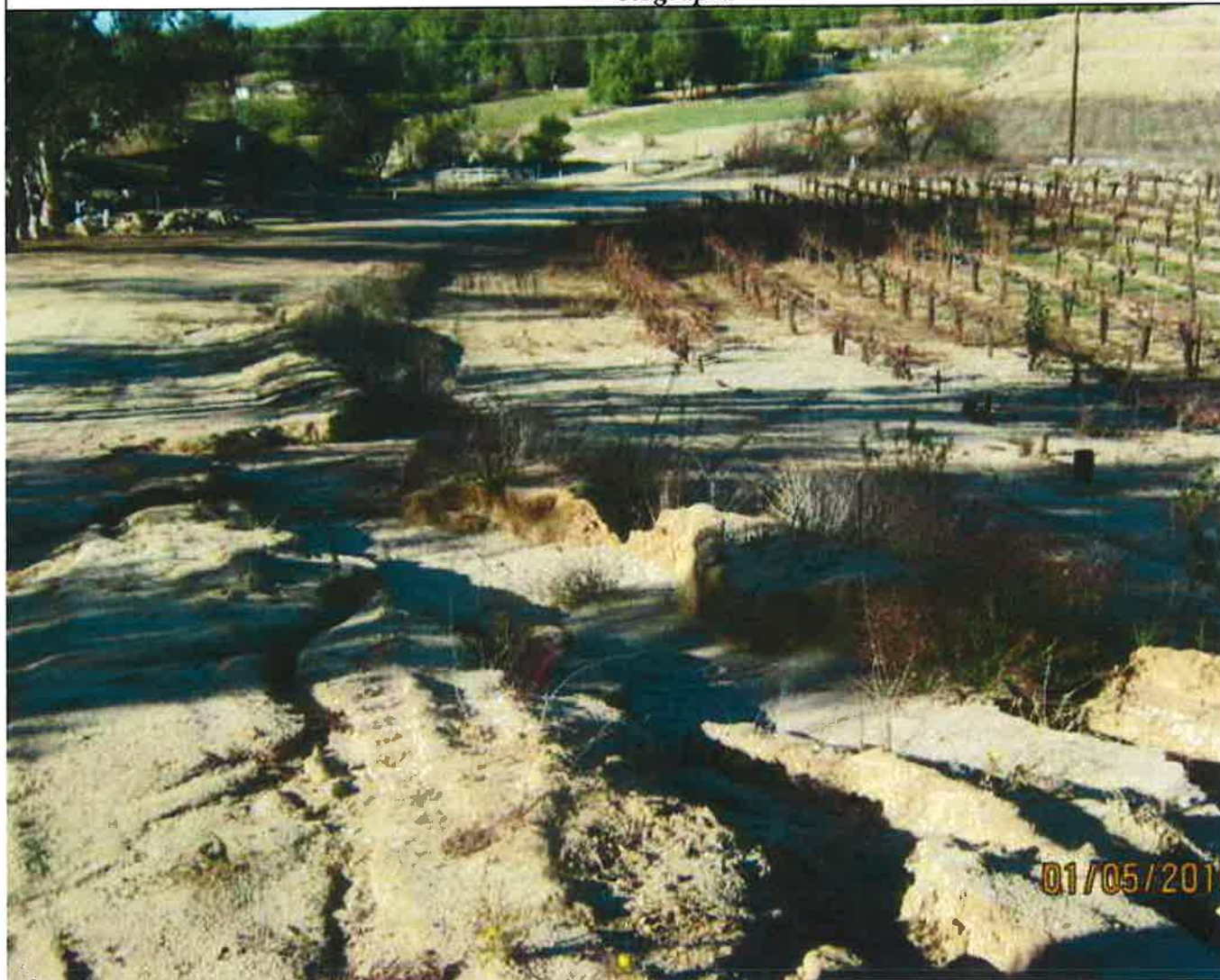
J.TATE/THELMA CIRCLE SHOWING RUTS AND THE VINEYARD DAMAGE FROM MISSING ON THIS PROPERTY - 01/05/2010
