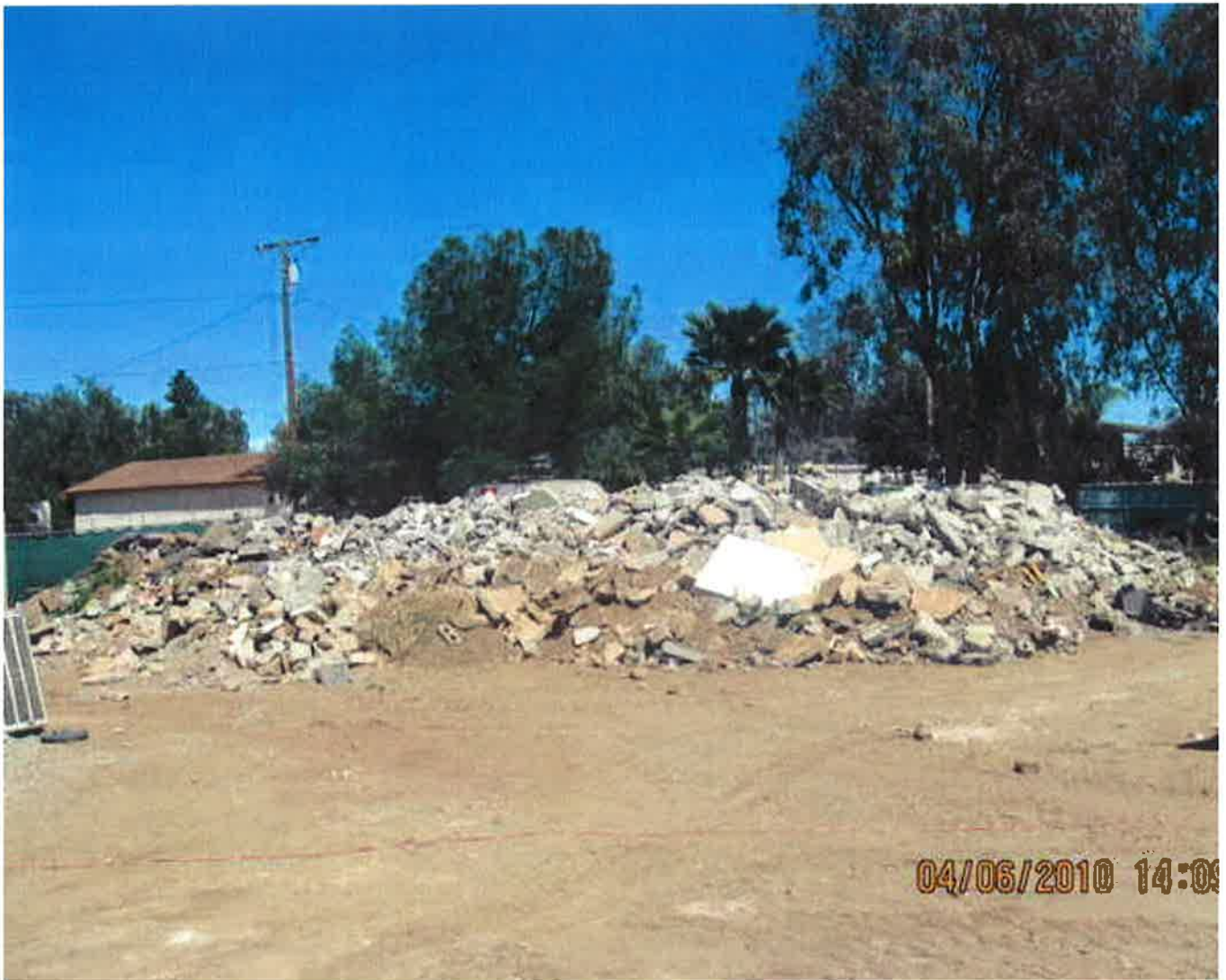
J.Wagner #80 Large pile of broken concrete. - 04/06/2010
