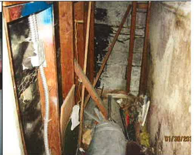
Void area between room and garage, missing drywall. RHannah NOD 13
