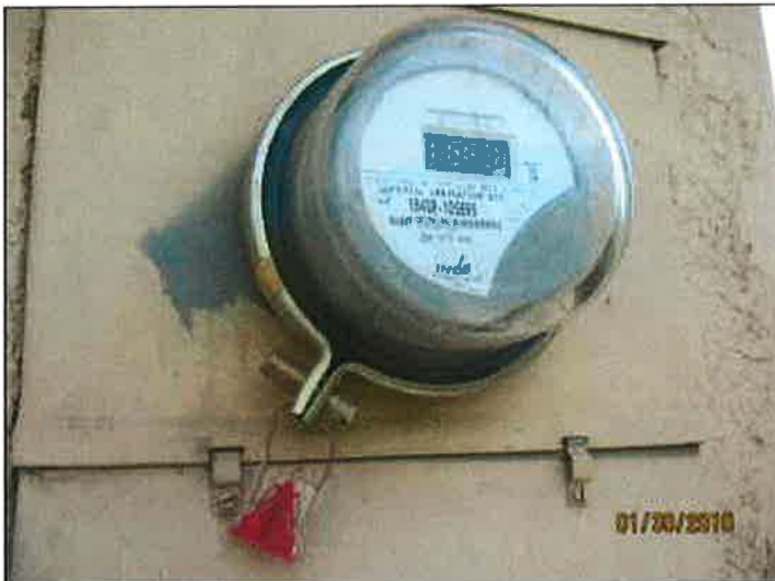
Locked out meter, no power. RHannah
