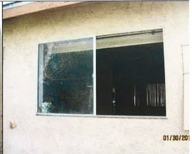
Missing window in kitchen area. RHannah NOD 13
