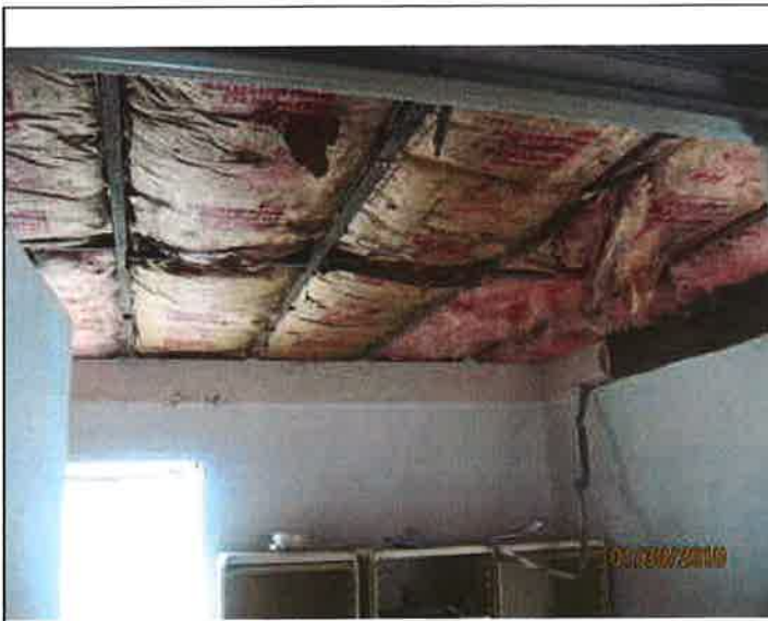
Missing drywall in garage. RHannah NOD 13
