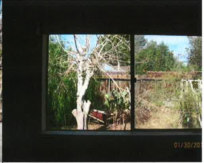
Missing rear window. RHannah NOD 13
