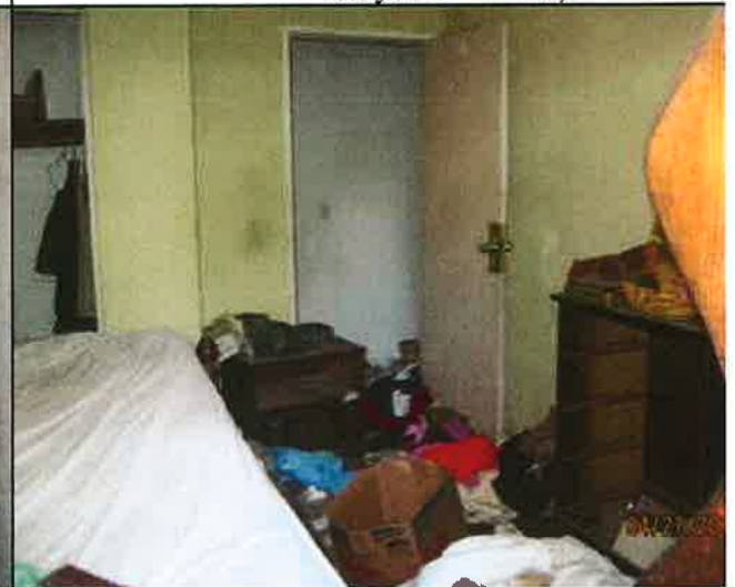
Rear bedroom, through broken window A100 13, 14,
