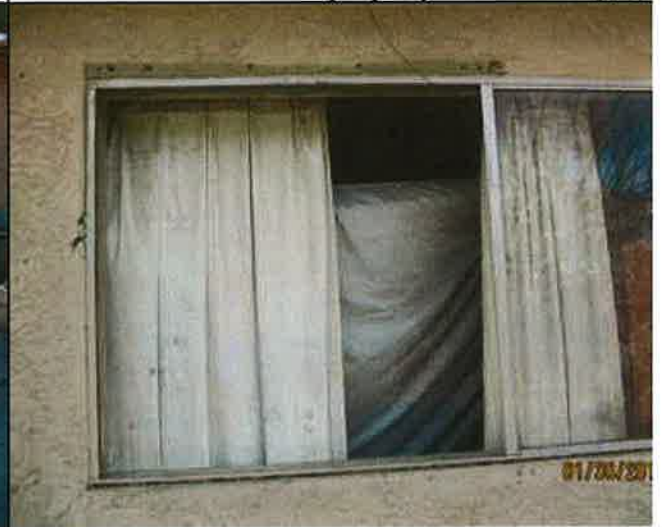
Missing bedroom window. RHannah NOD 13
